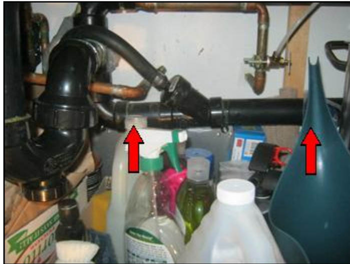
pipe slopes slightly upwards
