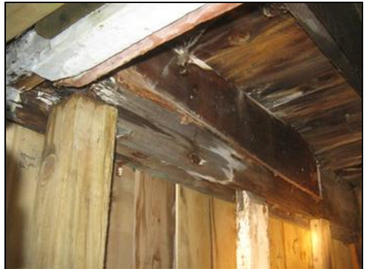
soft, rotted framing under deck
