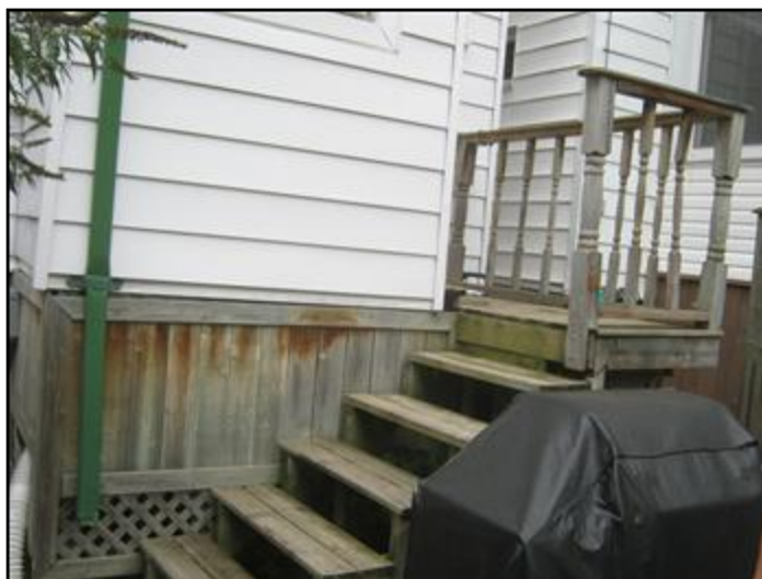
railing needed at stairs
