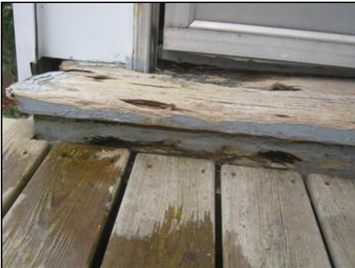
damage at threshold
