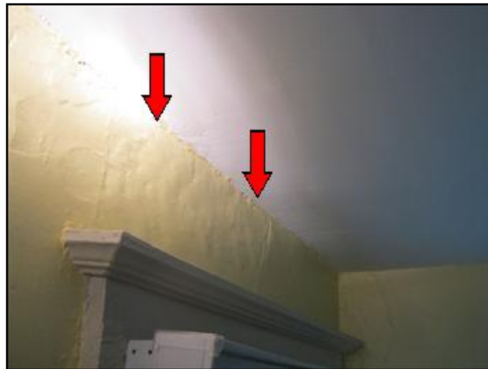
old repair noted above window
