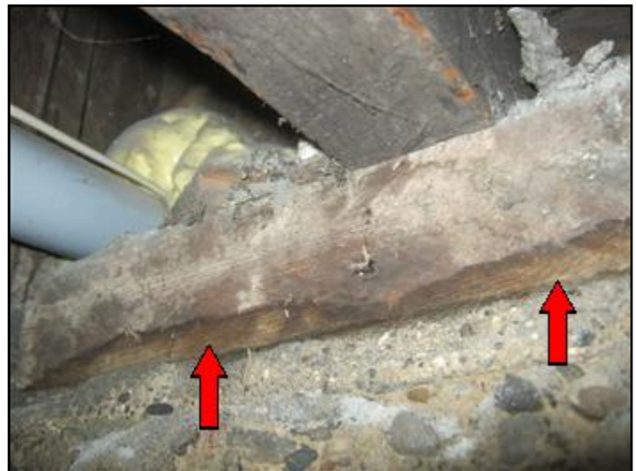
water stains under service entrance conduit
