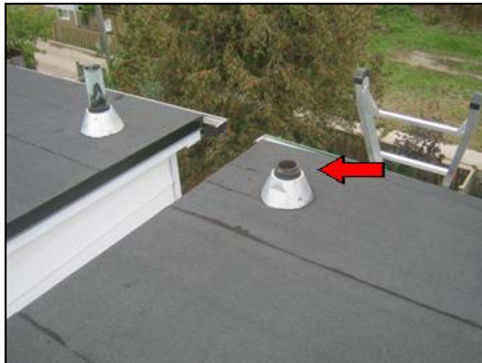
plumbing stack is short
