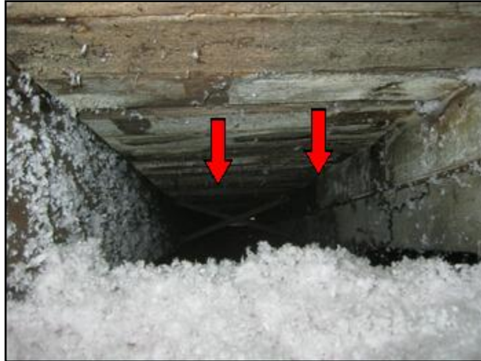
no party wall between attic spaces
