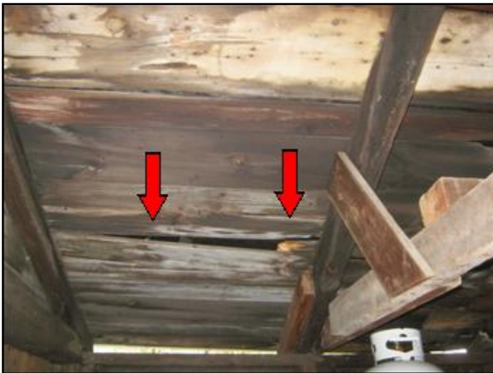
damage at garage roof sheathing
