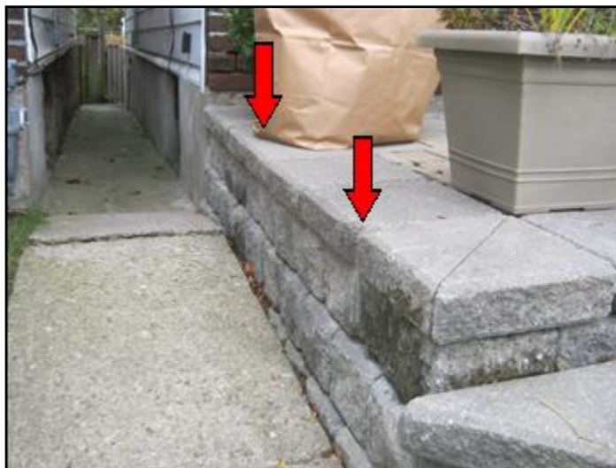
fall hazard for small children?
