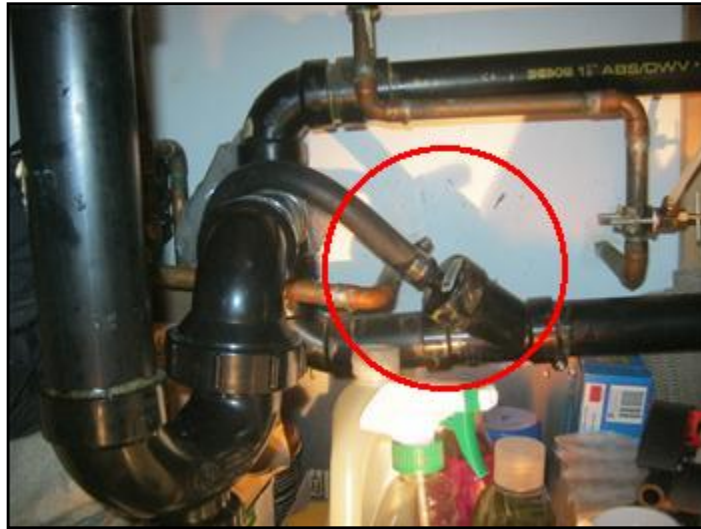
connection on wrong side of trap
