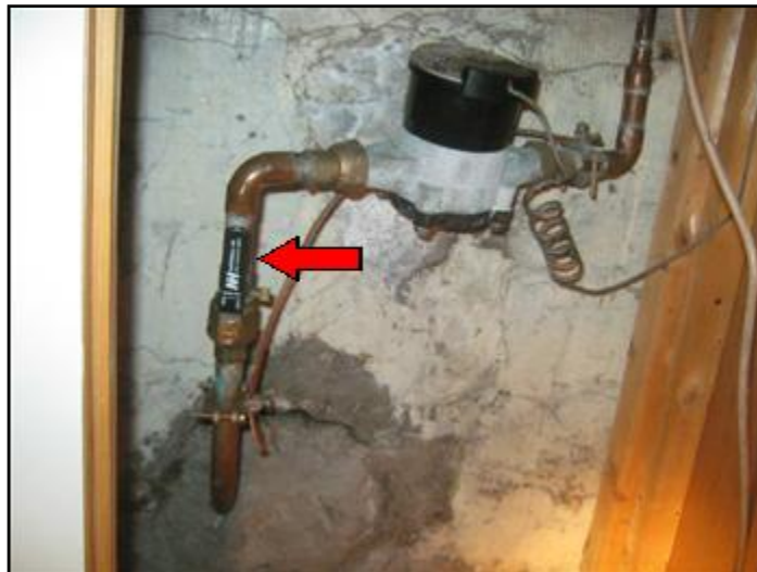
main water shut-off indicated
