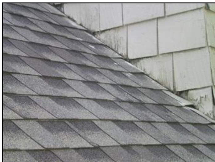
7. Cracked, split or broken
