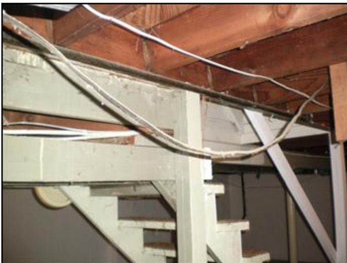
20. Not well secured
