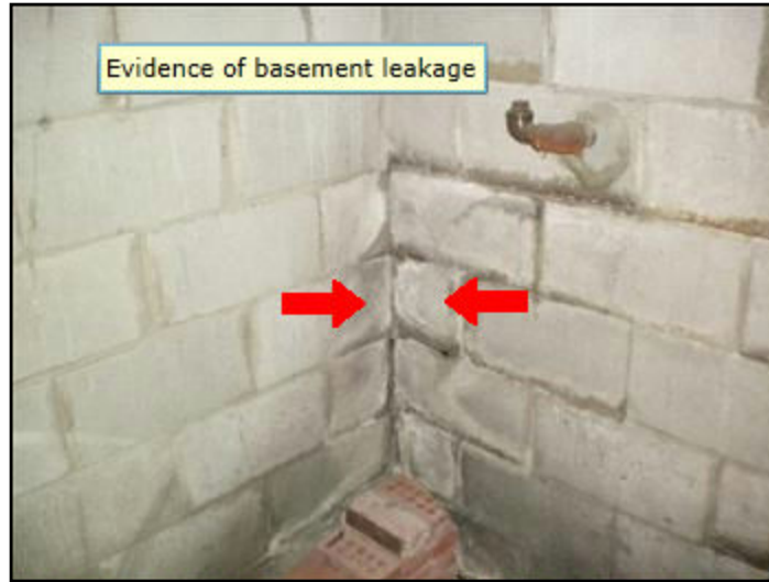
41. Leakage - See EXTERIOR section for relevant recommendations
