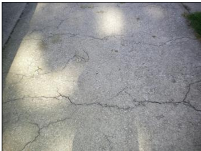
12. Cracked or damaged surfaces
