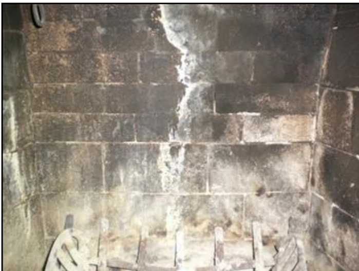
27. Inspect chimney, and sweep, if needed before using
