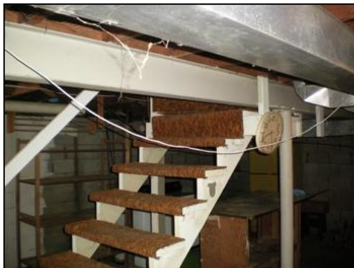
24. Not well secured
