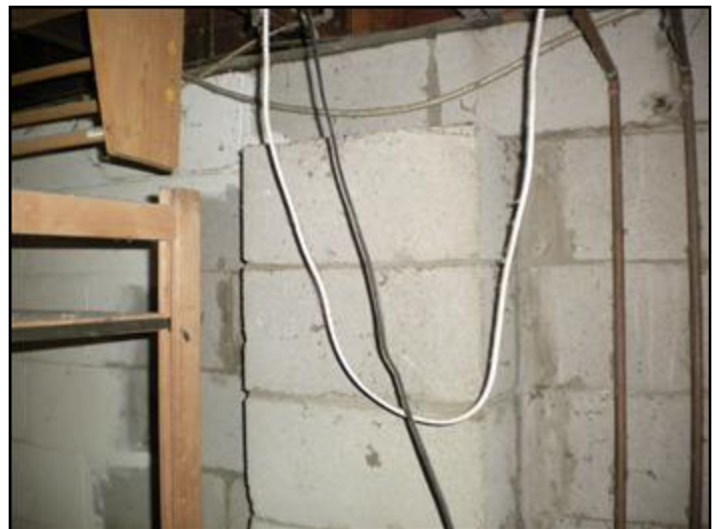
21. Not well secured
