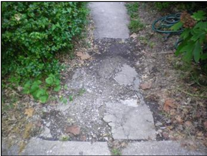
13. Improper slope or drainage
