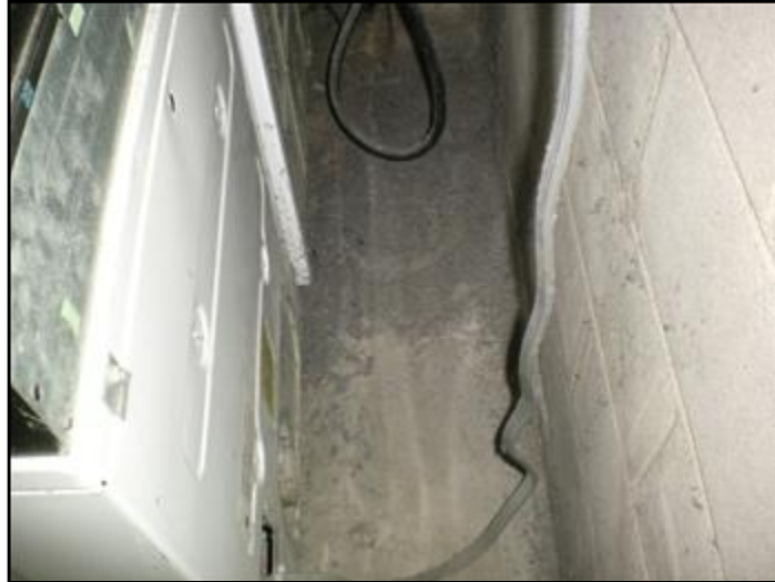
43. Not vented to exterior
