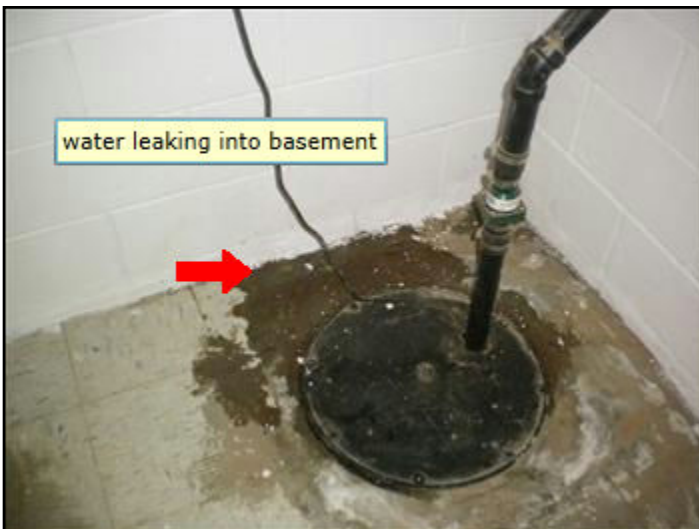
39. Leakage - See EXTERIOR section for relevant recommendations
