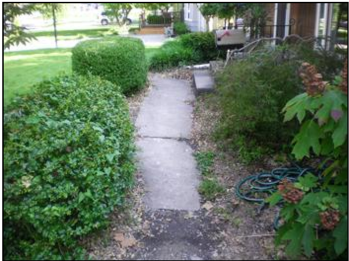
14. Improper slope or drainage
