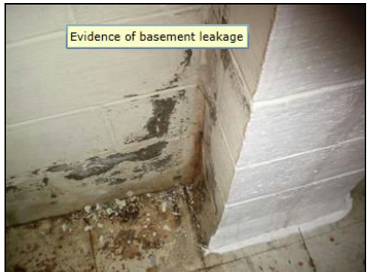
40. Leakage - See EXTERIOR section for relevant recommendations
