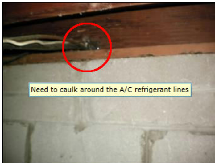
6. Caulking missing or ineffective
