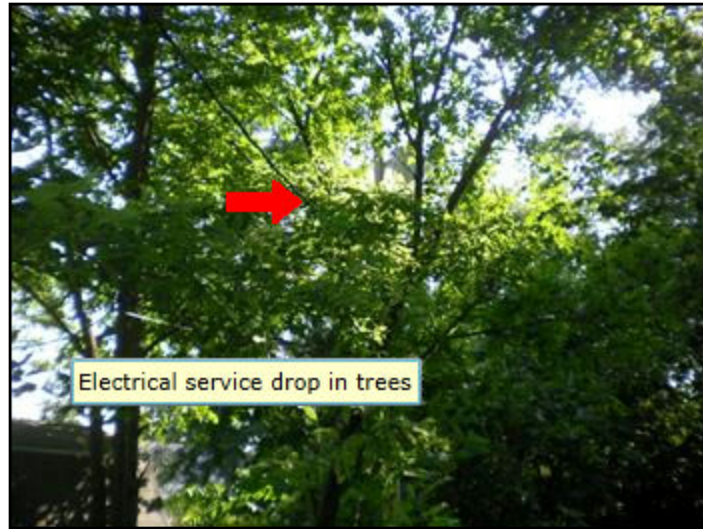
15. Branches, vines interfering with wires
