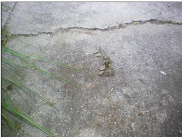
11. Cracked or damaged surfaces
