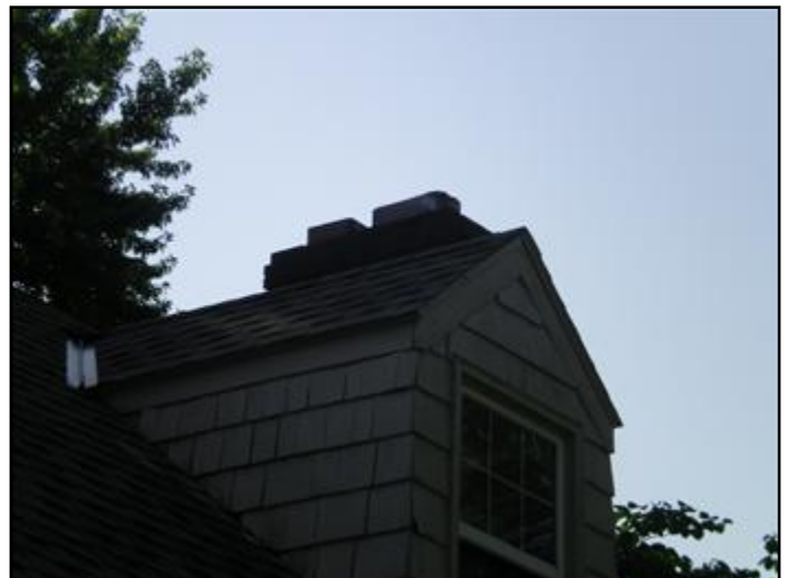
28. Inspect chimney, and sweep, if needed before using
