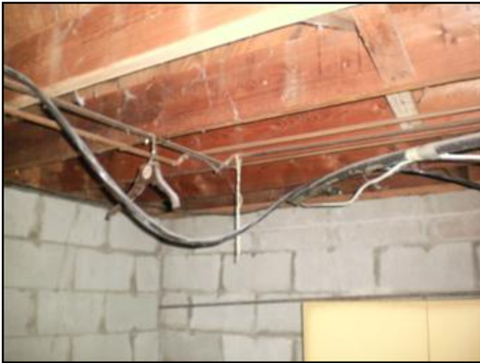
22. Not well secured
