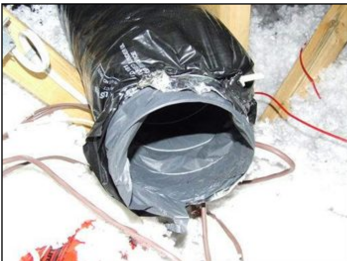
17. loose telephone wires and exhaust fan
