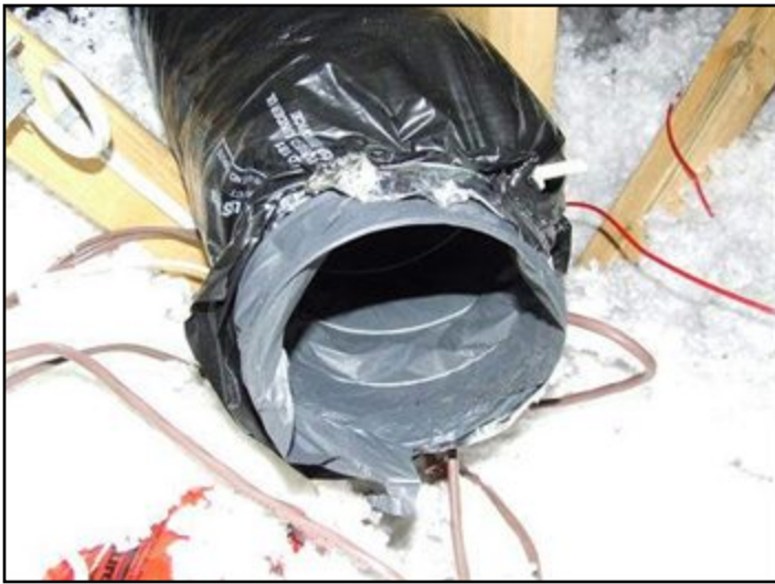
39. loose telephone wires and exhaust fan
