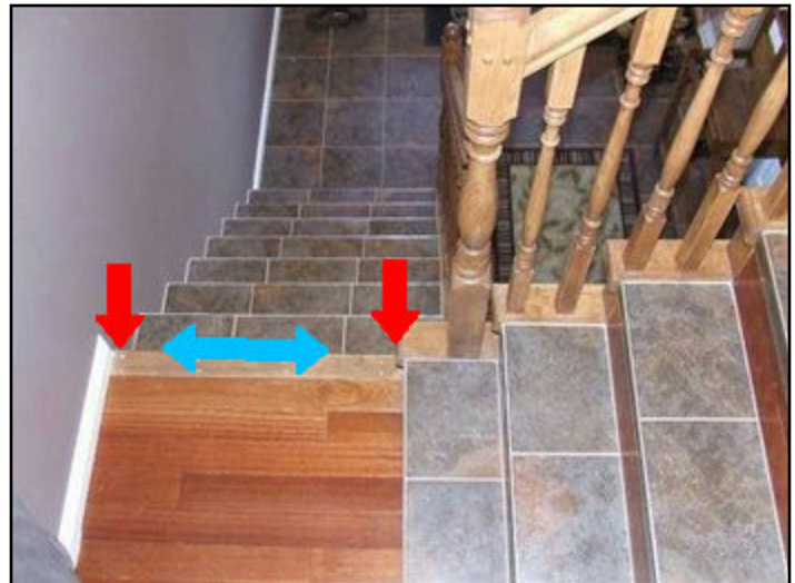
16. Landing is 32 inches wide, should be 36
