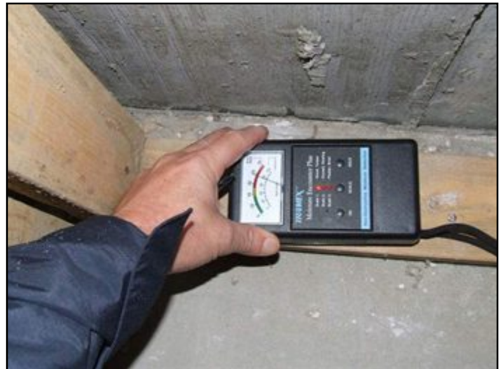
26. Excessive moisture reading on interior wall f
