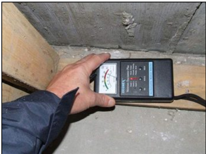
4. Excessive moisture reading on interior wall f
