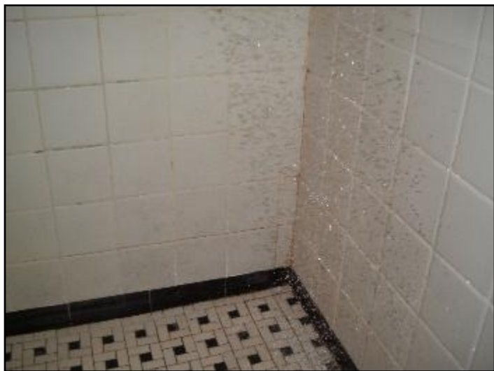
7. Grout broken and deteriorated
