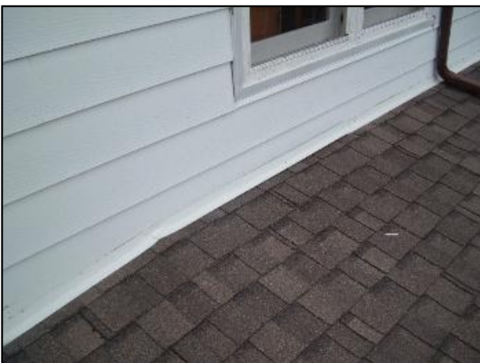
1. improper installation/open at top
