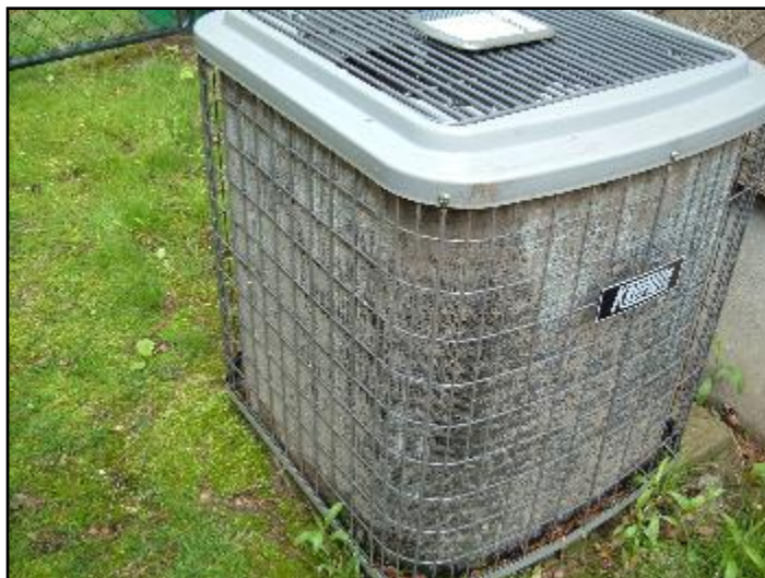
6. Clean condensing unit immediately
