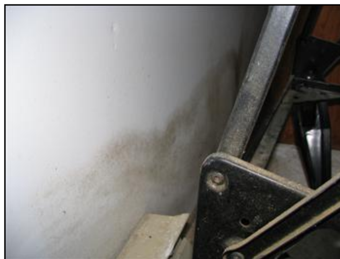
16. Efflorescence and staining
