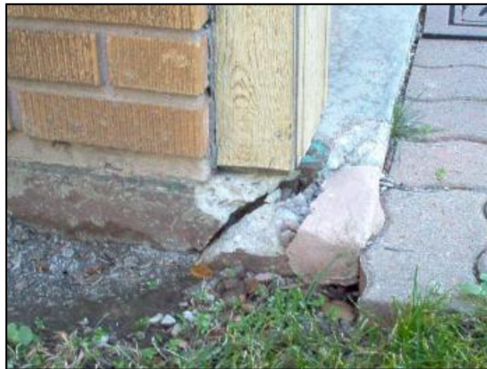
8. Concrete damage at front entrance.
