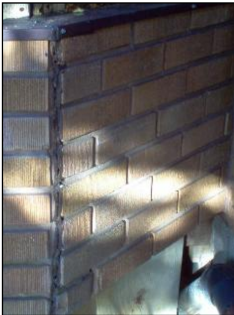
5. Crack along mortar joint at bay window.
