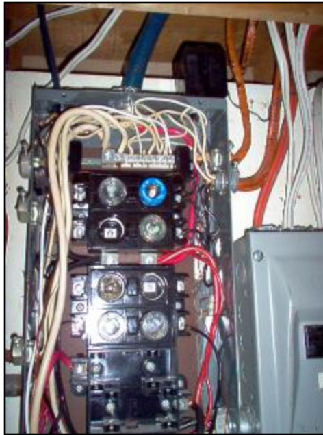
9. Missing fuses in auxiliary panel.
