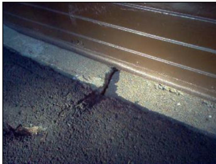
6. Poor slope at driveway/garage slab.
