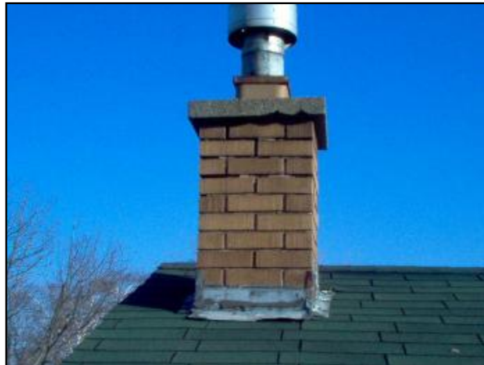
3. Damaged chimney flashing.
