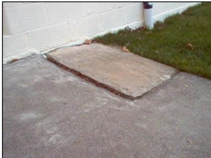
7. Trip hazard at rear patio.
