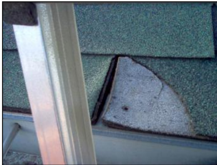
1. Broken shingle, exposed sheathing.
