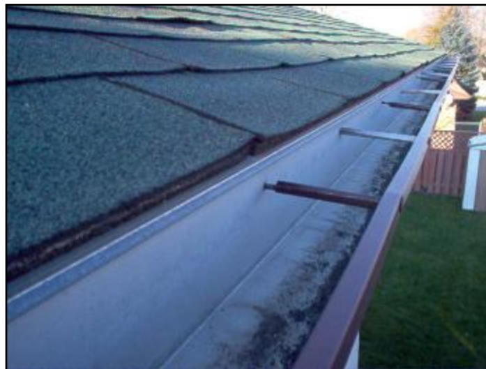
2. Shingles not extended into trough.
