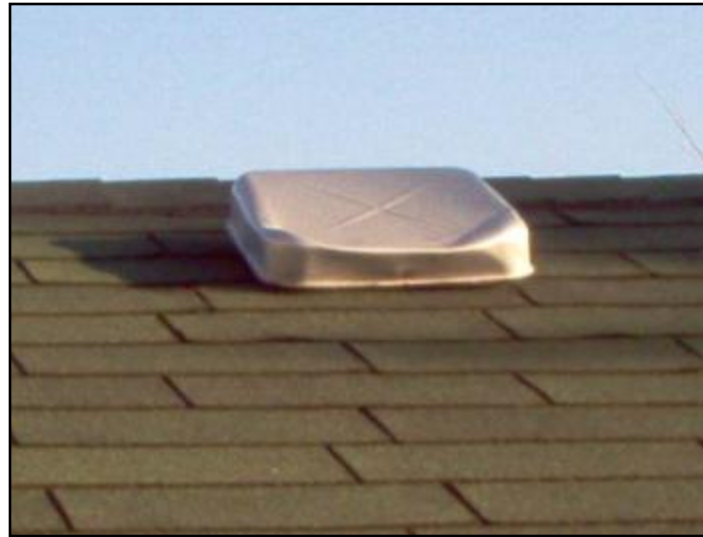
10. Damaged roof vent.
