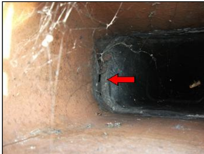
10. Opening and Crack in Flue
