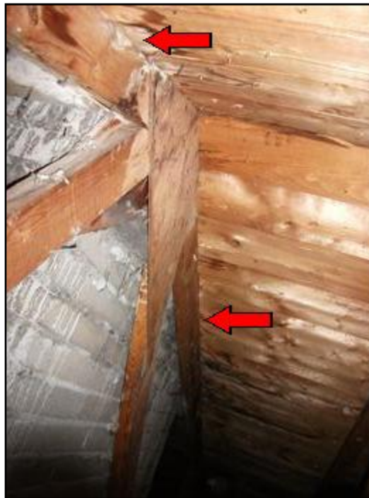
1. Signs of Past Leak
