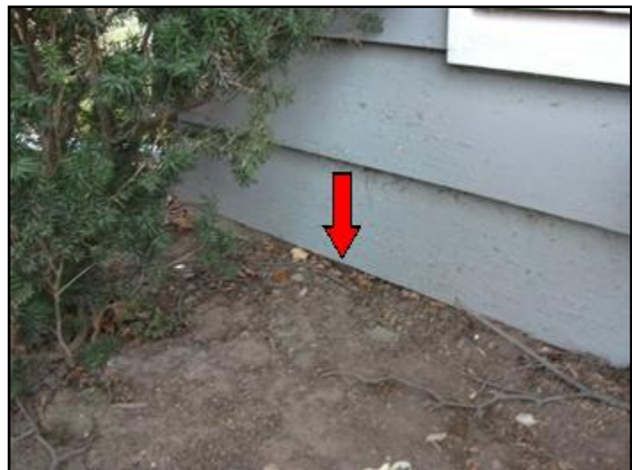
4. Wood Siding in Contact With Ground
