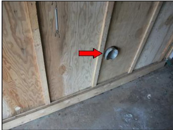
19. Dryer Vent Termination in Garage
