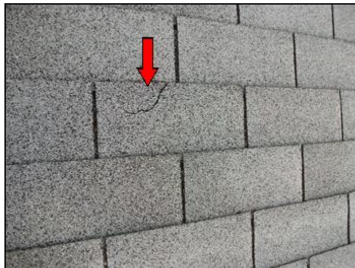
2. Roof Shingle Cracked
