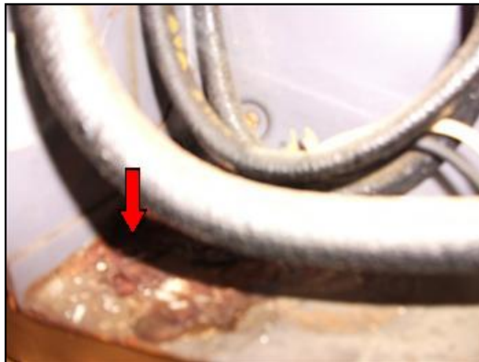
5. Rust in Panel
