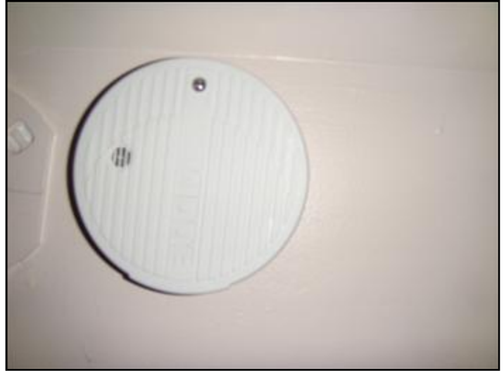
5. not working 2nd floor
