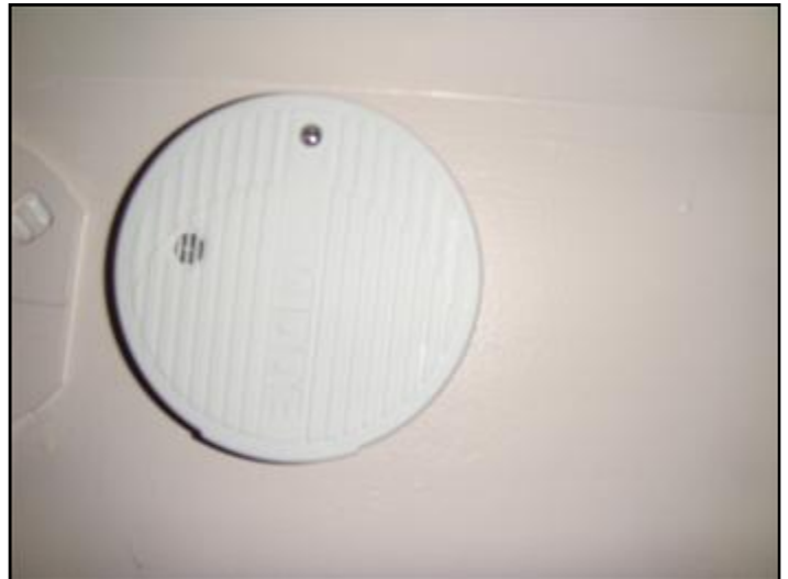
16. not working 2nd floor
