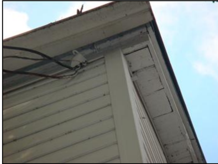
2. cable covered with siding
