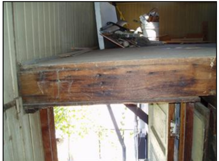
4. SAG LEANING FLOOR
