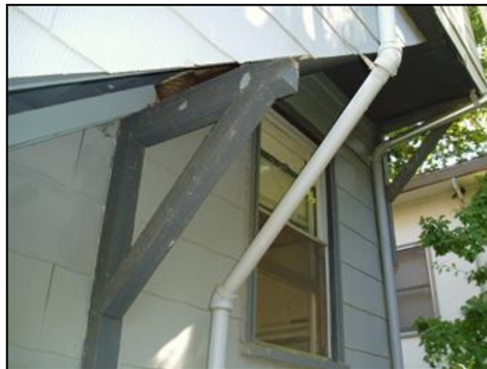
5. POOR SUPPORT OF ATTIC AREA
