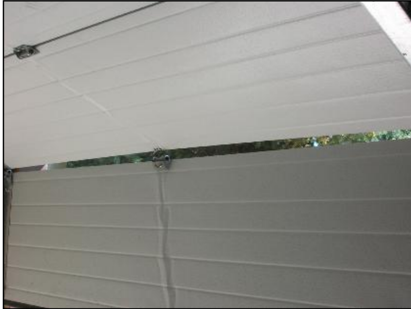
12. Mechanical damage to garage door
