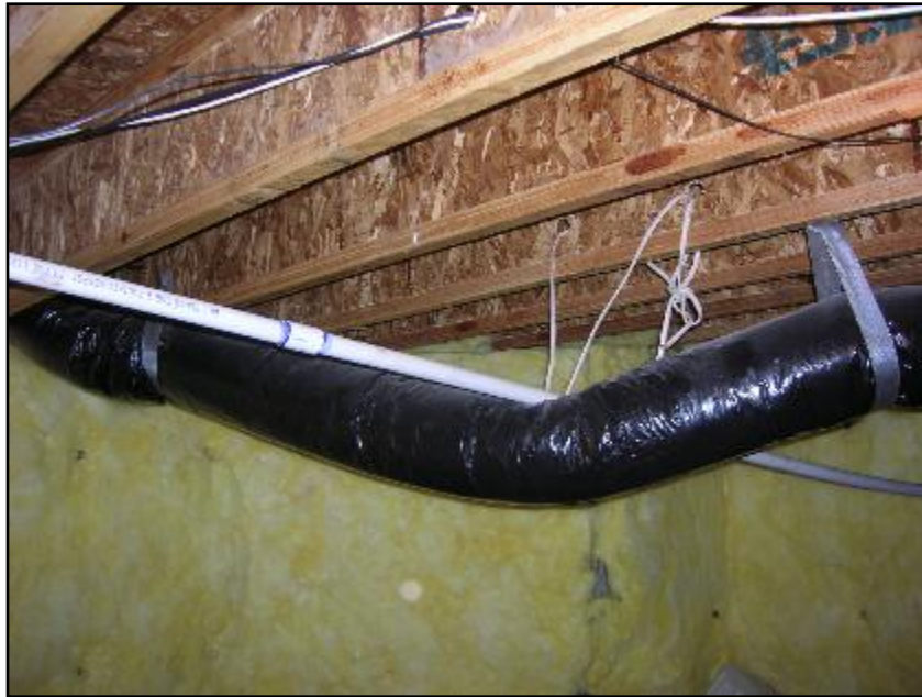
9. Poor support for PVC water line
