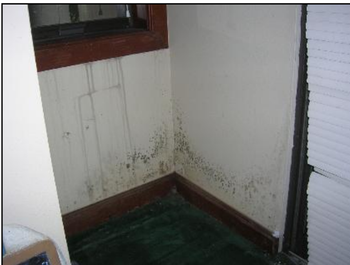
10. Water damage with mold on drywall
