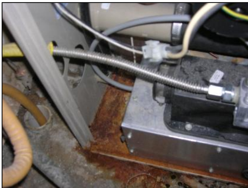
5. Rust in furnace
