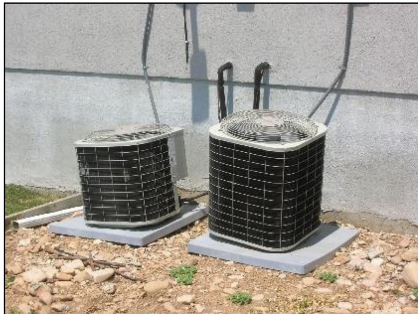
6. Compressors out of level
