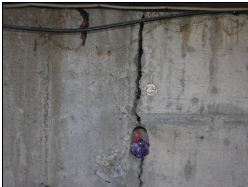
3. Crack in foundation
