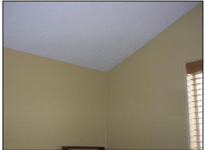
8. Area of missing insulation
