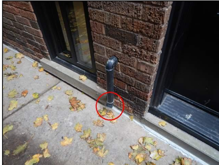
Discharge pipe problems
