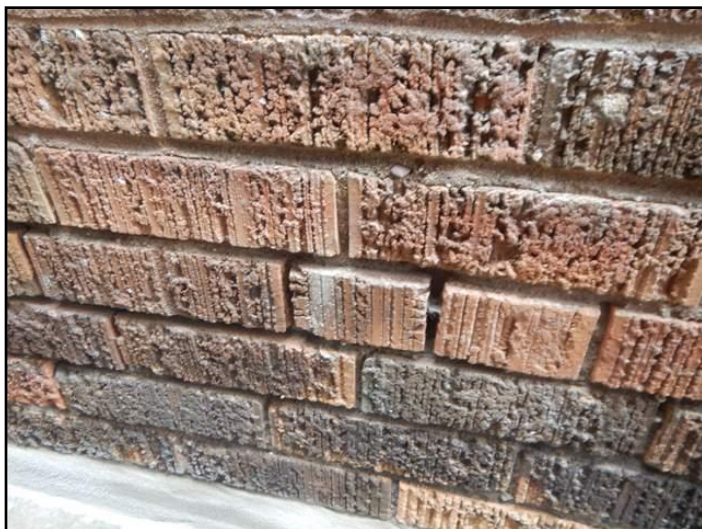
Example - Mortar deteriorating
