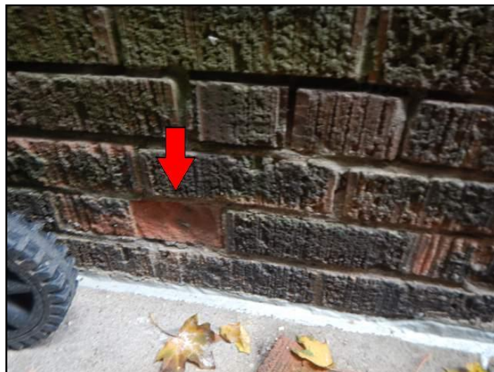
Example - Spalled brick
