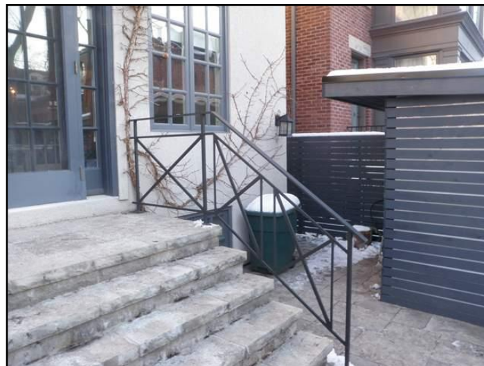
Large openings at railings
