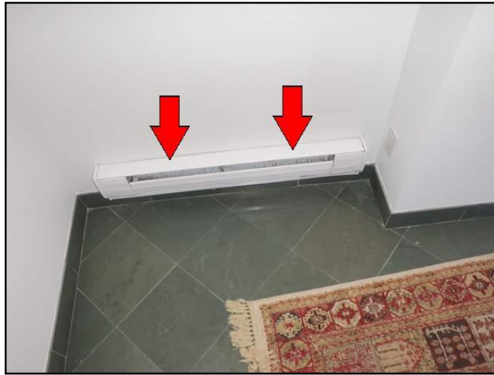
Electric baseboard heater (foyer)
