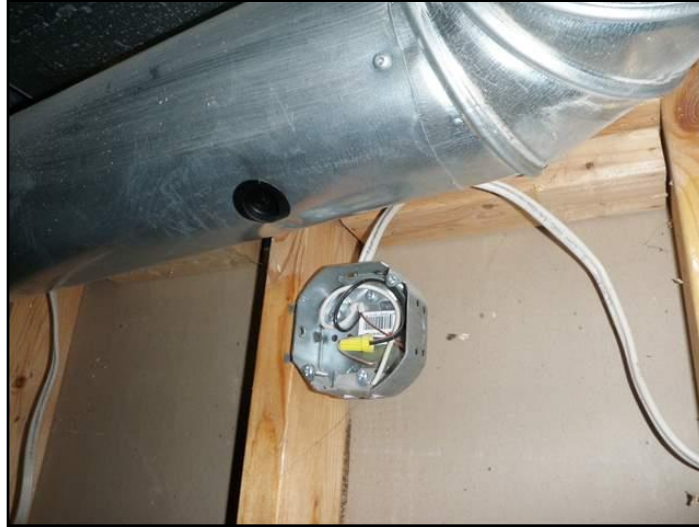
Cover missing at junction box
