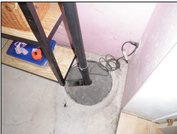
Sump pump- rear cold room
