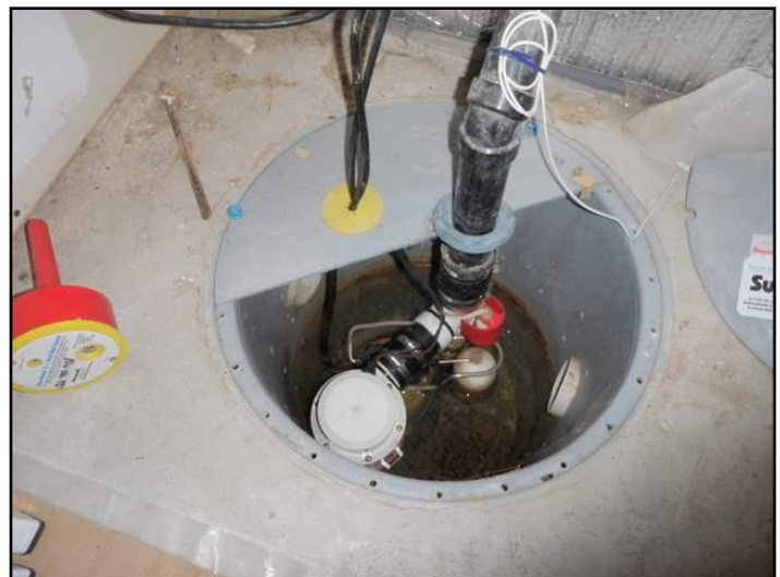
Sump pump- west basement
