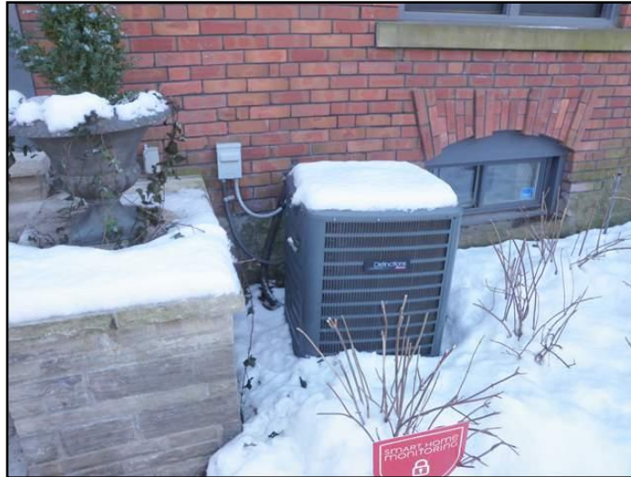
Air cooled- outdoor unit at front yard
