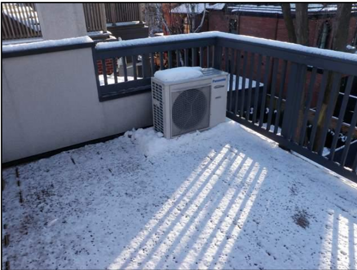
Ductless (Mini split) system- outdoor unit
