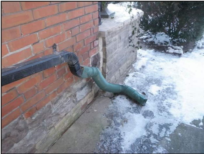
Discharge too close to building
