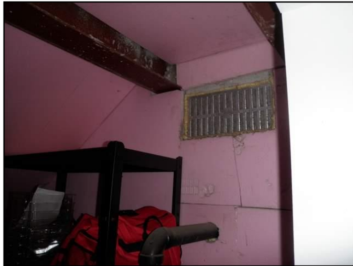
Combustible insulation exposed
