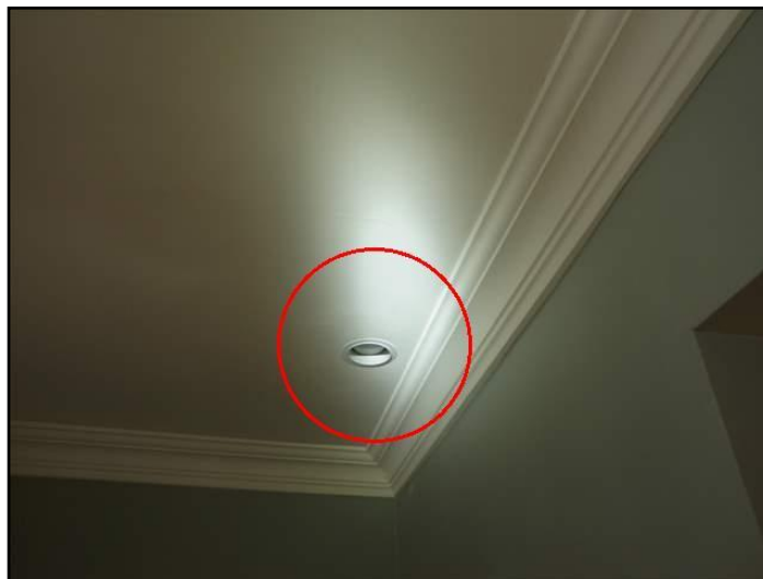
Patched ceiling under rear ensuite
