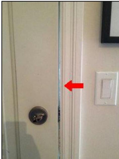
Weatherstripping missing or ineffective
