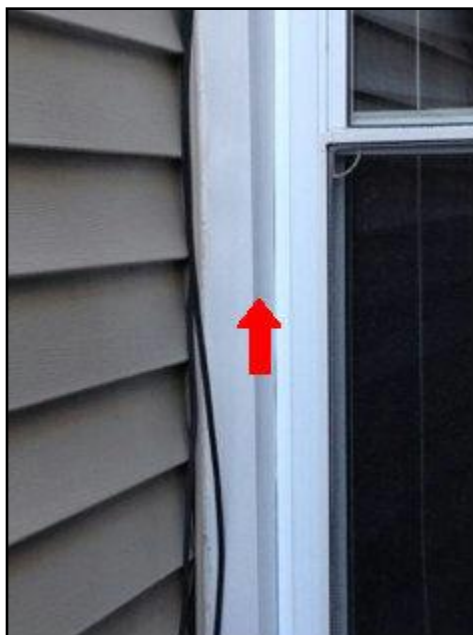
Caulking missing, loose or deteriorated
