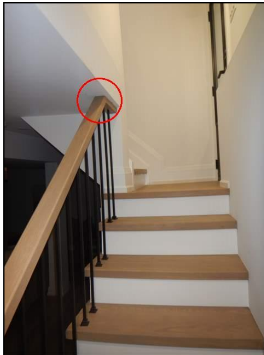
Incomplete or not continuous railing
