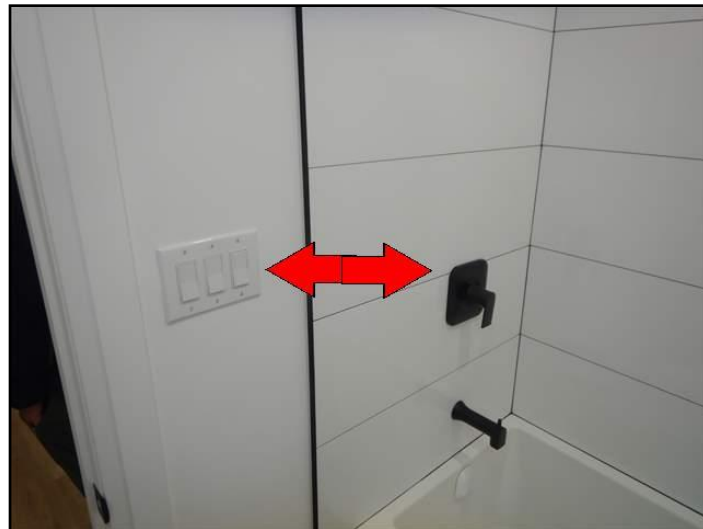
Location poor (near Bathtub or Shower Stall)
