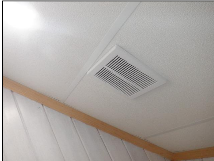
72. Bathroom exhaust fan
