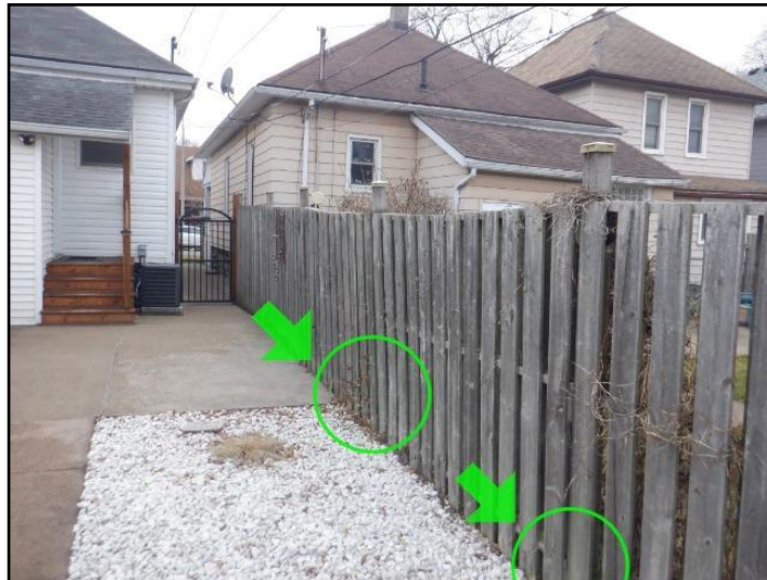
19. Few broken fence posts
