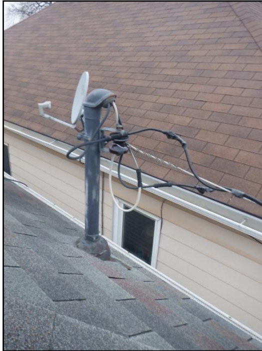
39. Overhead - cable type not determined
