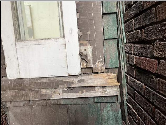
3. Cracked, split or broken
