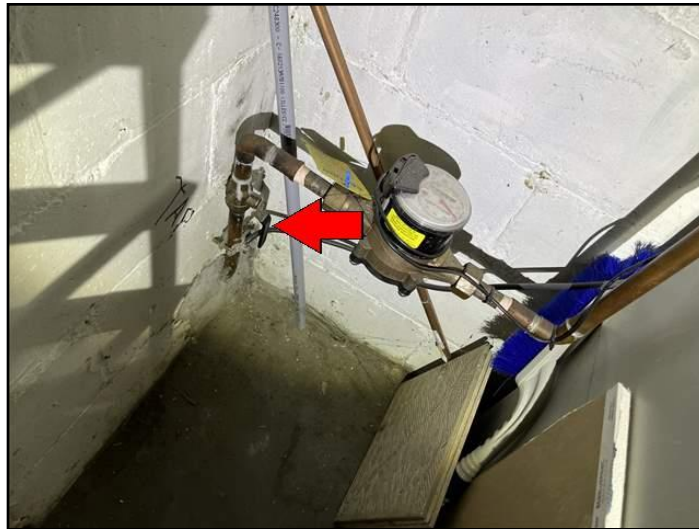
12. Main water shut off valve
