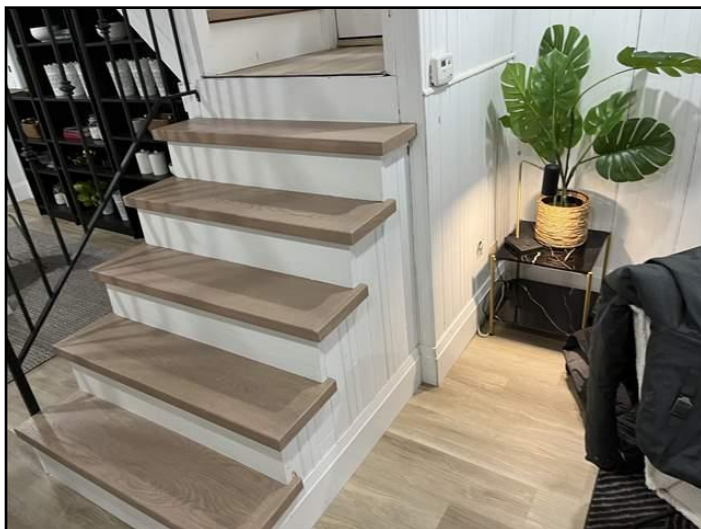
17. Missing on open side
