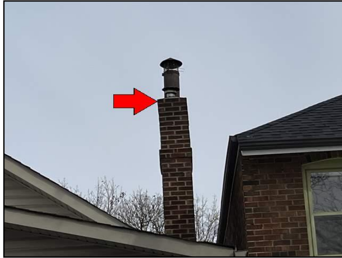
9. No drip edge on cap (crown)
