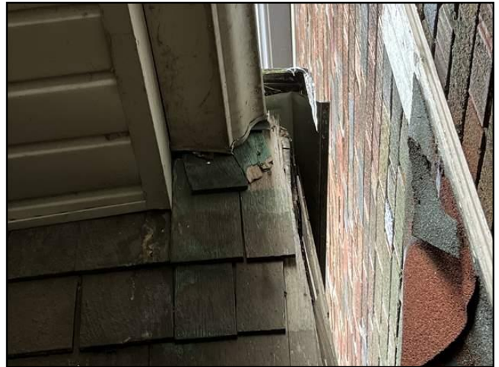
4. Cracked, split or broken
