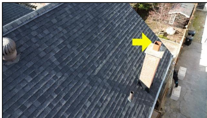
13. Rain cap missing or damaged
