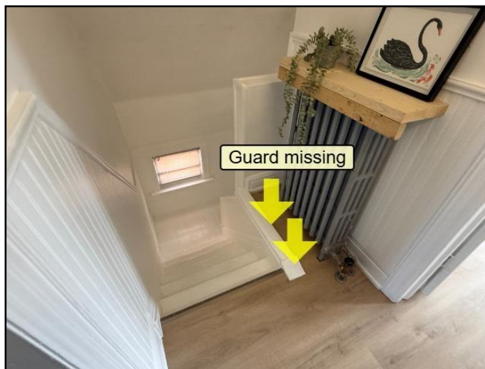
15. Missing Guard and handrails
