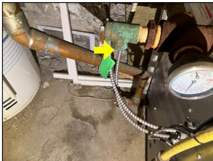
11. No pipe extension
