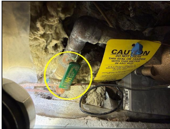
14. Main water shut off valve - Front of the...
