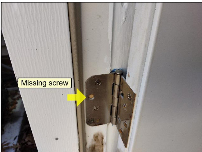
Missing or damaged
