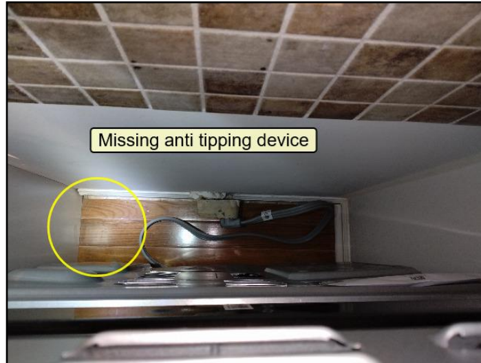
Anti-tipping device missing
