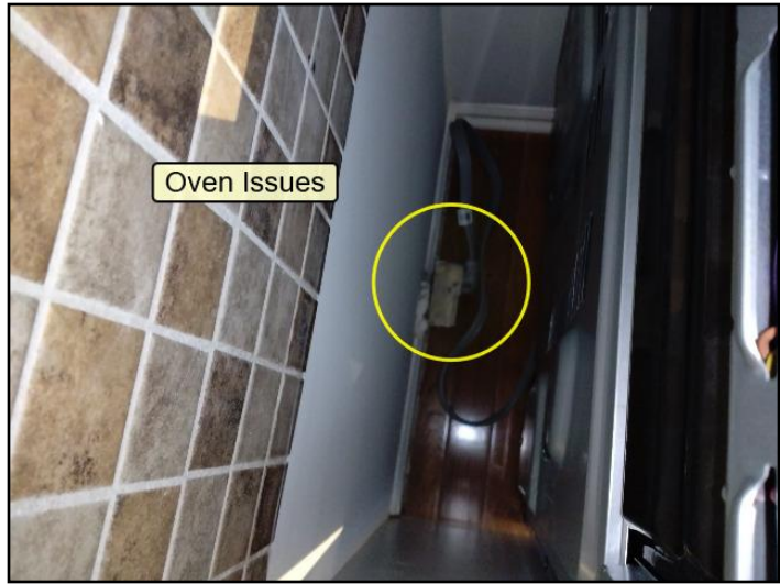
Loose Electrical Connection
