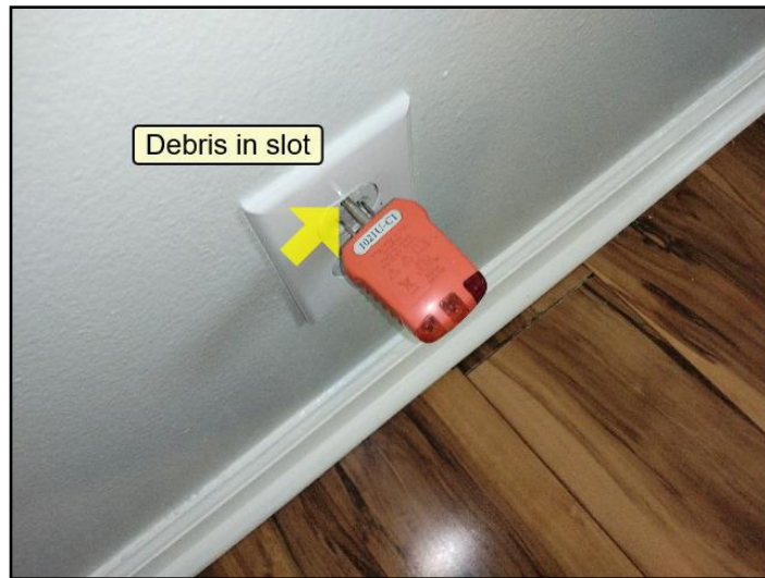
Obstructed by paint
