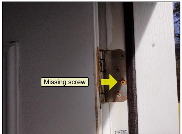
Missing or damaged
