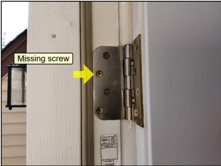
Missing or damaged
