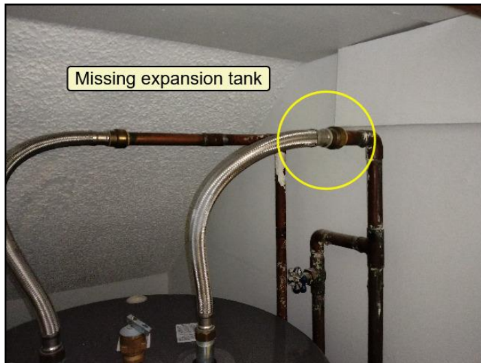
Expansion tank missing
