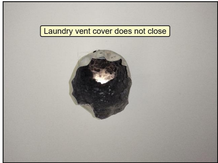
Cover does not close properly
