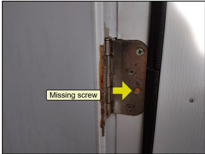
Missing or damaged
