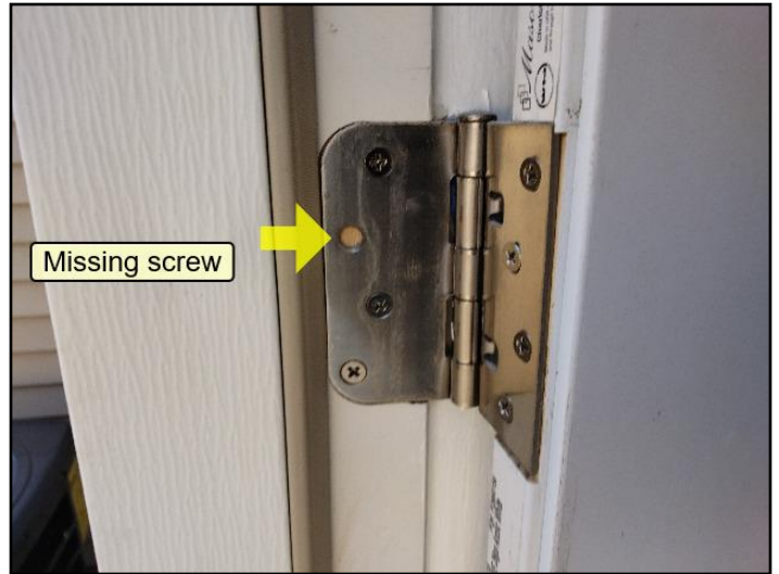
Missing or damaged
