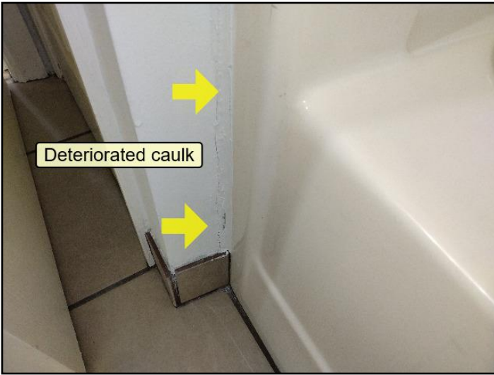
Caulking loose, missing or deteriorated
