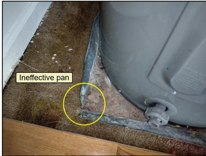
Safety pan and drain defect
