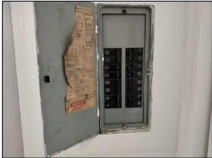
Breakers - first floor
