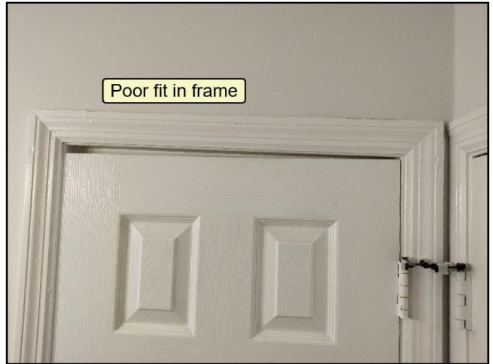
Loose or poor fit
