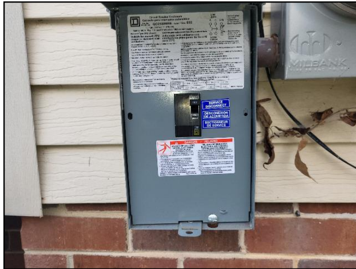
Breakers - exterior wall
