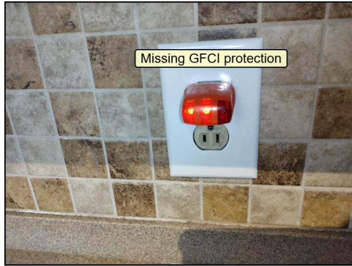
GFCI/GFI needed (Ground Fault Circuit...
