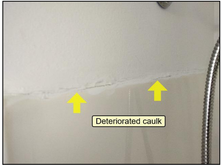
Caulking loose, missing or deteriorated
