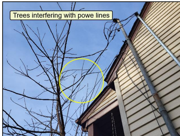
Branches / vines interfering with wires
