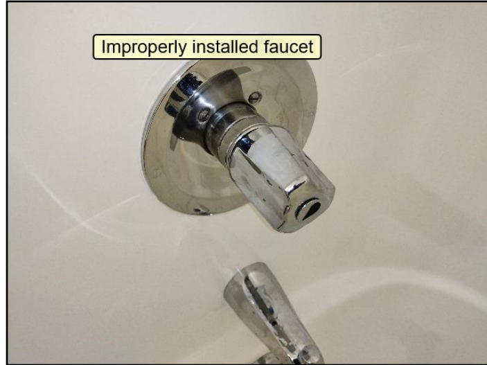
Hot and cold faucets not identified clearly
