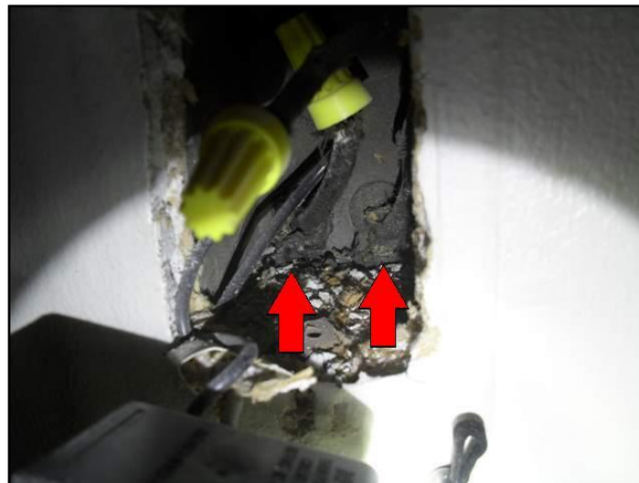
Switch at front door
