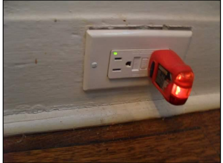
Ungrounded, sideways mounted outlet.
