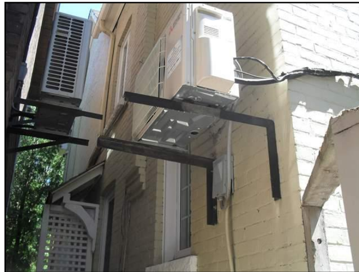
Ductless (Mini split) system
