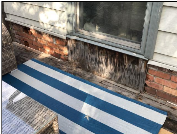
Masonry and mortar - incomplete/missing...
