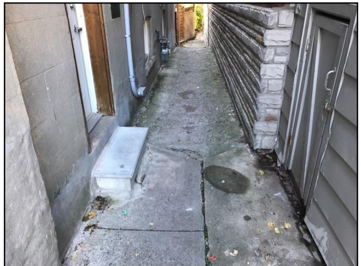
Improper slope or drainage
