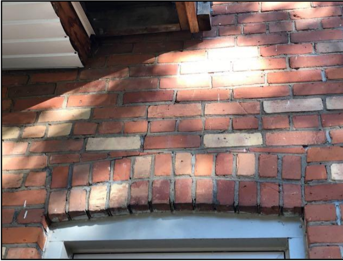
Typical minor cracks
