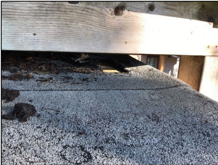
Damage, punctures, tears
