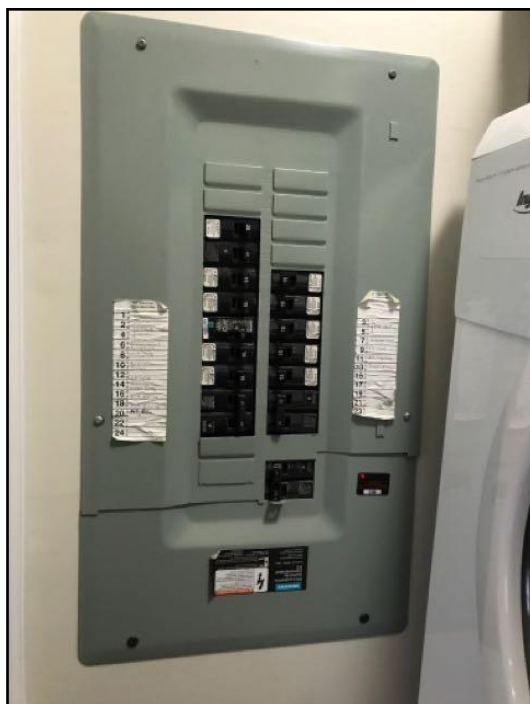
Breakers - Rear first floor
