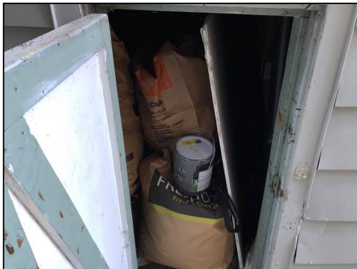
Access door - damage, loose
