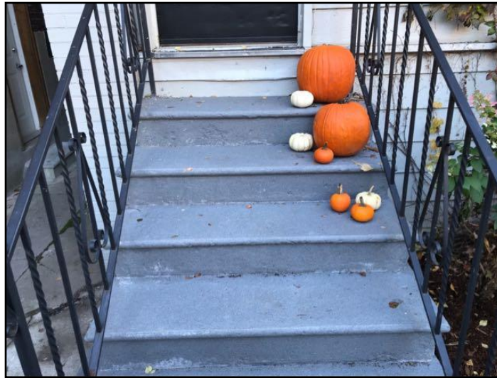
Landing - too small/missing
