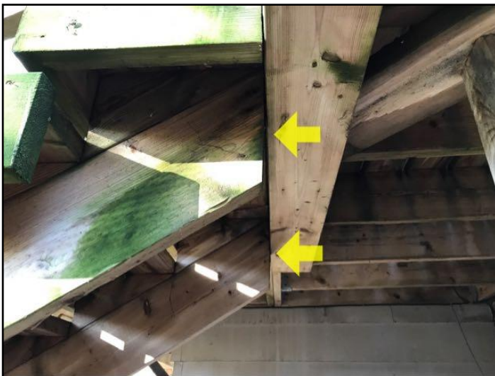
Connections weak, not level
