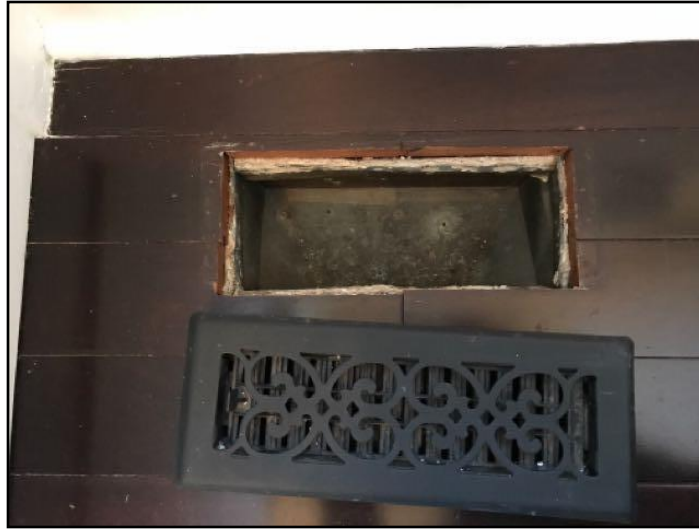
Duct insulation - may contain asbestos
