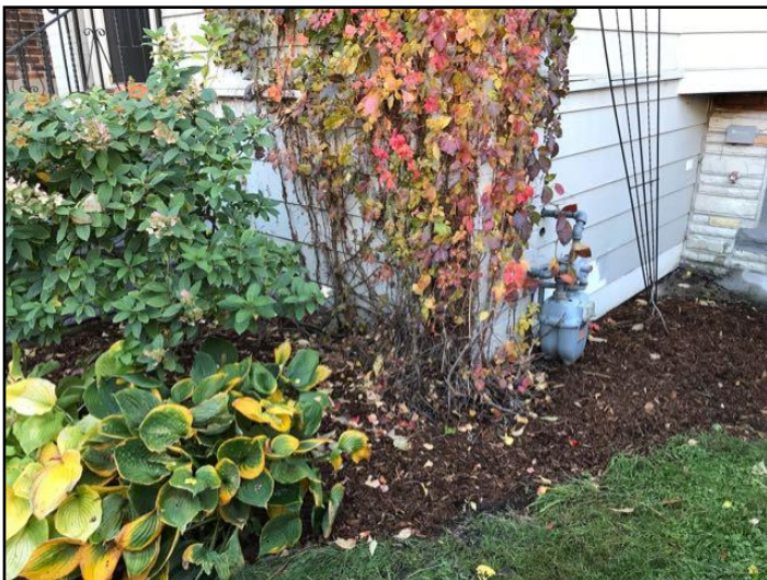
Wood/soil contact, water damage
