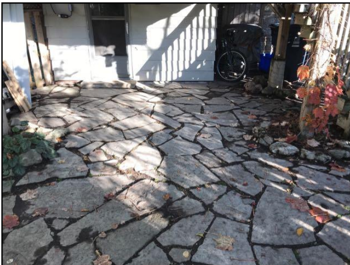
Improper slope or drainage
