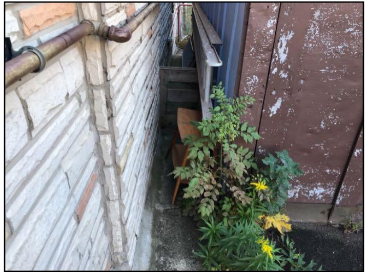
Improper slope or drainage
