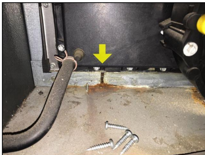
Prior condensate leak...
