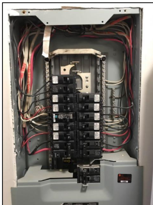
Breakers - Rear first floor
