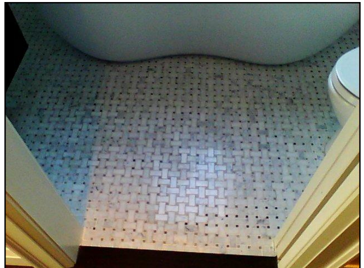
Radiant floor heating (electric)
