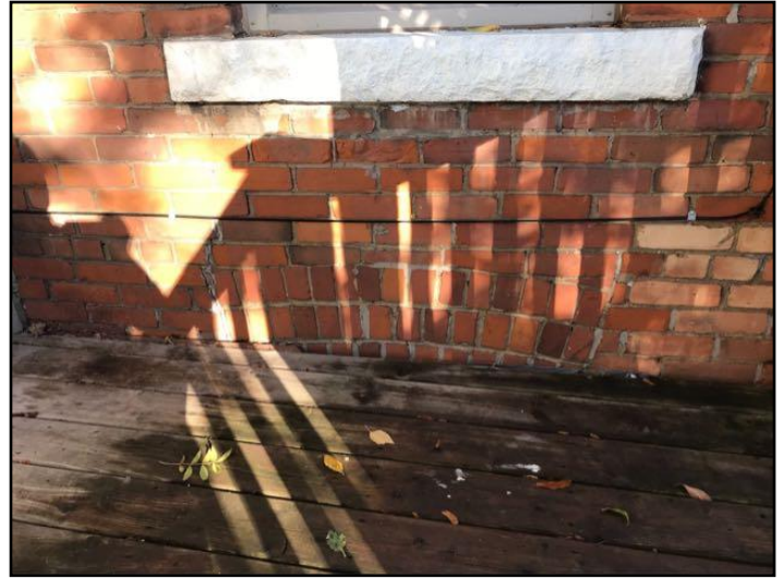
Typical minor cracks
