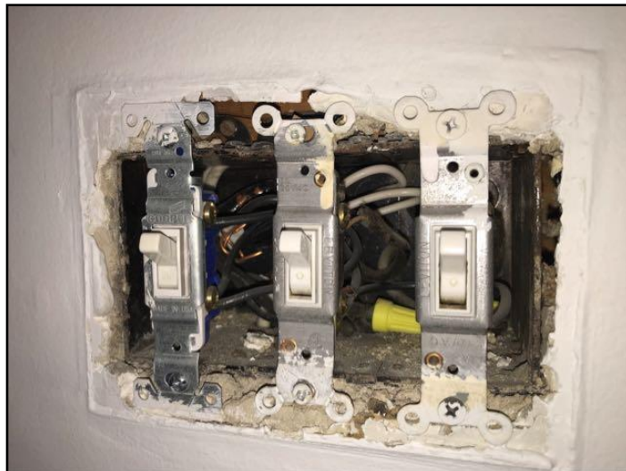
Knob and Tube Wiring - in use
