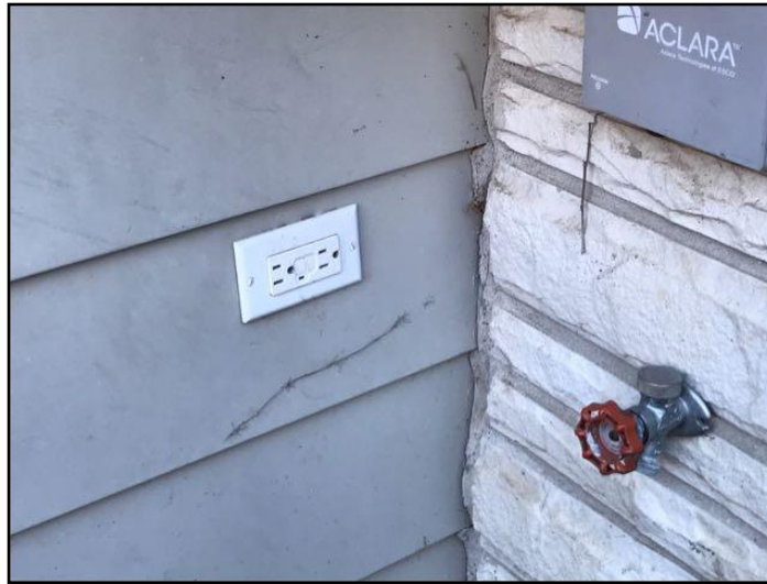
GFCI outlet - wrong type
