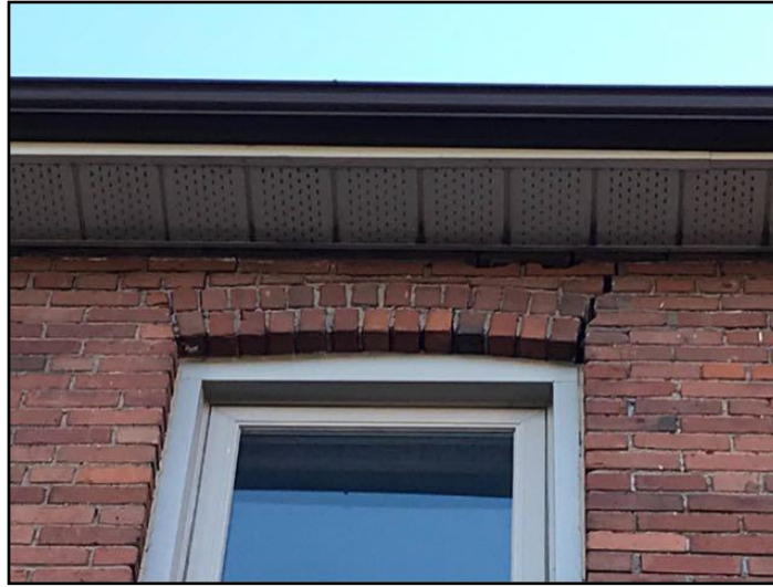
Arch - movement, cracks
