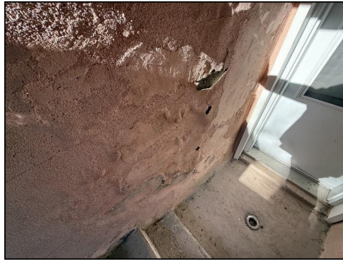
28. Spalling or damaged parging
