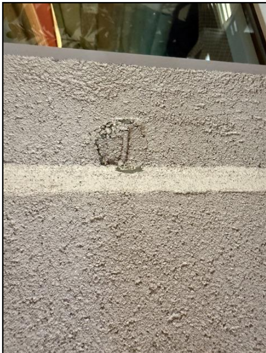
33. Minor damage at EIFS stucco
