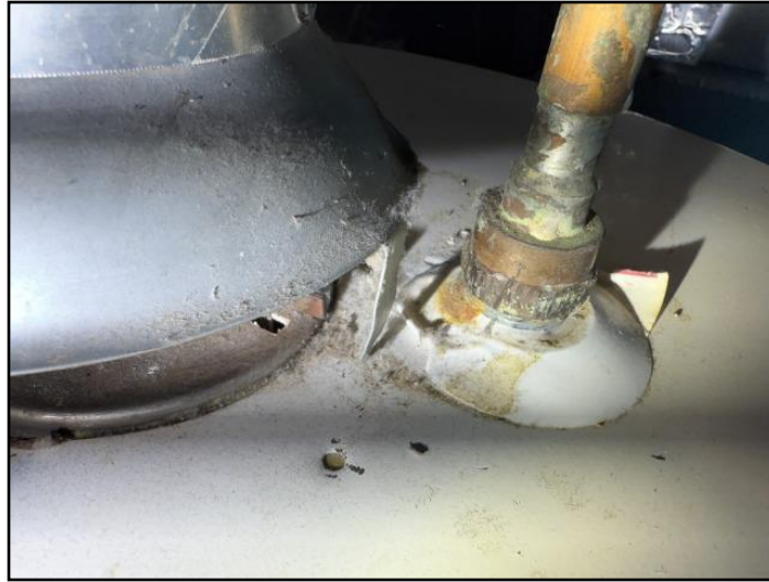
53. Spillage or backdraft at the draft hood
