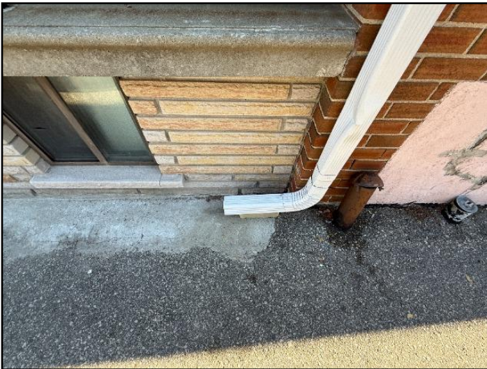
9. Discharge too close to building
