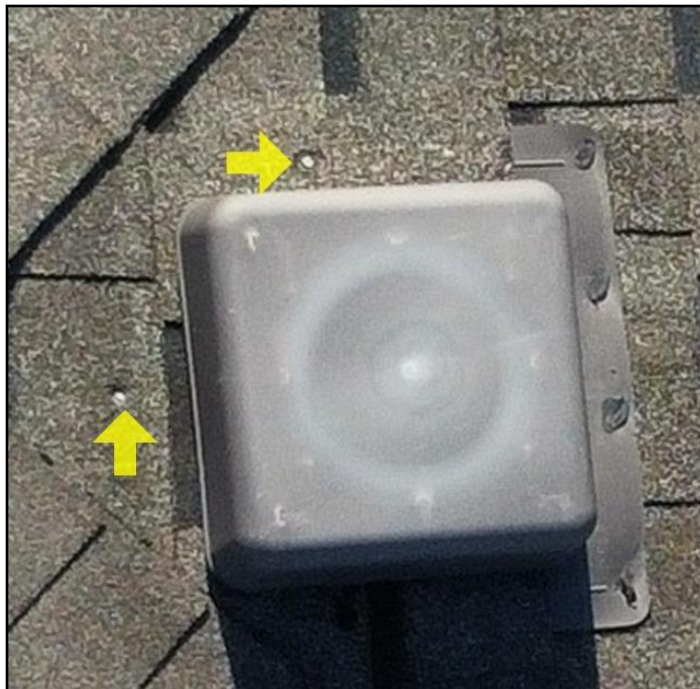
5. Exposed fasteners not sealed
