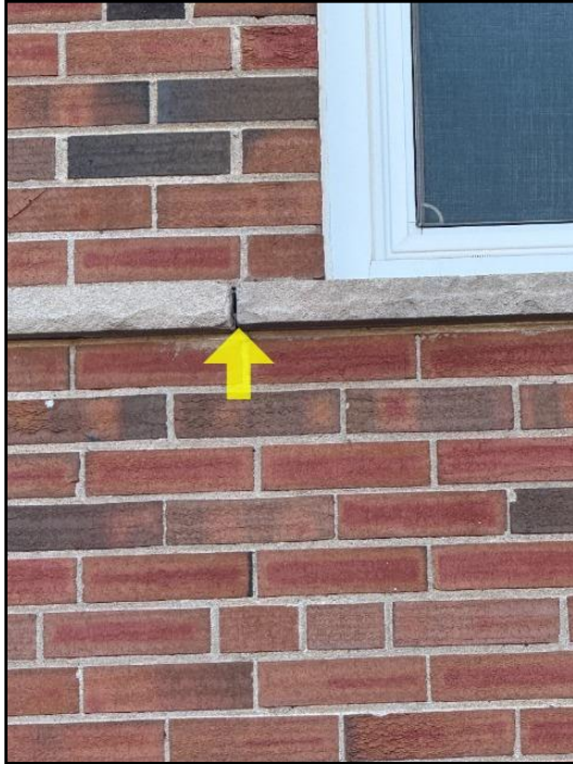
17. Mortar deterioration at window sill control...
