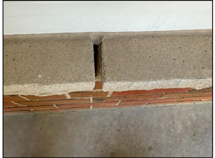
18. Mortar deterioration at window sill control...
