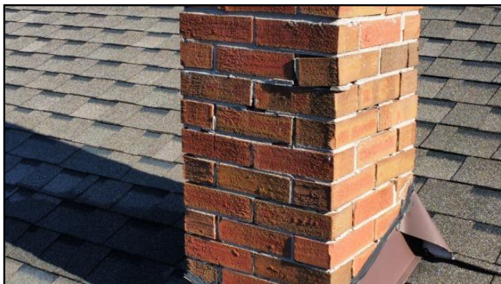
47. Loose, missing or deteriorated masonry...
