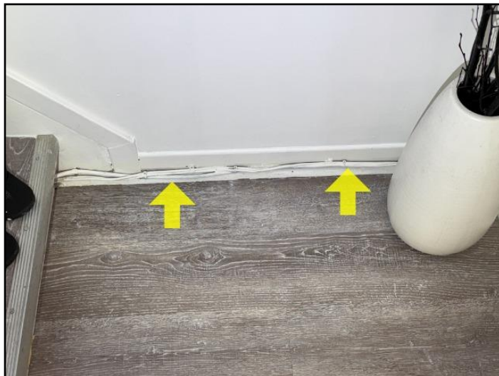
42. Exposed on walls or ceilings
