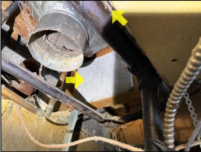
61. Possible asbestos containing materials
