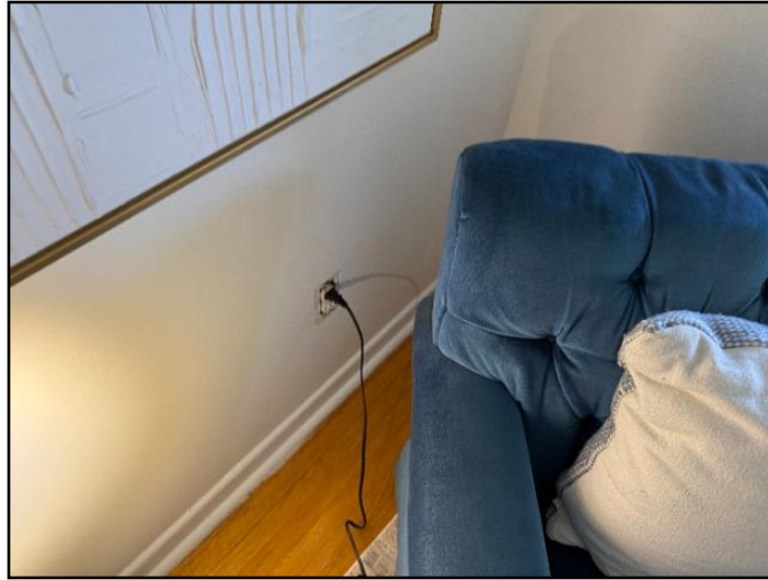
46. For outlet (receptacle) is missing
