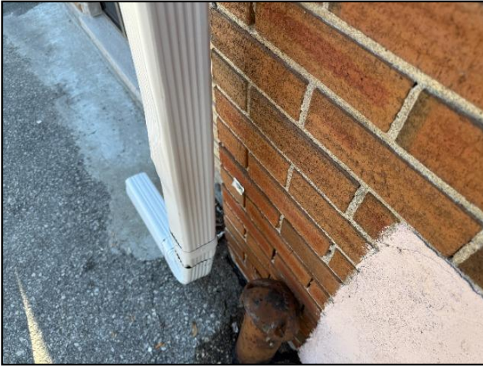
11. Not well secured
