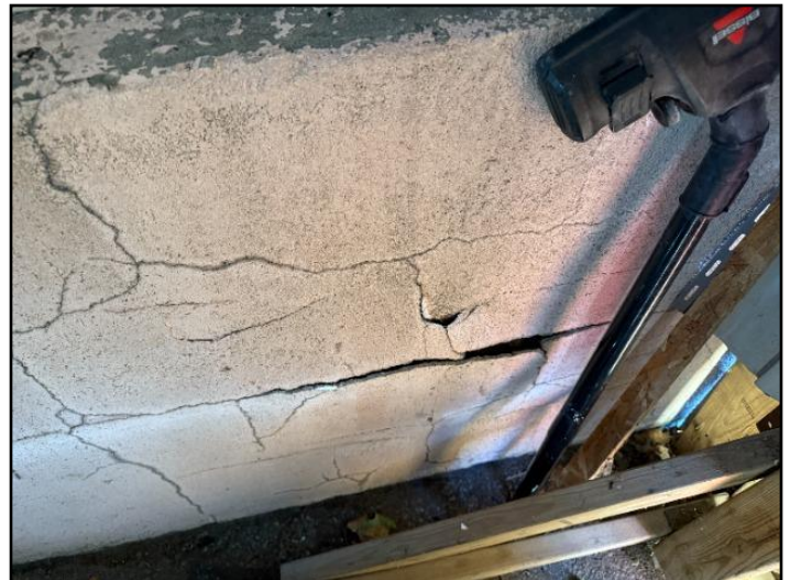
27. Cracked parging and wall behind parging
