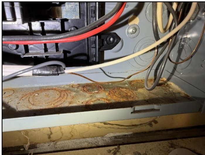
37. Rust or water in panel
