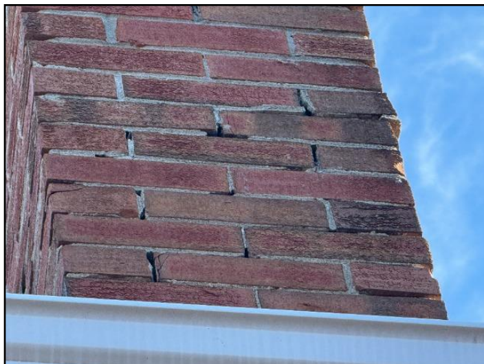
48. Loose, missing or deteriorated masonry...
