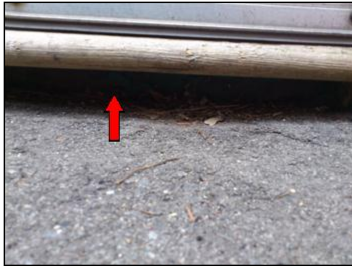
Gap under door
