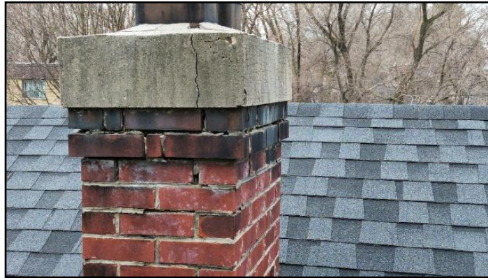
11. Loose, missing or deteriorated masonry...
