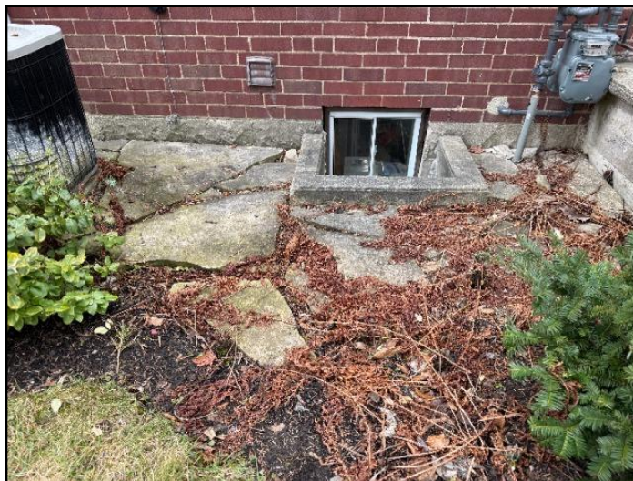
7. Improper slope or drainage
