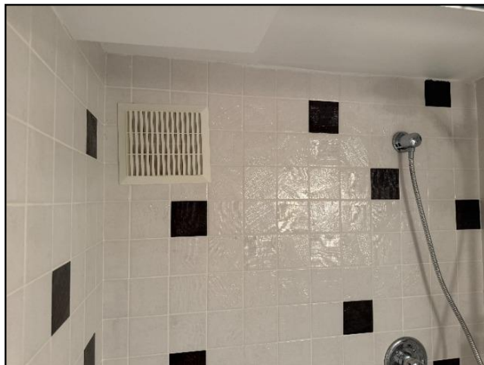
15. Bathroom exhaust fan installed within the...
