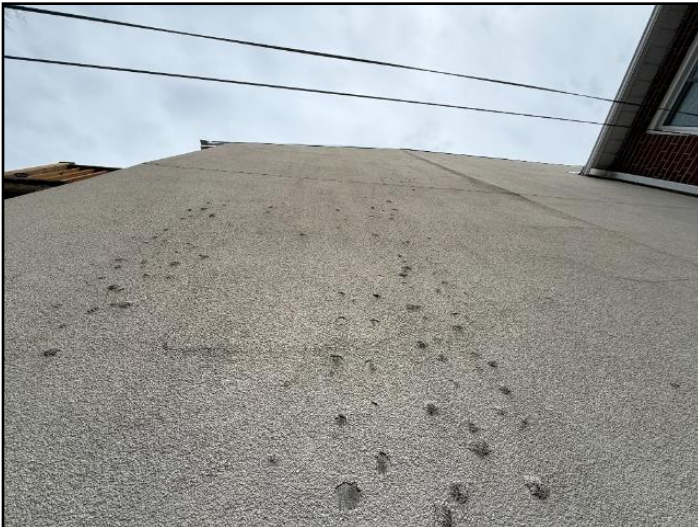
5. minor surface damage examples
