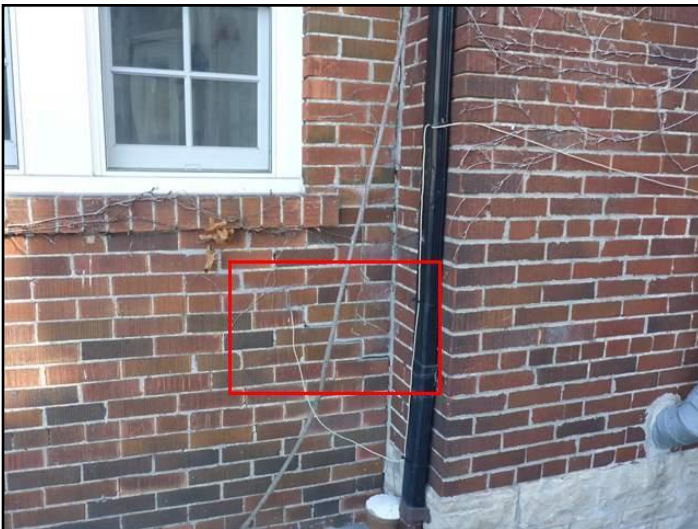
Step crack at porch side wall
