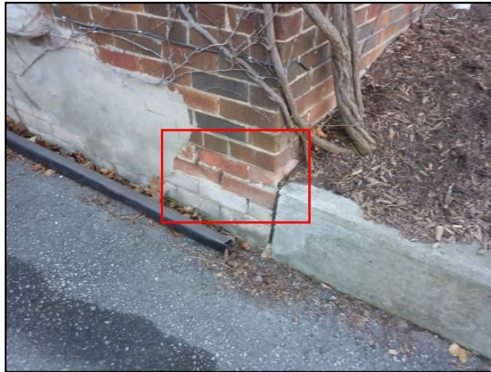
Masonry deterioration at grade level
