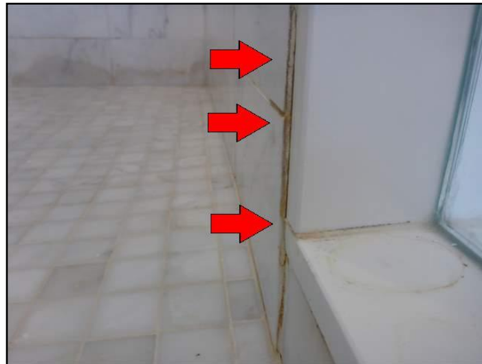
Tile pushing outwards slightly
