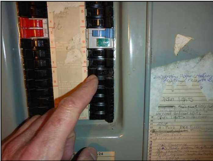
Breaker in OFF position
