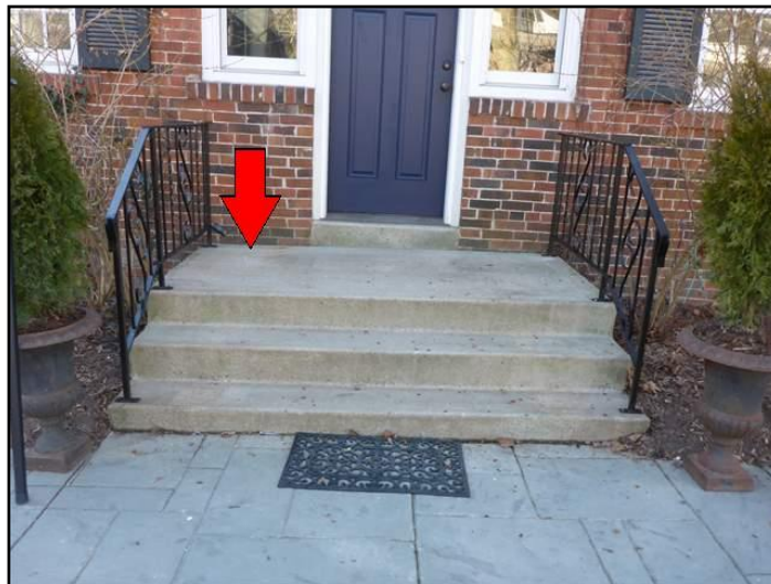
Minor settlement noted at stair system
