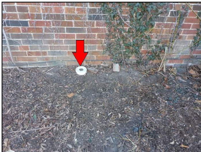
Newer cleanout at front yard
