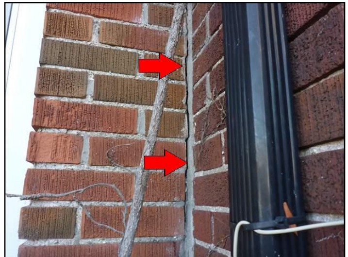
Cracked where porch meets house
