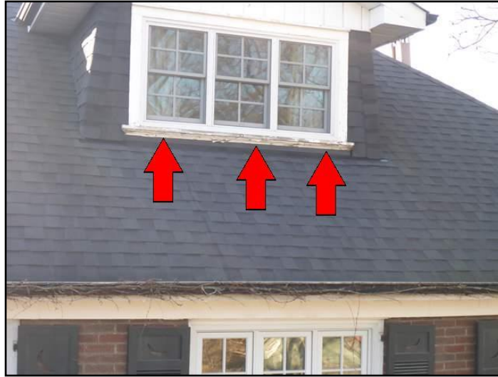
Paint needed at front
