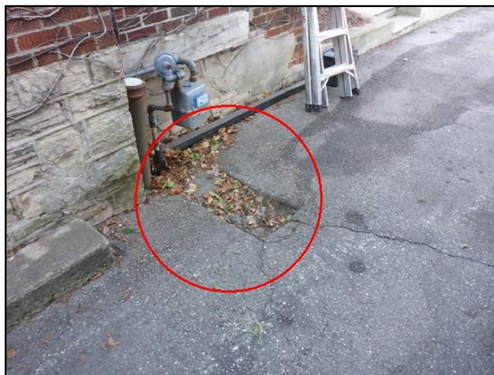
Trip hazard at driveway
