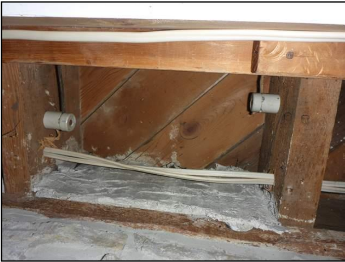
Remnants of knob-and-tube wiring (basement)
