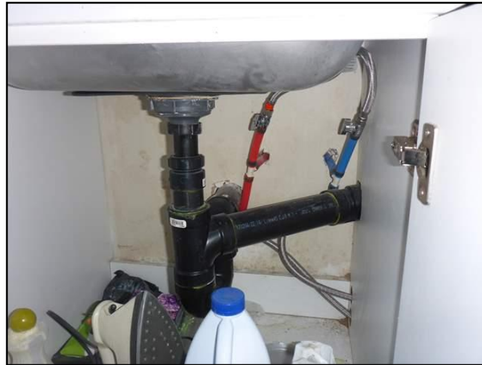
Leak at laundry tub drain
