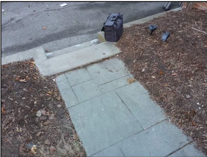
Trip hazard at edge of walkway
