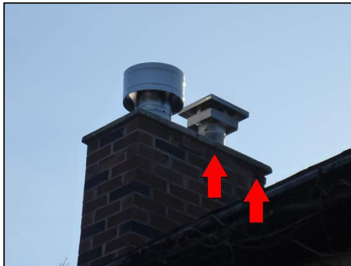
Loose, missing or deteriorated masonry
