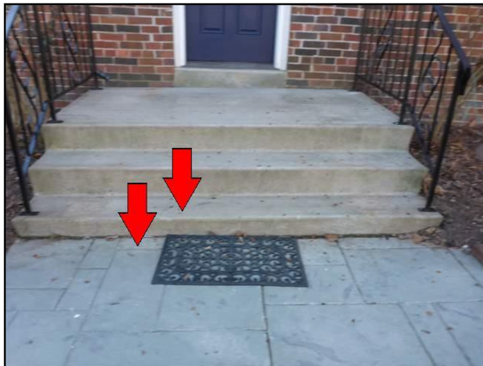
Trip hazard at short bottom step?
