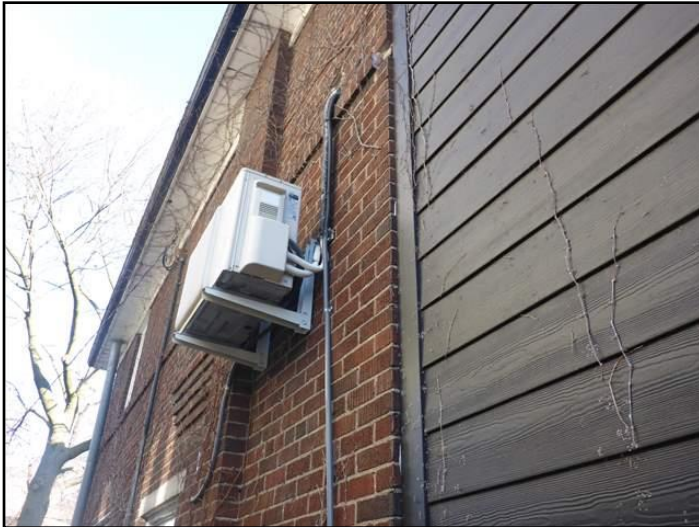
Ductless (Mini split) system- outdoor unit
