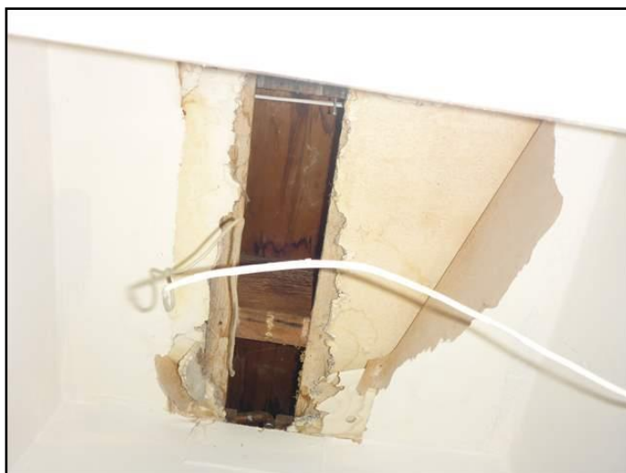
Damage- drywall removed at closet ceiling
