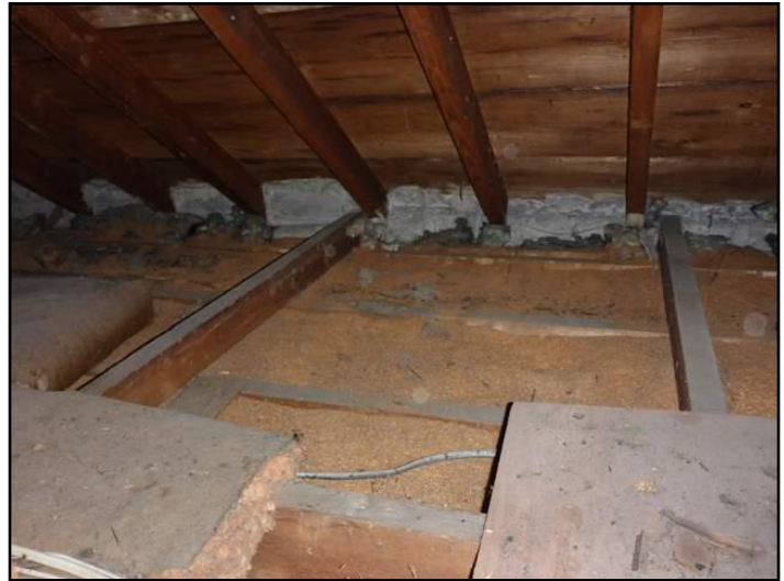
Wood shavings at front knee wall
