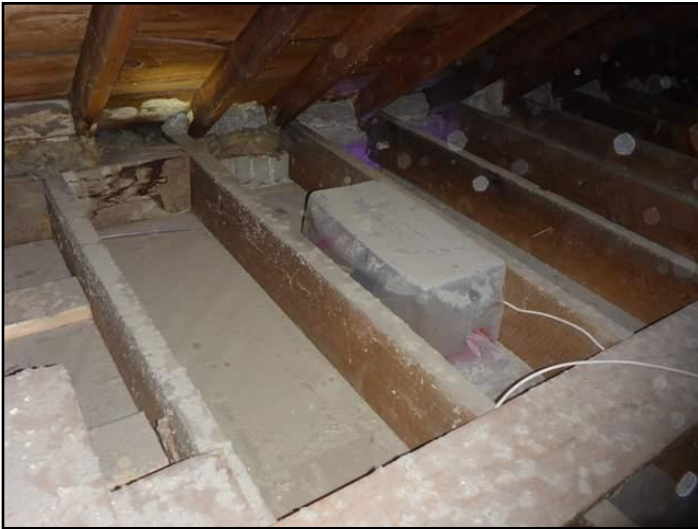
No insulation at rear knee wall
