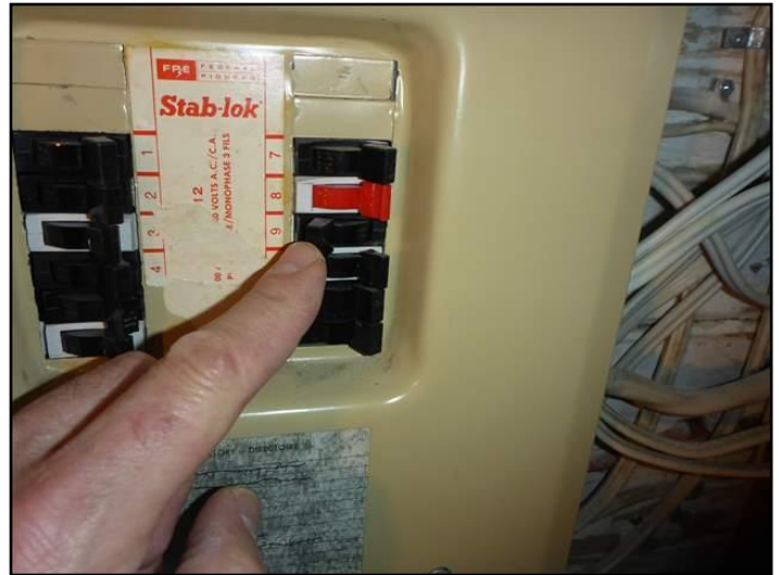
Breaker in OFF position
