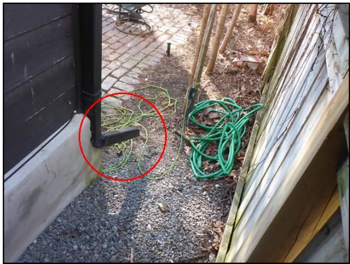
Discharge too close to building
