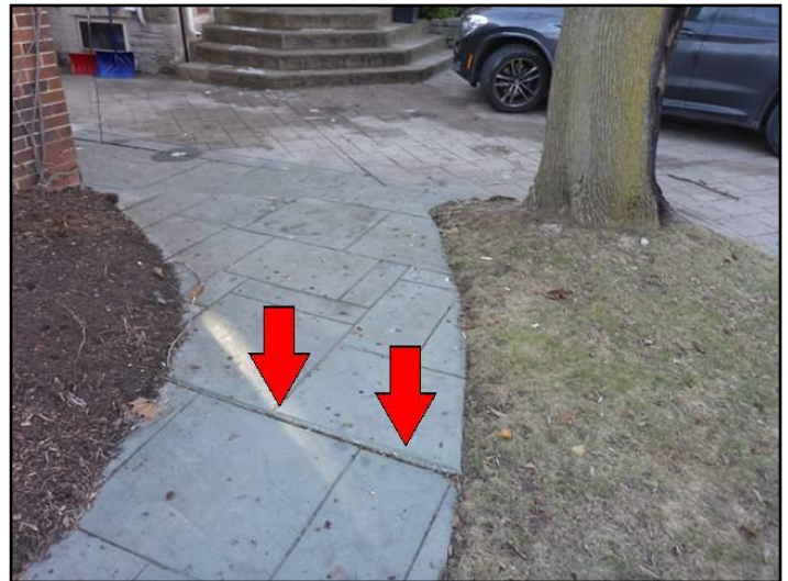
Trip hazard beside tree
