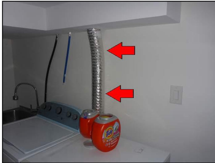
Dryer vent material not smooth wall
