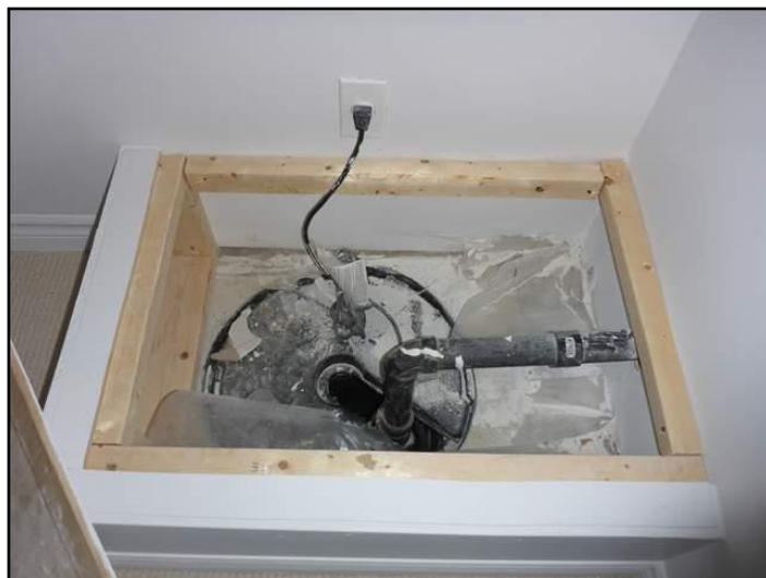
Sump pump (rear addition)
