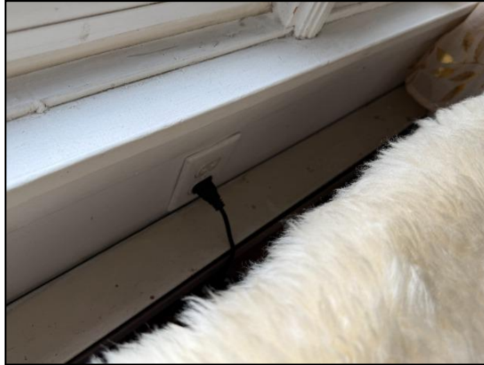
14. Above electric baseboard heaters
