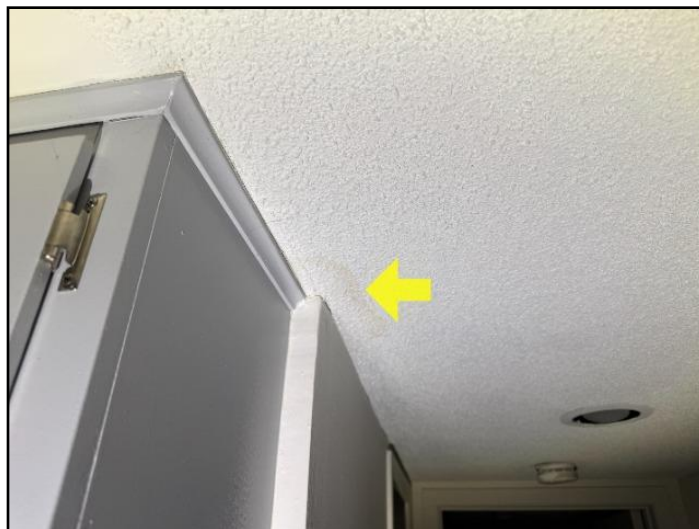
17. Water stains - Dry at time of inspection
