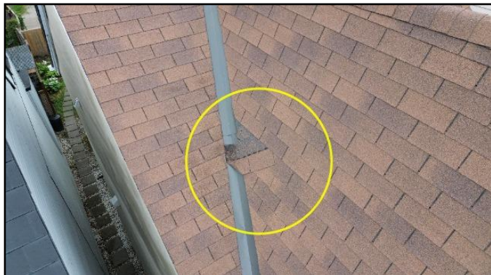
3. Missing, loose or torn
