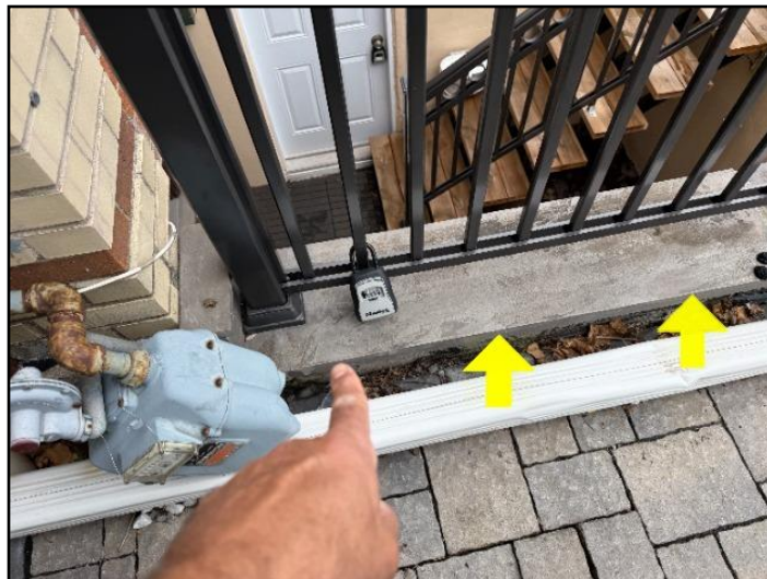
8. Guard and handrail problems
