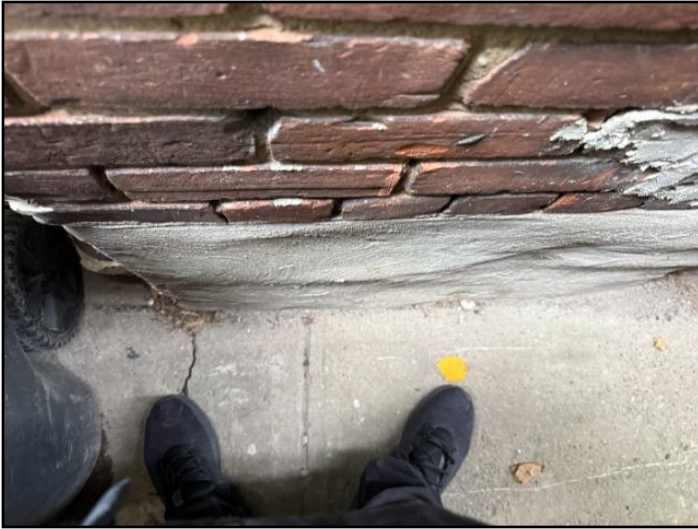
11. Masonry and/or mortar deterioration
