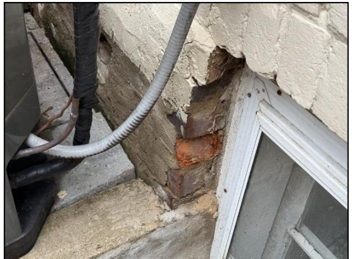
14. Masonry and/or mortar deterioration
