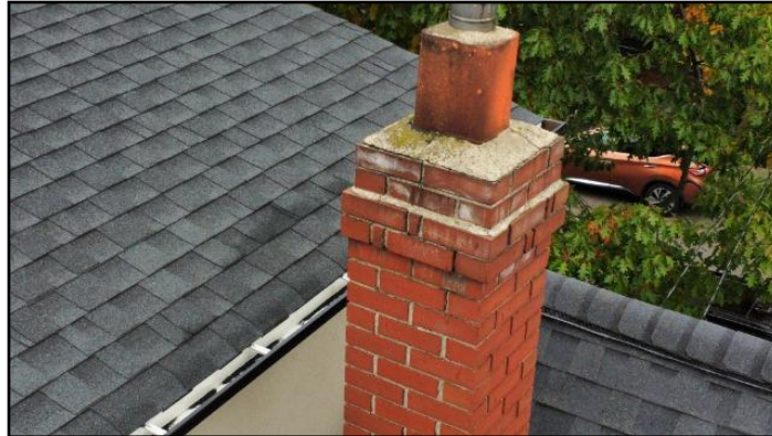
23. No drip edge on cap (crown)
