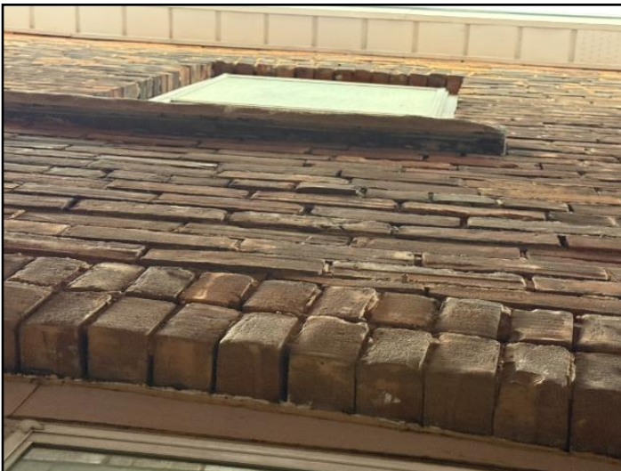
13. Masonry and/or mortar deterioration
