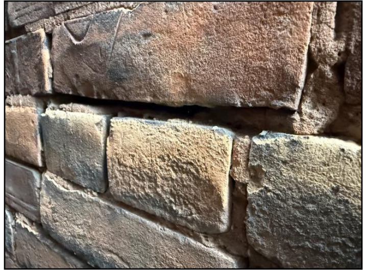
12. Masonry and/or mortar deterioration
