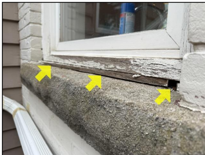
16. Missing or loose pieces
