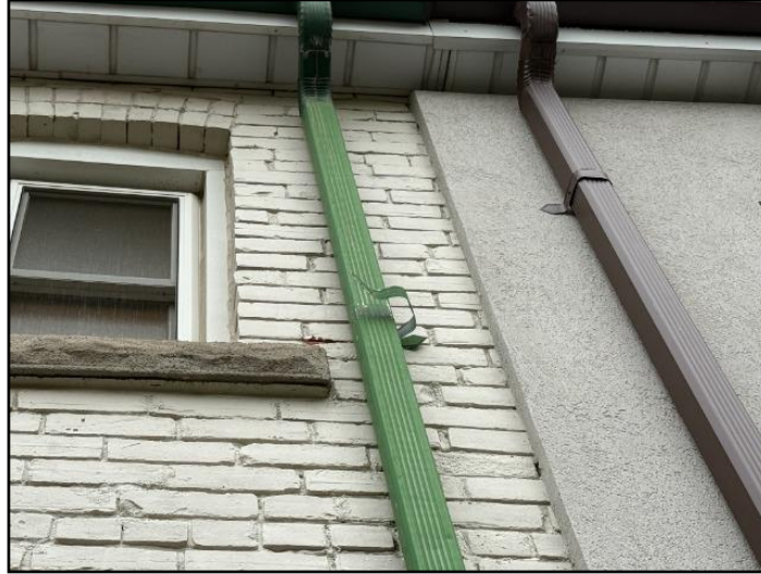
10. Not well secured
