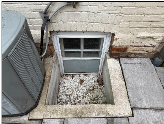
17. Less than 6 inches below window
