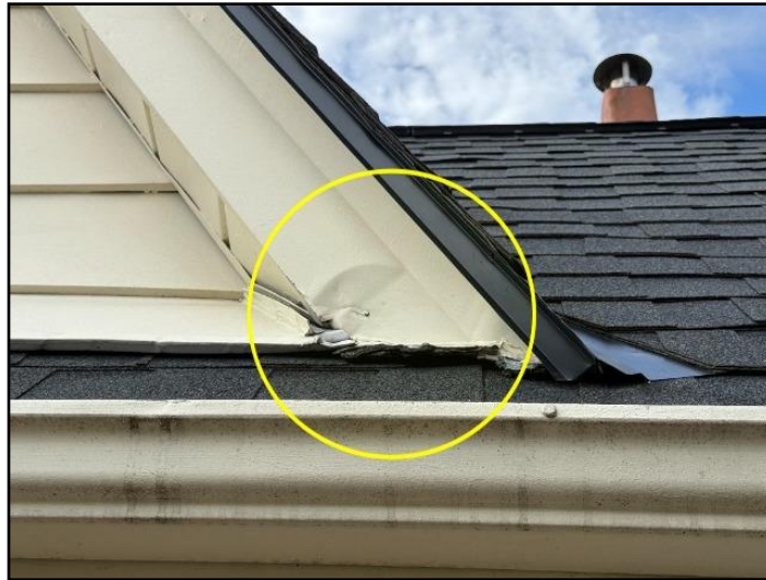
5. Damage, loose, open seams, patched
