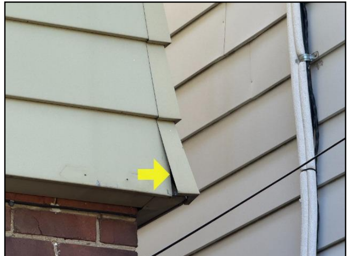
8. Loose or missing pieces
