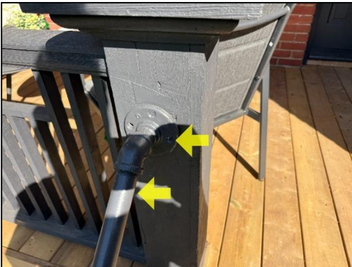
13. Too low and poorly fastened
