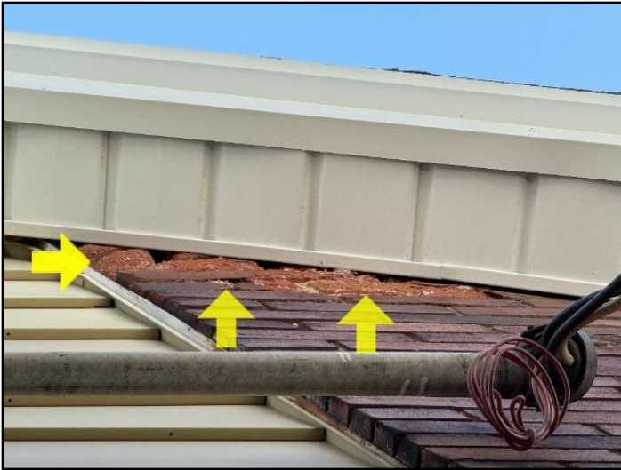
9. example spalling at side
