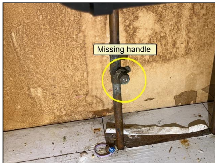
21. Missing isolation valve handle
