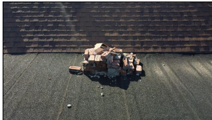
5. Debris on roof
