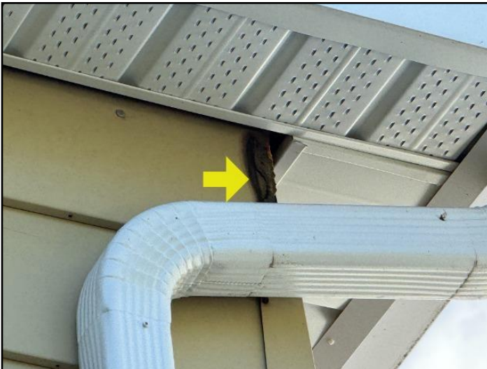
7. Loose or missing pieces
