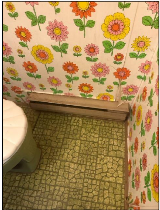
82. Electric baseboard heaters
