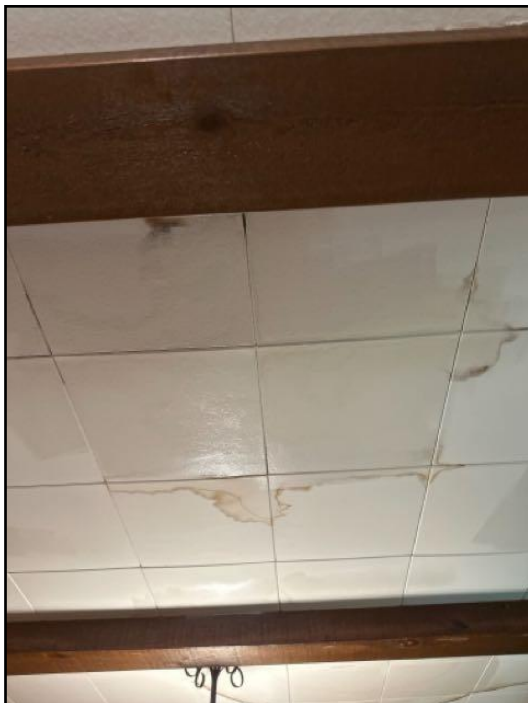
15. Vulnerable to ice damming
