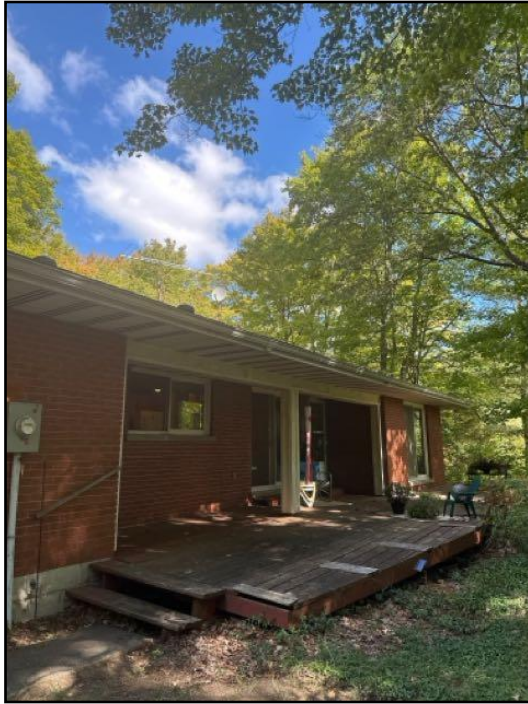
13. Vulnerable to ice damming
