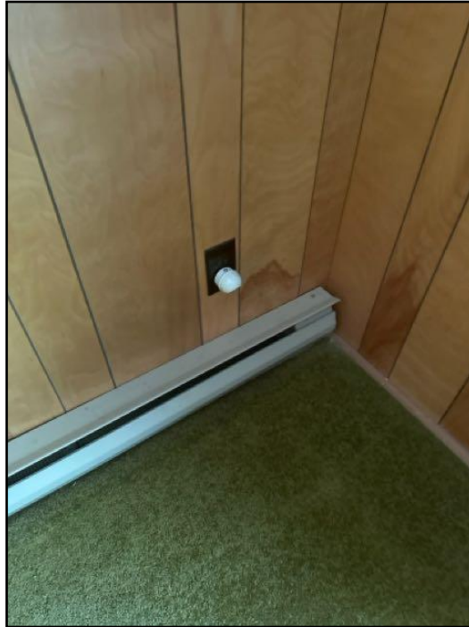
116. Electrical receptacle above heater
