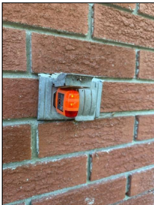
75. GFCI/GFI needed (Ground Fault Circuit...
