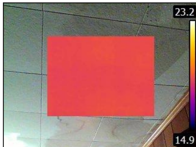
30. Vulnerable to ice damming
