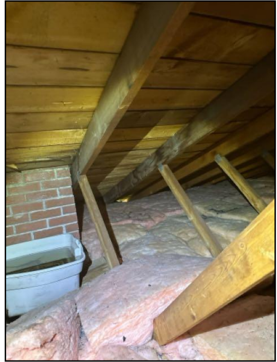
14. Vulnerable to ice damming
