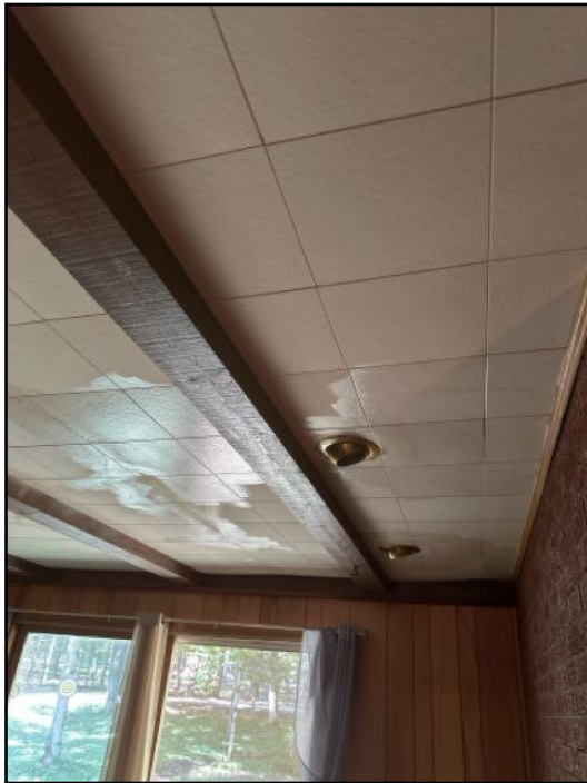
17. Vulnerable to ice damming
