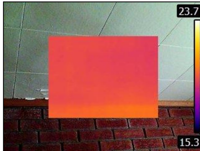
31. Vulnerable to ice damming
