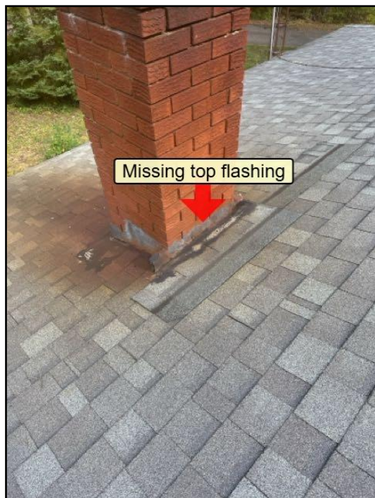
32. Vulnerable to ice damming
