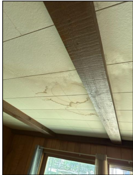
18. Vulnerable to ice damming
