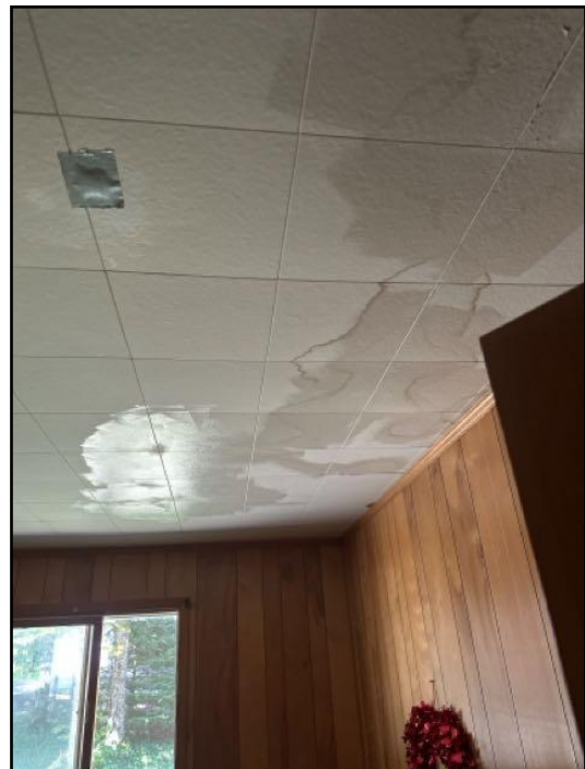
20. Vulnerable to ice damming
