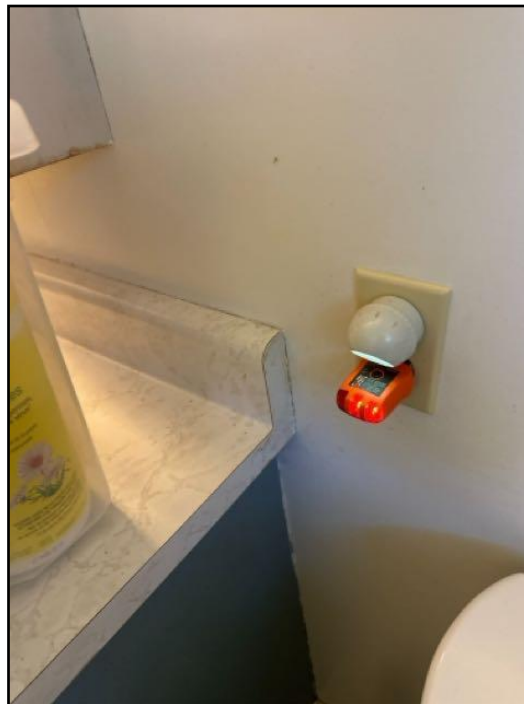
78. GFCI/GFI needed (Ground Fault Circuit...
