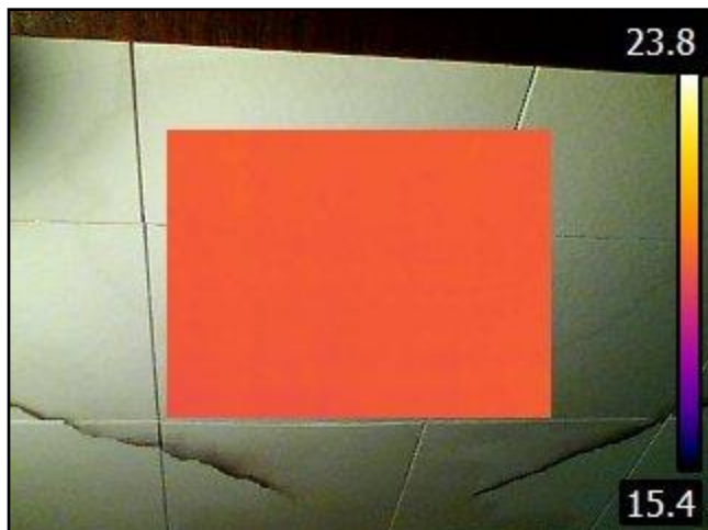
27. Vulnerable to ice damming
