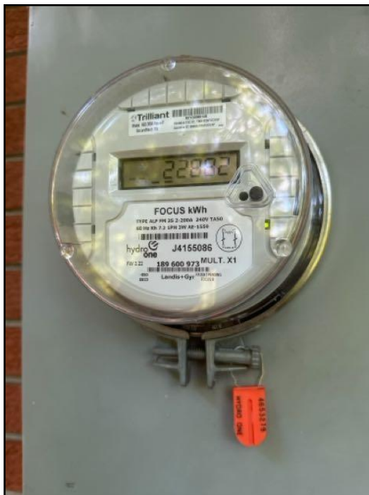
66. Underground - cable material not visible
