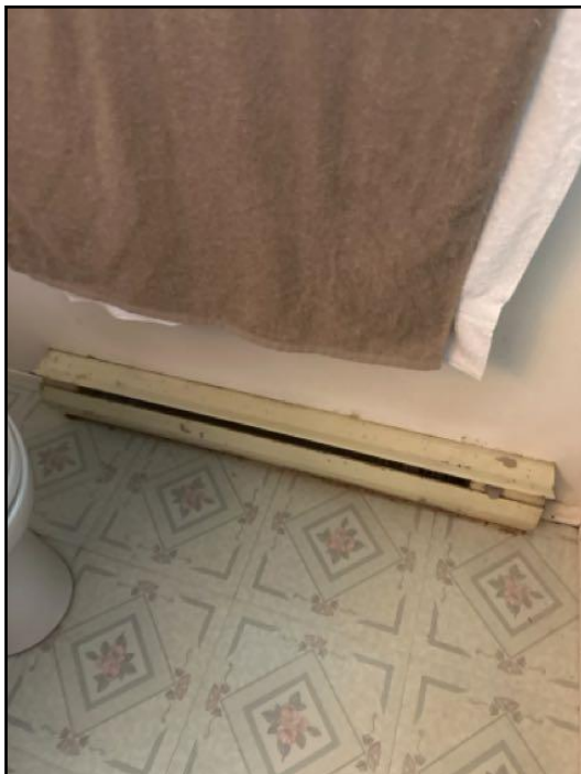
87. Electric baseboard heaters
