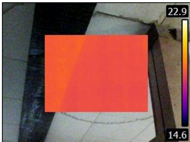
25. Vulnerable to ice damming
