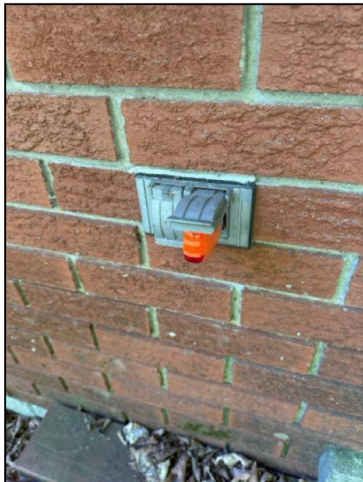
77. GFCI/GFI needed (Ground Fault Circuit...
