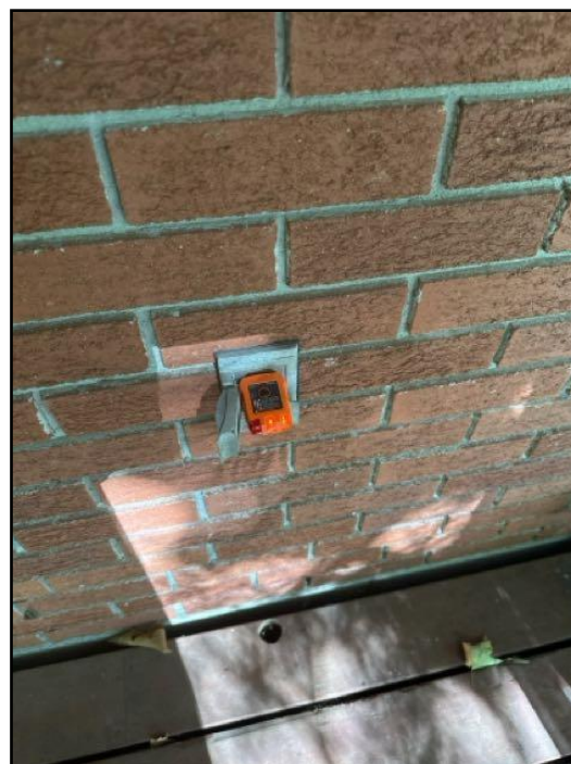
76. GFCI/GFI needed (Ground Fault Circuit...
