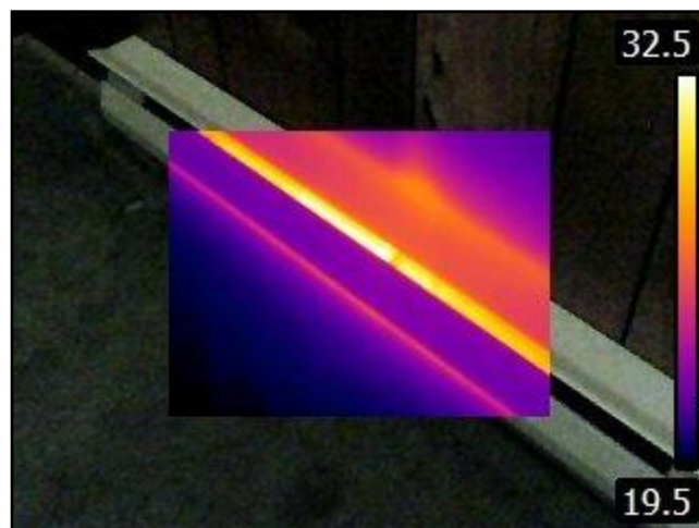
92. Electric baseboard heaters
