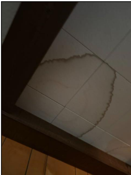
19. Vulnerable to ice damming
