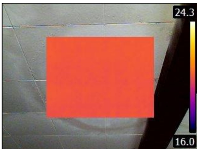
23. Vulnerable to ice damming
