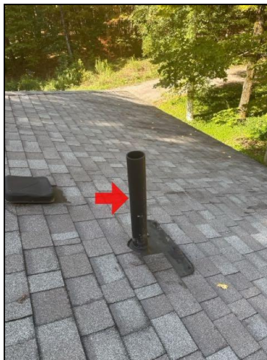
146. Vent termination problems
