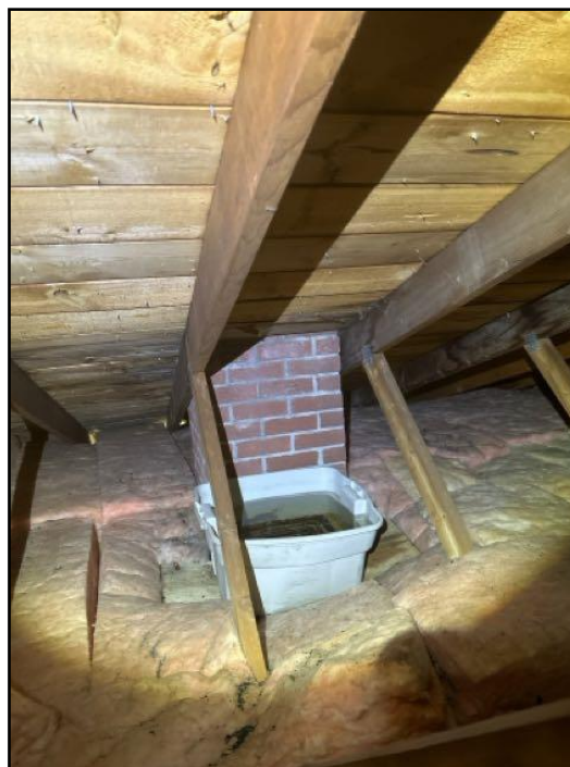
33. Vulnerable to ice damming
