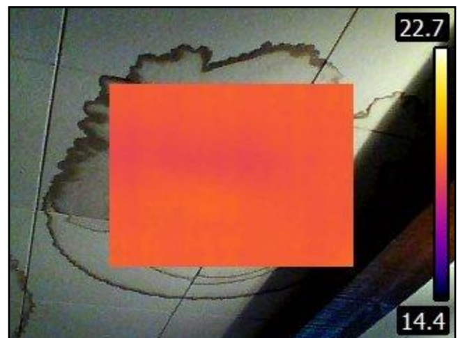
24. Vulnerable to ice damming
