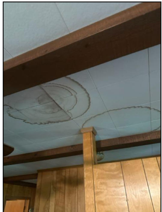
16. Vulnerable to ice damming
