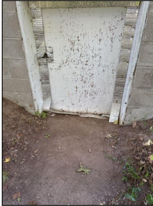
56. Improper slope or drainage
