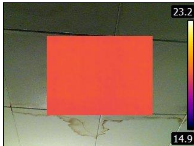
26. Vulnerable to ice damming
