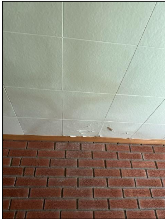
21. Vulnerable to ice damming
