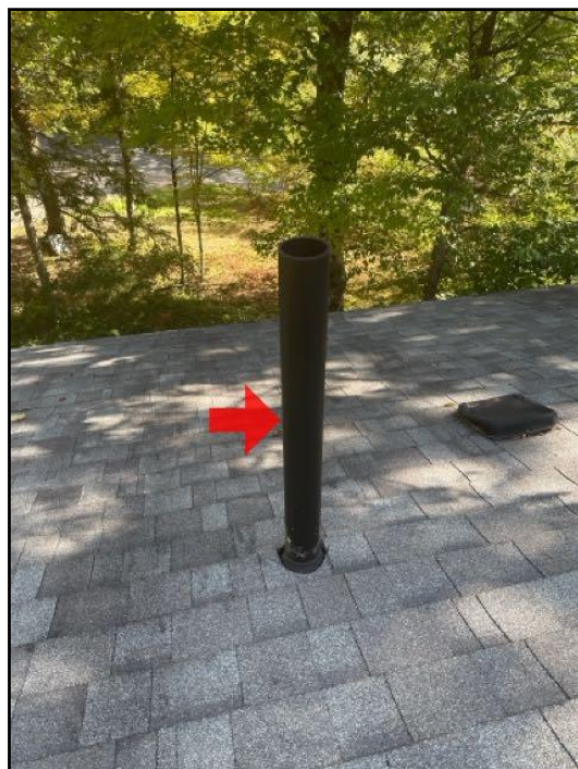
145. Vent termination problems
