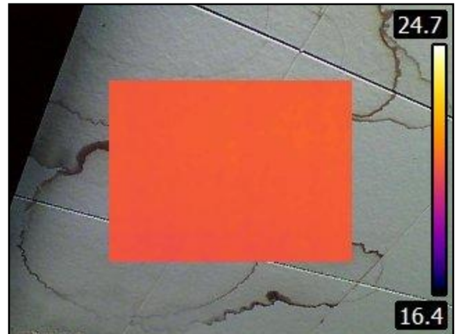
22. Vulnerable to ice damming
