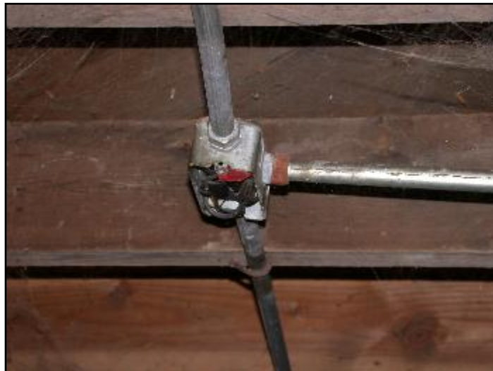
7. missing cover for junction box
