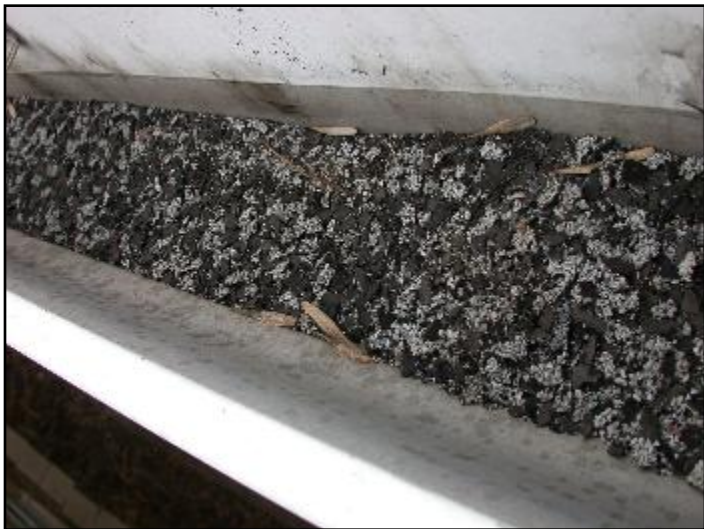
4. These are deteriorated shingle granules
