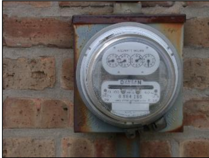
6. This is the meter located rear south east
