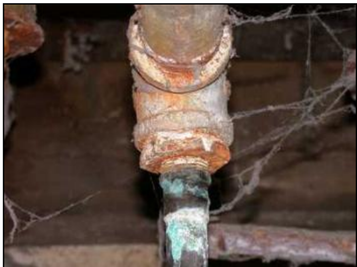
10. copper should not connect to galvanized
