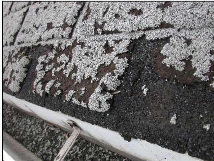
1. Note missing granules
