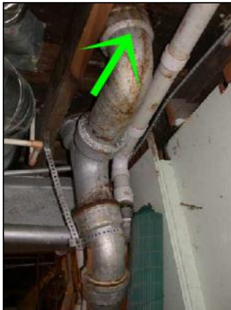
11. underside of toilet shows leaking
