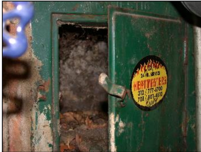
9. Clean out should be cleaned of debris
