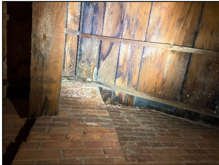
11. Water stains or discoloration - Attic plank...
