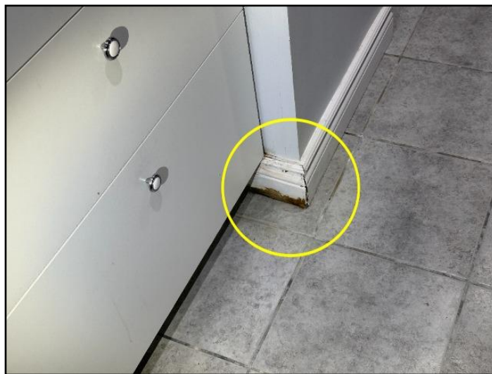
21. Damaged plaster, dry wall or other finished...
