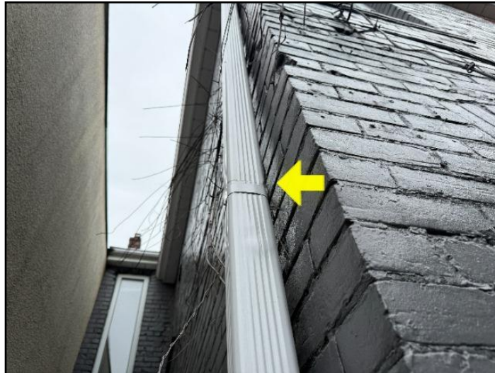
3. Not well secured
