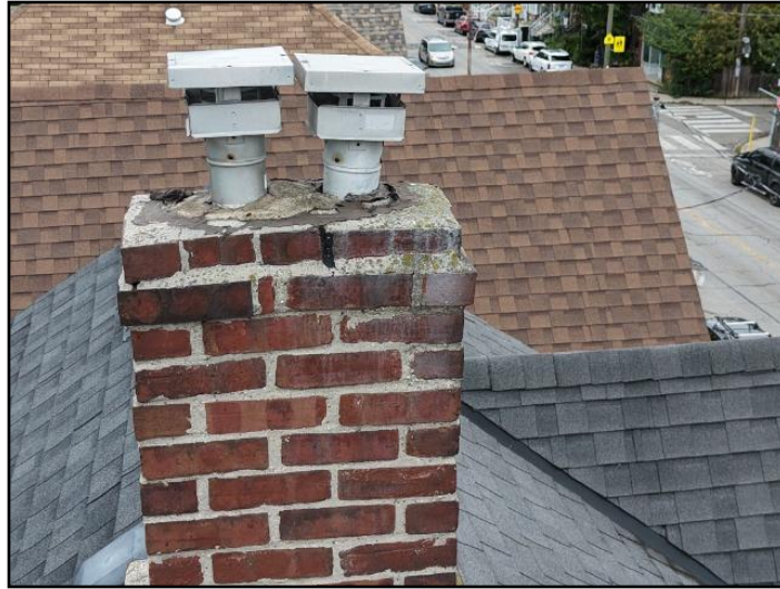
15. No drip edge on cap (crown)
