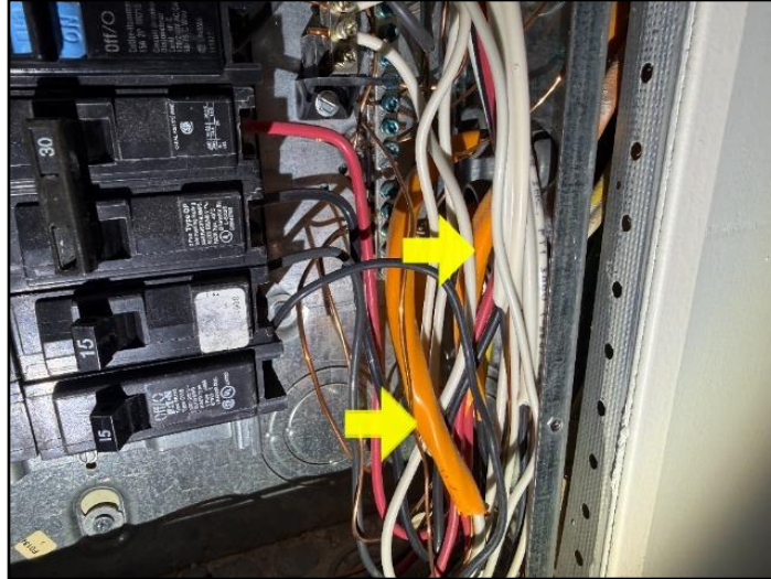
13. Sheathing not removed
