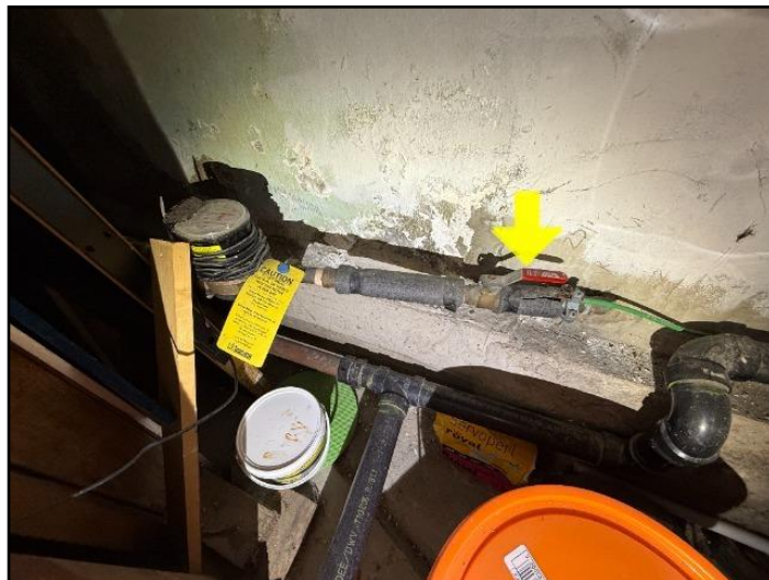
8. Main water shut off valve - Front of the...
