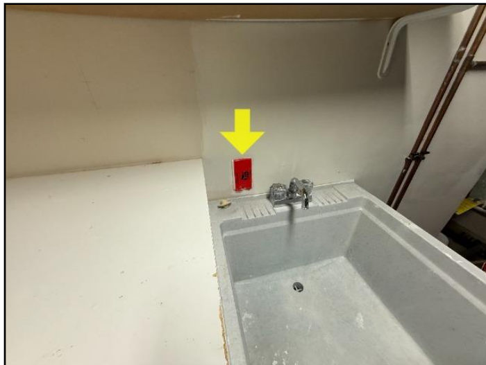
7. GFCI/GFI needed (Ground Fault Circuit...)
