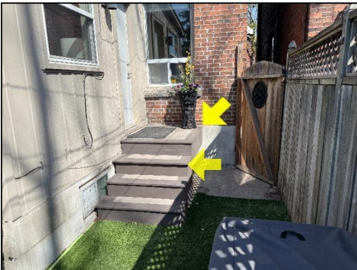
4. Missing hand/guard rails
