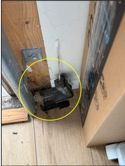
7. Sensors poorly located
