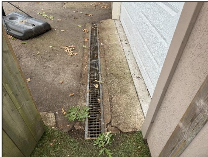
6. Debris Accumulation or Clogged catch basin
