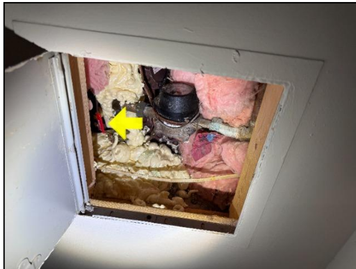
13. Main water shut off valve - Basement
