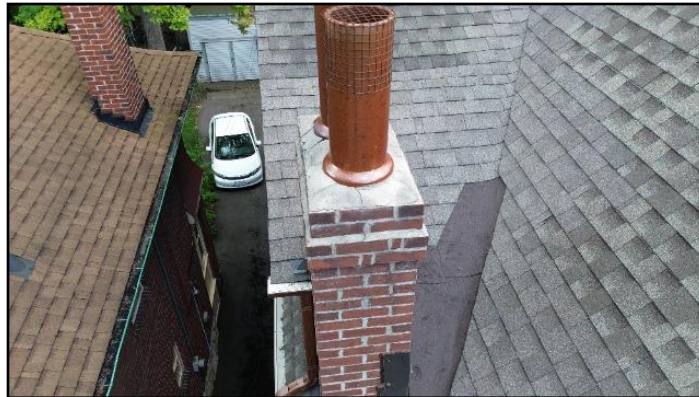
12. No drip edge on cap (crown)
