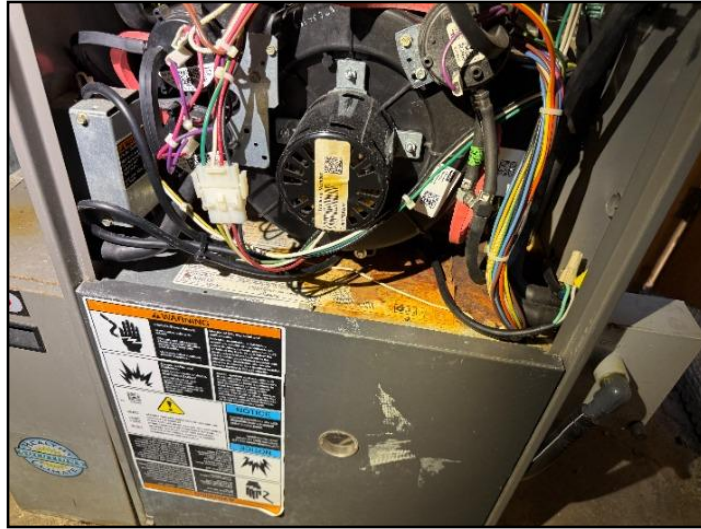
18. Condensate prior issues and/or rust
