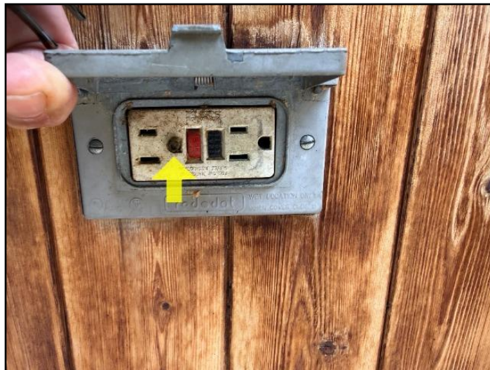
15. Test faulty on GFCI/GFI (Ground Fault...
