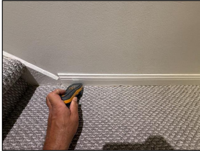
27. Water damage and/or stains, tested dry
