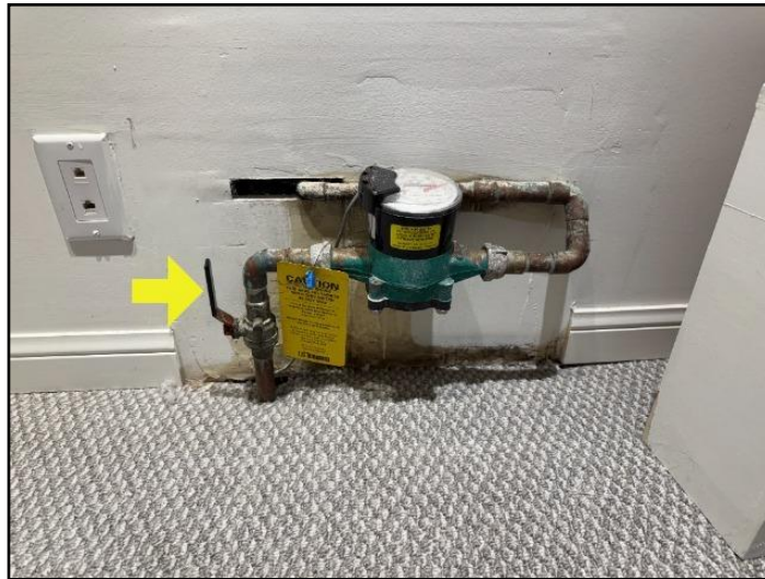
20. Main water shut off valve - Front of the...
