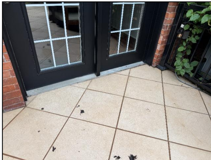
8. Threshold too low
