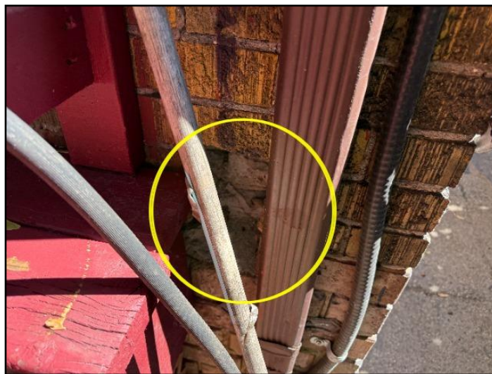
11. Gap or Hole at wall
