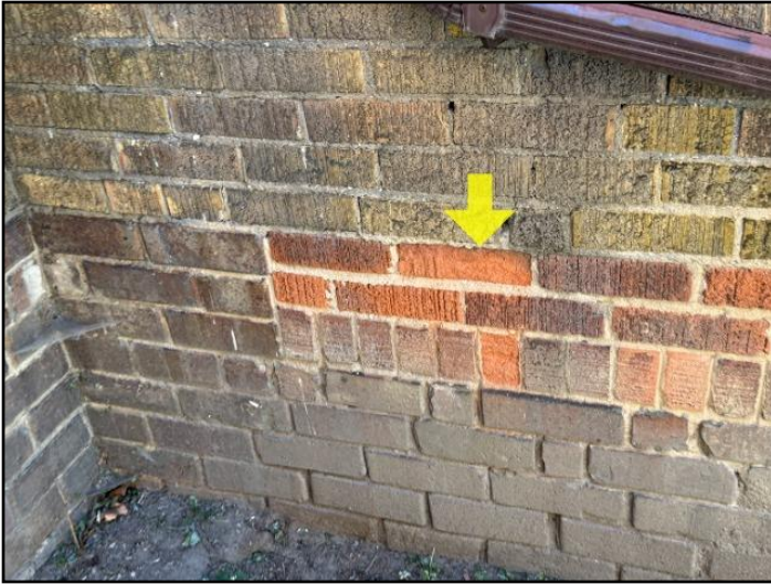
12. example of spalling
