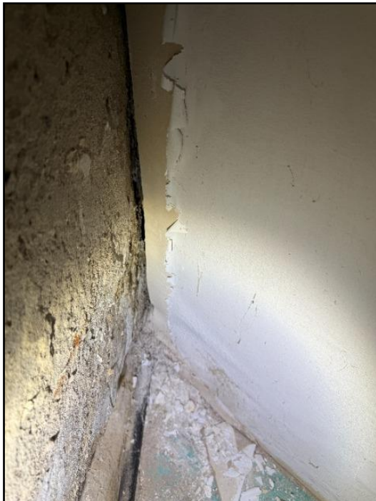
28. Water damage and wet
