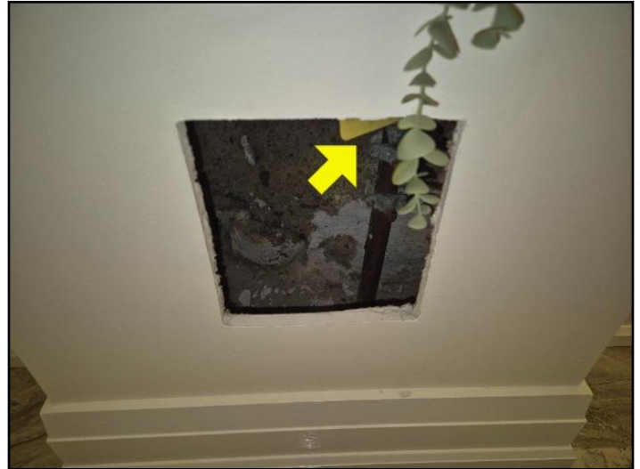
26. Main water shut off valve - Basement
