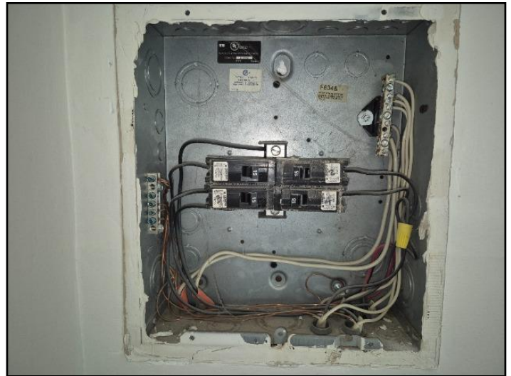
21. Breakers - Sub panel third floor
