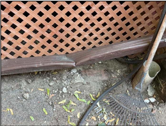
6. example of damage
