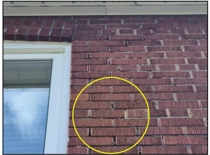
5. Masonry and/or mortar deterioration
