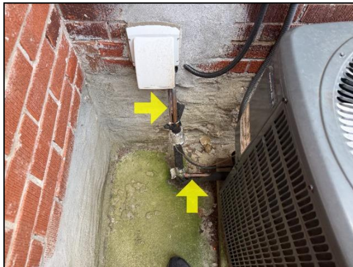
12. Insulation - missing or damaged
