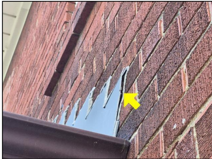
3. Damage, loose, open seams, patched
