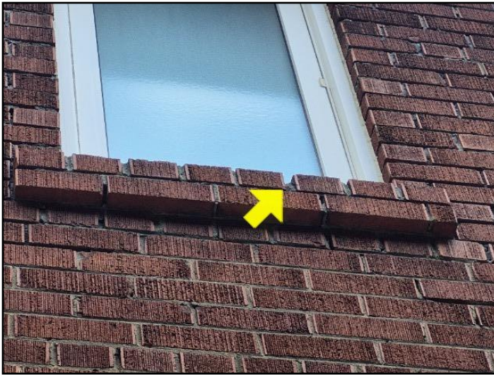
4. Masonry and/or mortar deterioration
