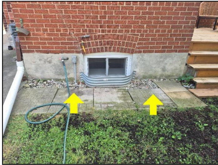
6. Improper slope or drainage
