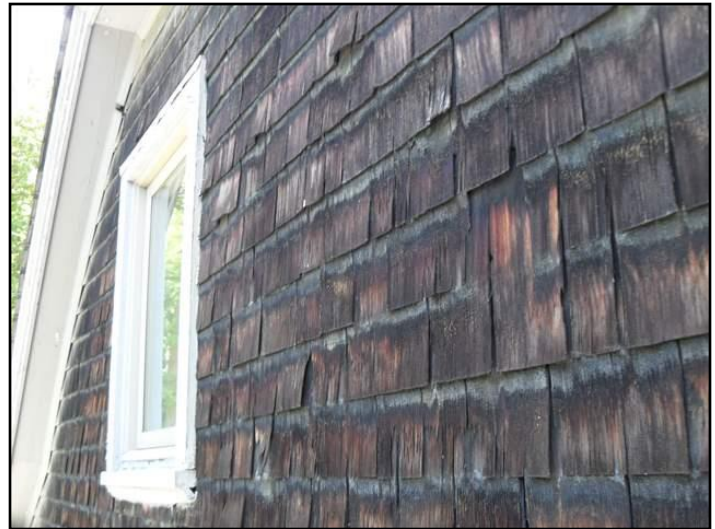
Missing shingle noted.
