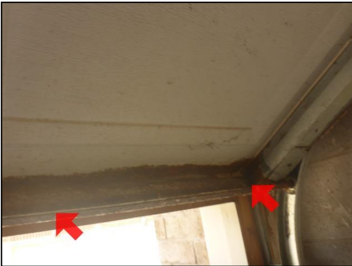
Rust along bottom edge of door
