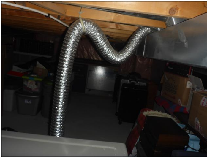
Flexible duct is too long, prone to clogging
