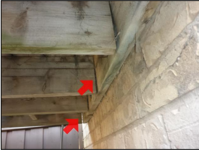
Joists pulling out, hangers needed
