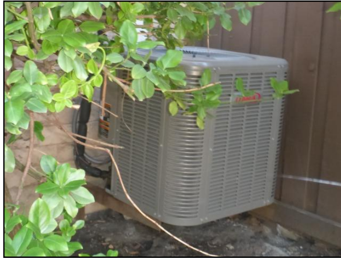
Air cooled- outdoor unit
