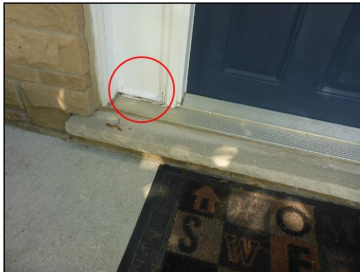
Trim deterioration beside front door
