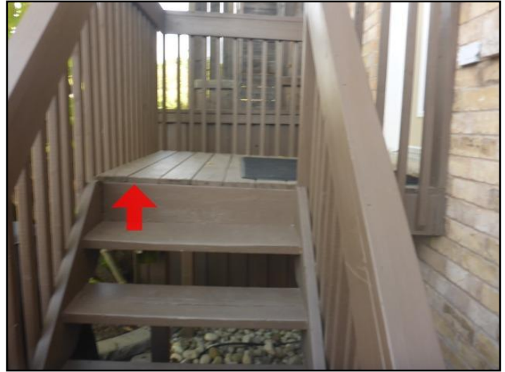
Outboard edge of deck is lifted
