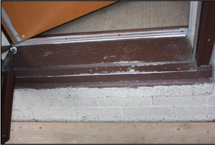
6. Inadequate sill projection
