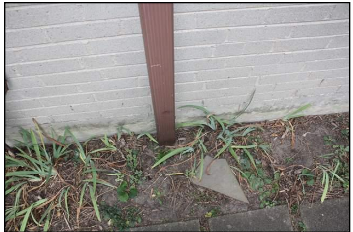
2. Discharge below grade
