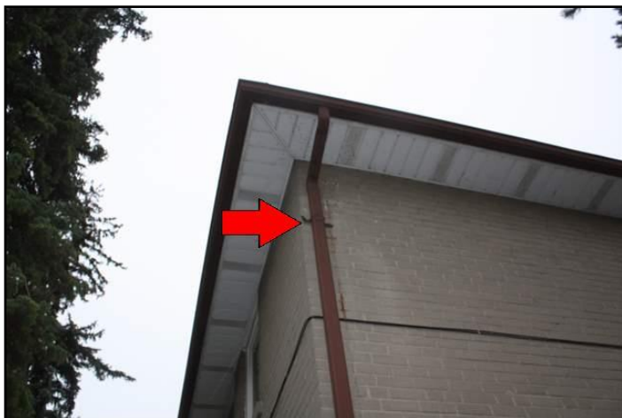
3. Not well secured
