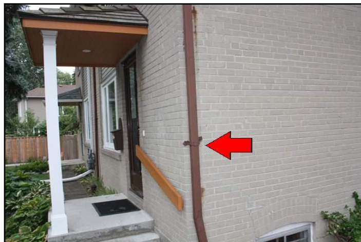
4. Not well secured
