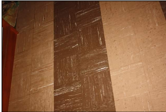
20. Possible asbestos containing materials
