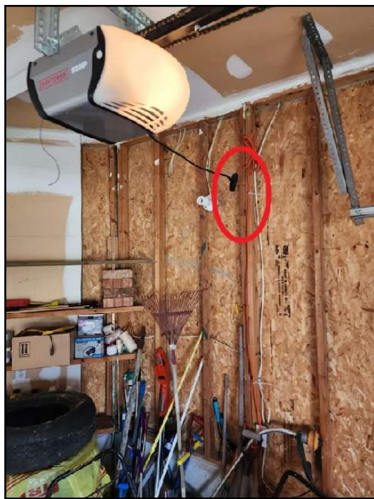
13. Extension cord for garage door operator...
