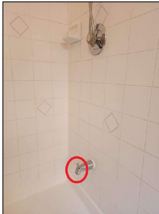
21. Shower diverter inoperative or defective
