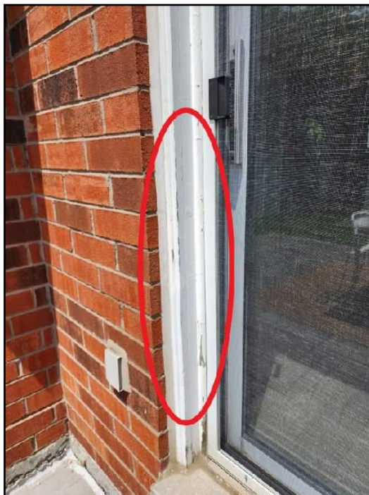
5. Paint or stain - deteriorated / missing
