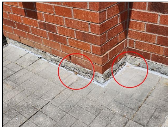
11. Spalling, crumbling or broken material
