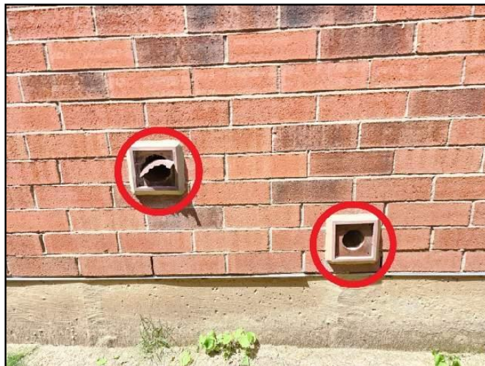
4. Vent covers missing, loose or damaged
