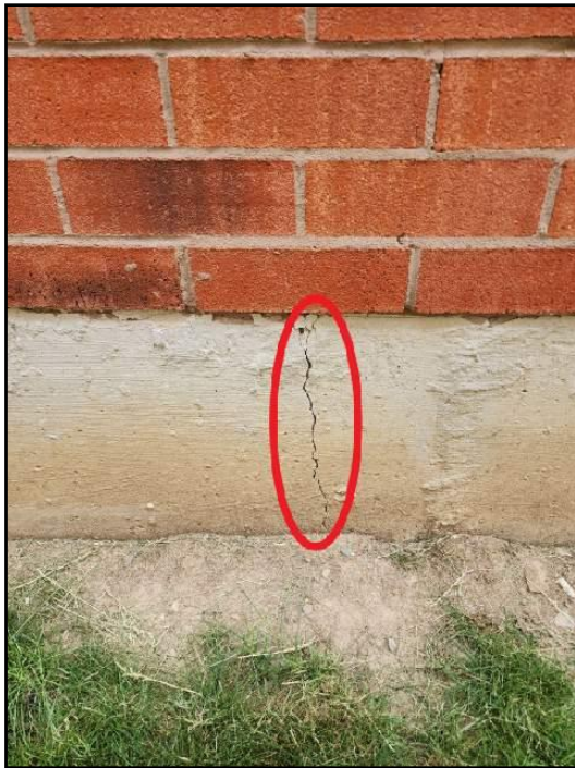
9. Typical minor cracks
