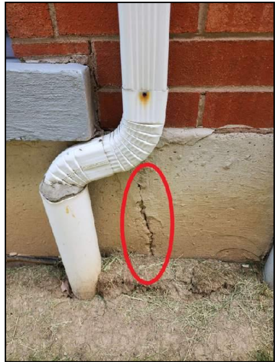
10. Typical minor cracks
