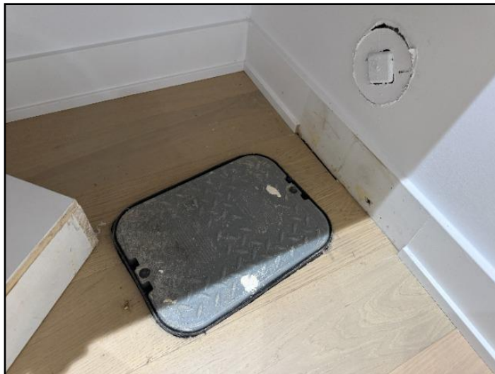
20. Backwater valve is present. These valves...
