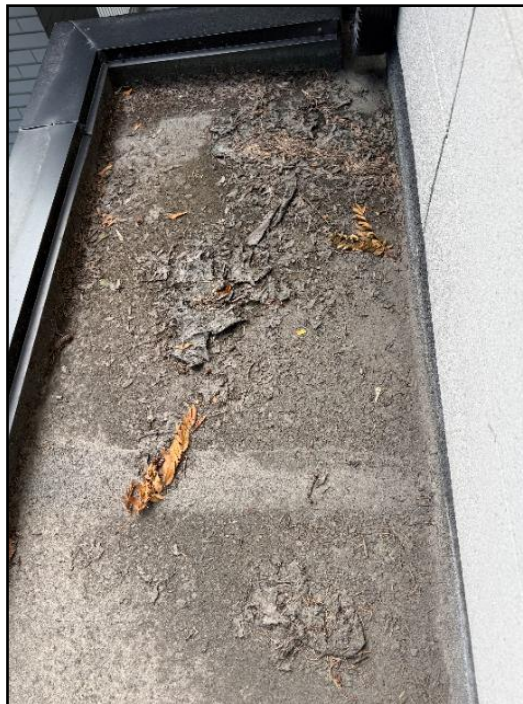
4. Debris on roof
