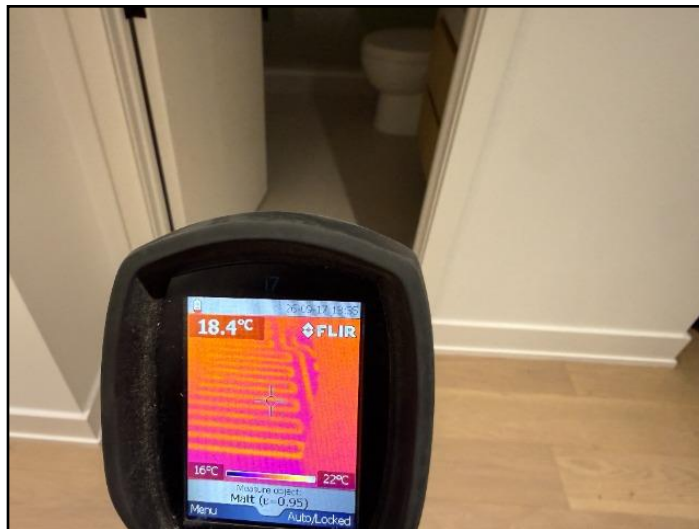
16. one example of bathroom radiant heat
