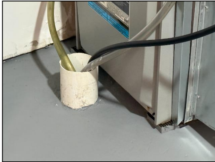
21. Floor drain not flush with floor
