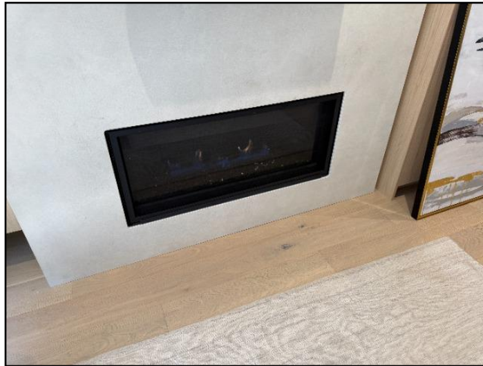
17. Gas fireplace - Functioned when tested
