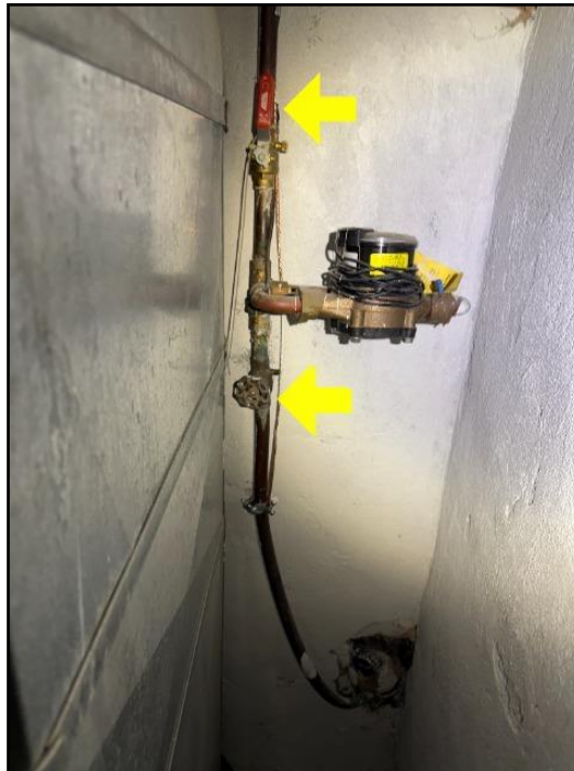
12. Main water shut off valve - Basement
