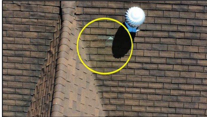
2. Missing, loose or torn
