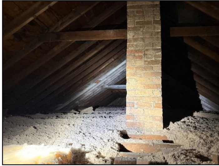
9. Incomplete in attic
