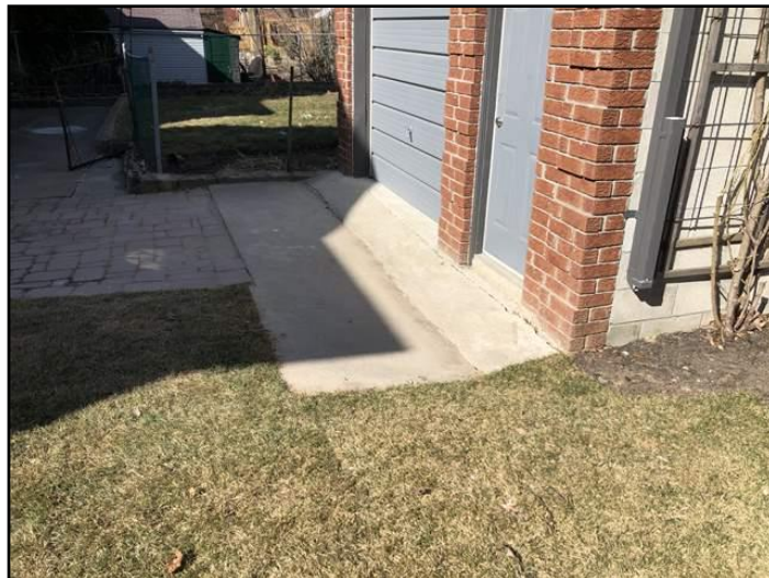
12. Improper slope or drainage
