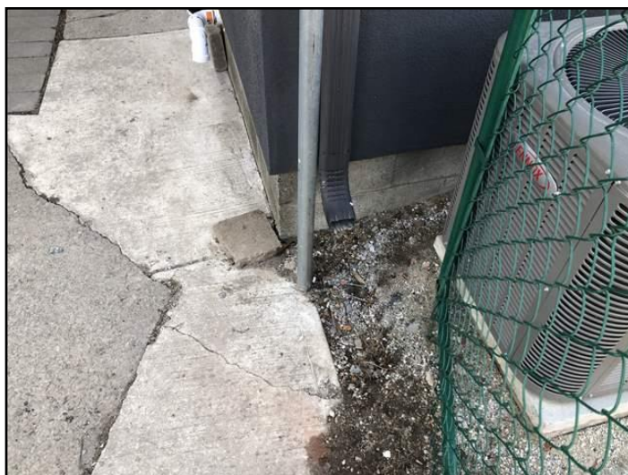
3. Discharge too close to building
