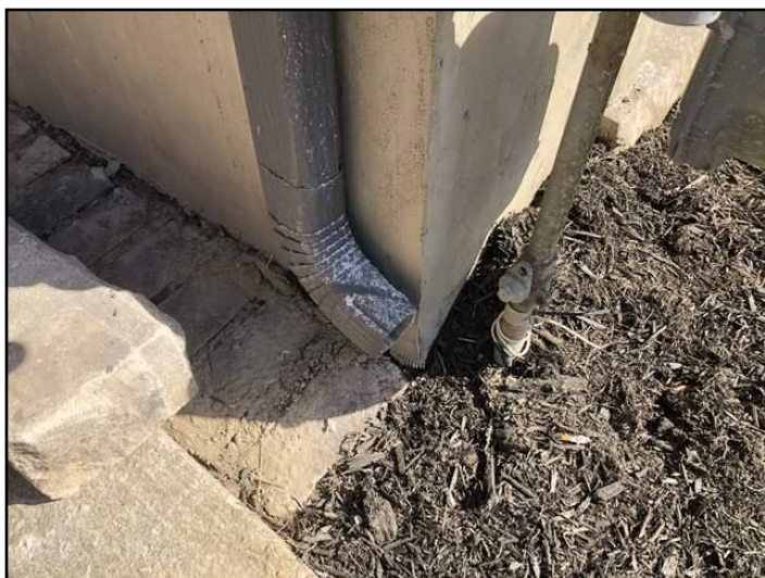
1. Discharge too close to building
