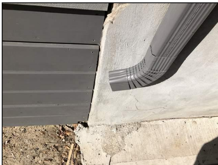
2. Discharge too close to building
