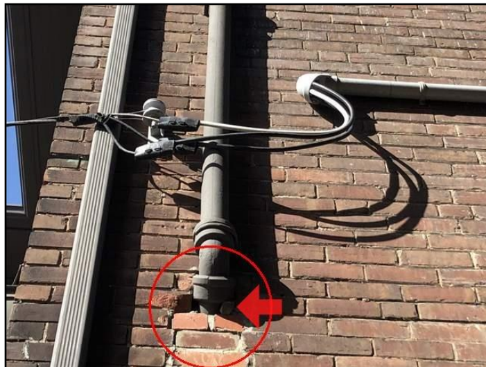
5. Caulking missing or ineffective
