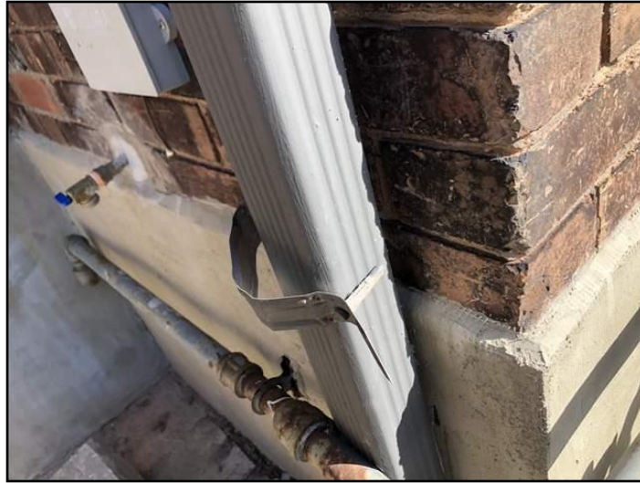
4. Not well secured
