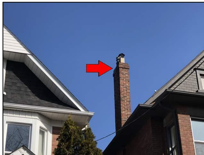
18. No drip edge on cap (crown)
