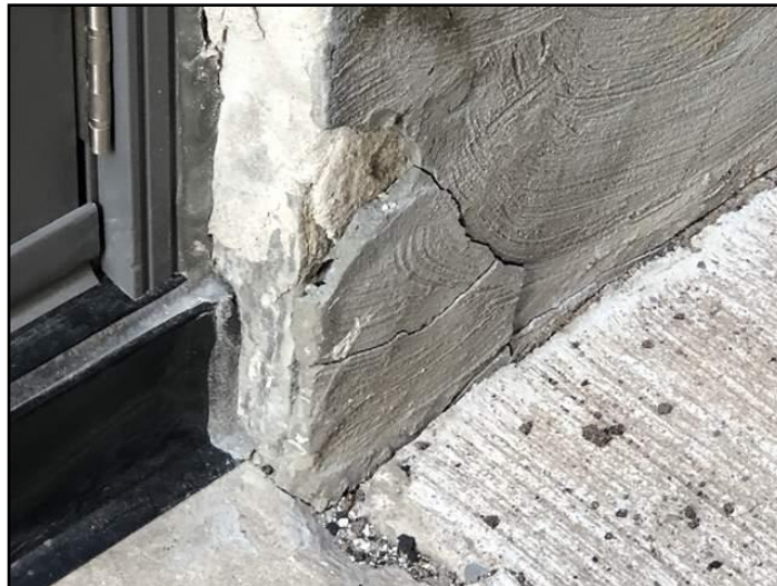
13. Parging damaged or missing
