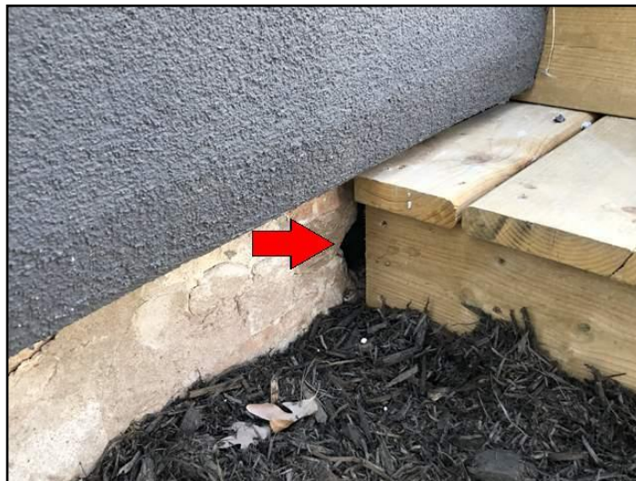
10. Gap at Wall
