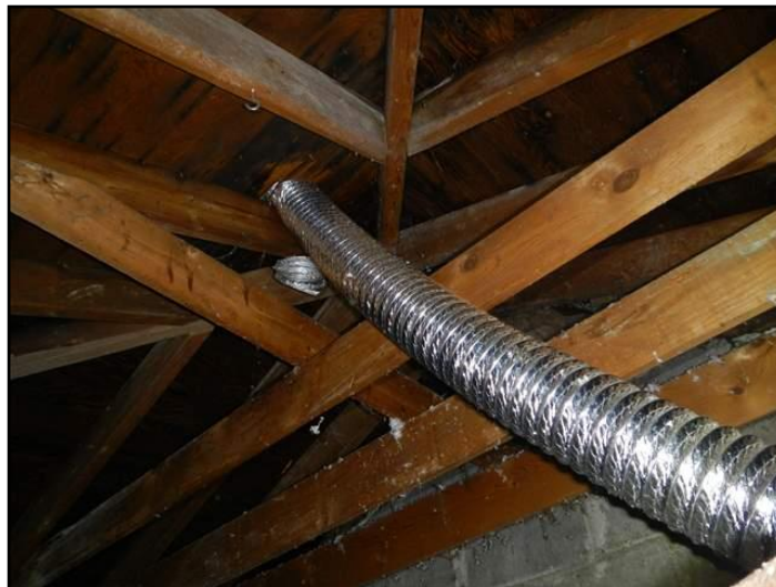
Ductwork not insulated in Attic
