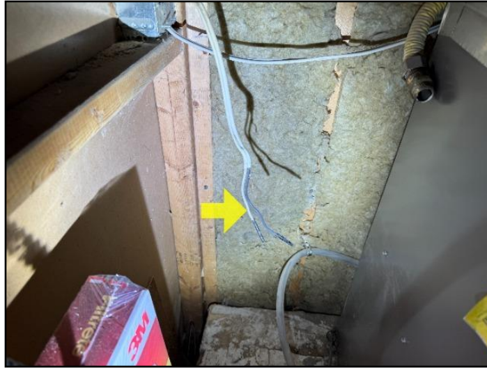
13. Wire not in use
