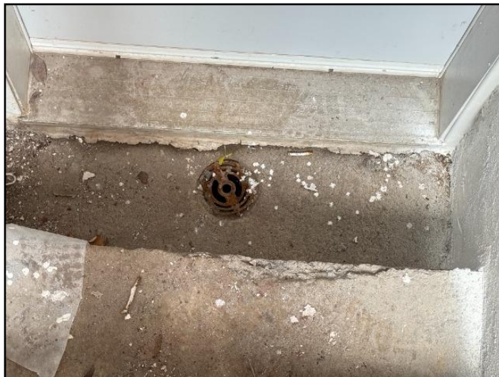
7. Door threshold missing, too low, not...
