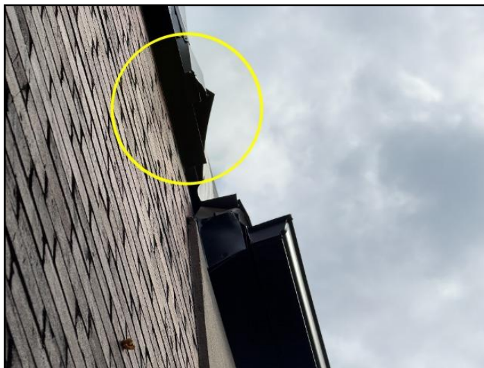
6. Flashings incomplete or ineffective
