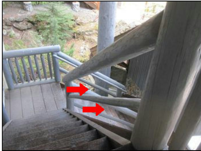
9. Stair guards ineffective for children
