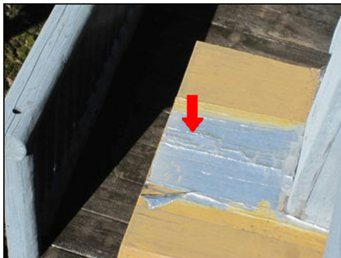
4. Uncapped log end needs flashing
