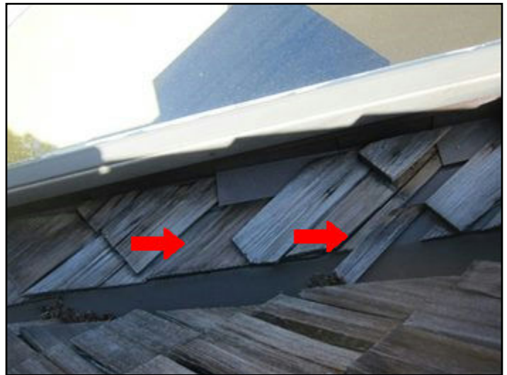
2. Loose and missing pieces
