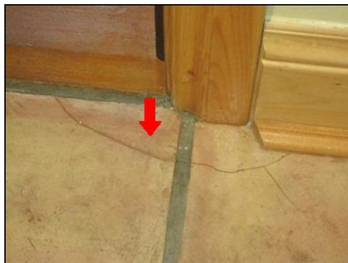
20. Cracked floor tile
