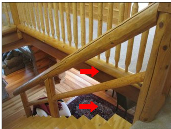
21. Missing stair guard
