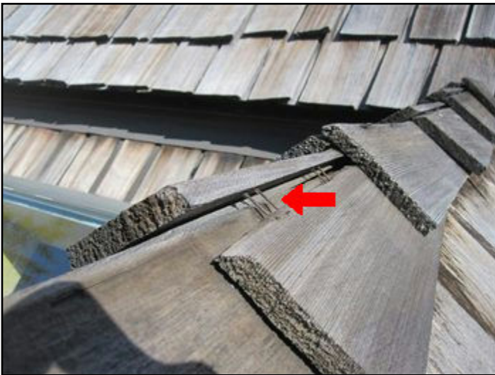
1. Ridge Cap Pulling Away
