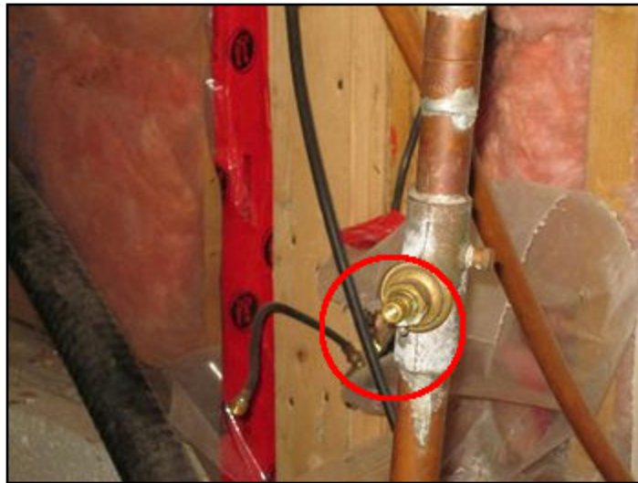
15. Shut off valve handle missing
