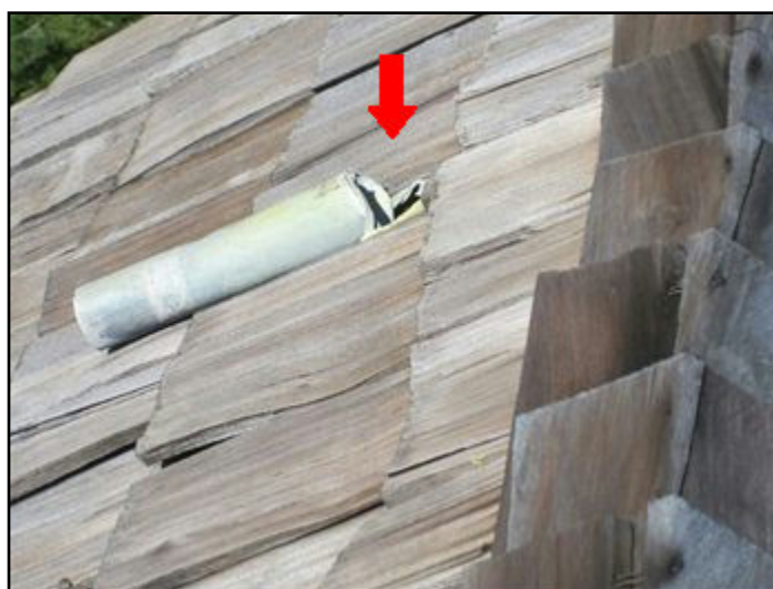
16. Vent pipe torn off roof by snow
