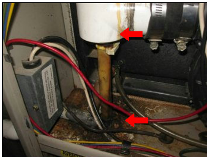
14. Rust, moisture dripping
