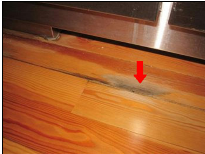
19. Water damaged from refrigerator
