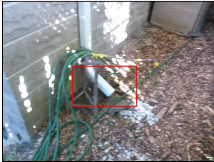
Discharge too close to building
