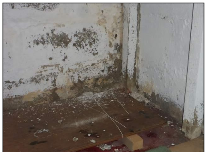
Efflorescence at front basement
