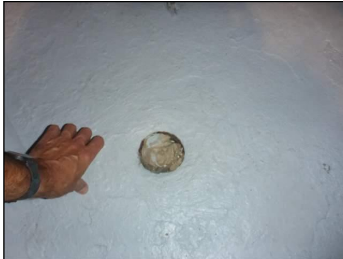
Obstructed- cloth stuffed into floor drain
