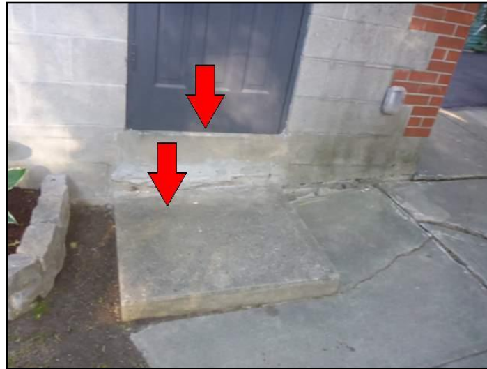
Stair rise too big or not uniform
