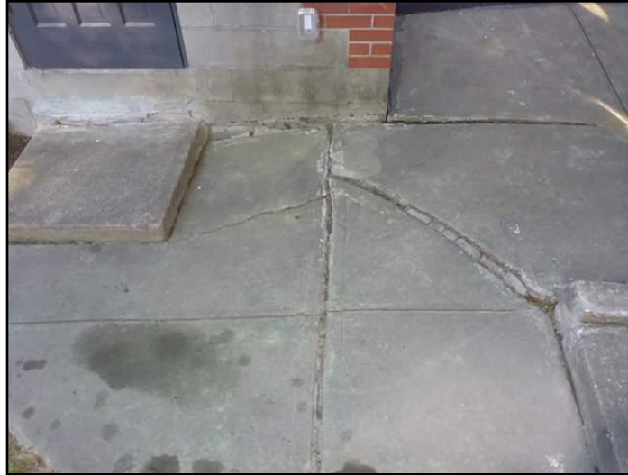
Cracked, settled, uneven
