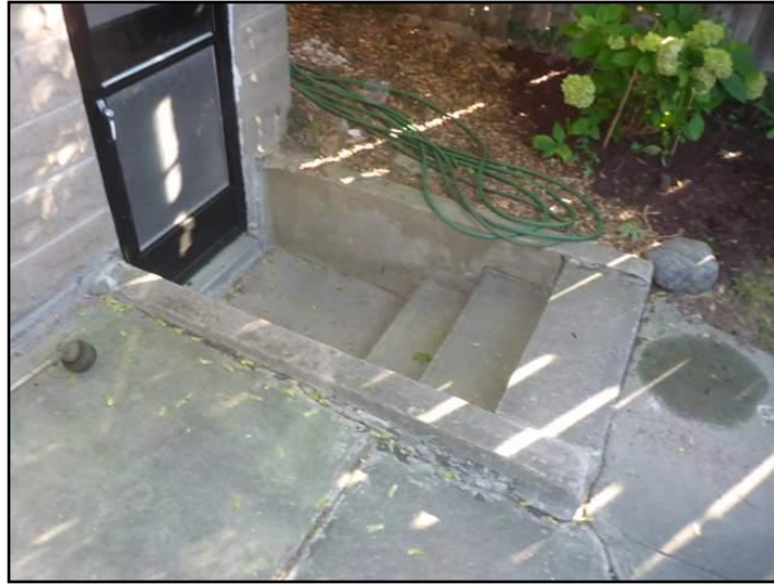
Guard / handrail - missing
