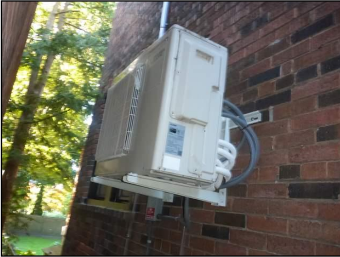
Ductless (Mini split) system- outdoor unit
