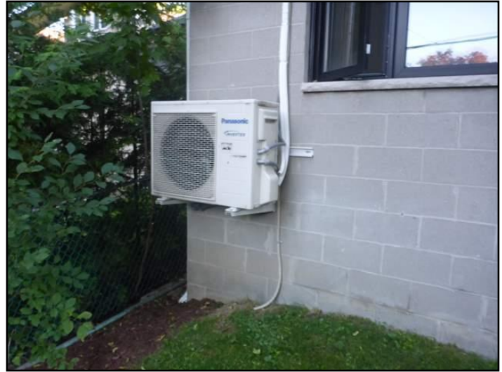
Ductless (Mini split) system- garage
