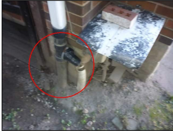
Discharge below grade
