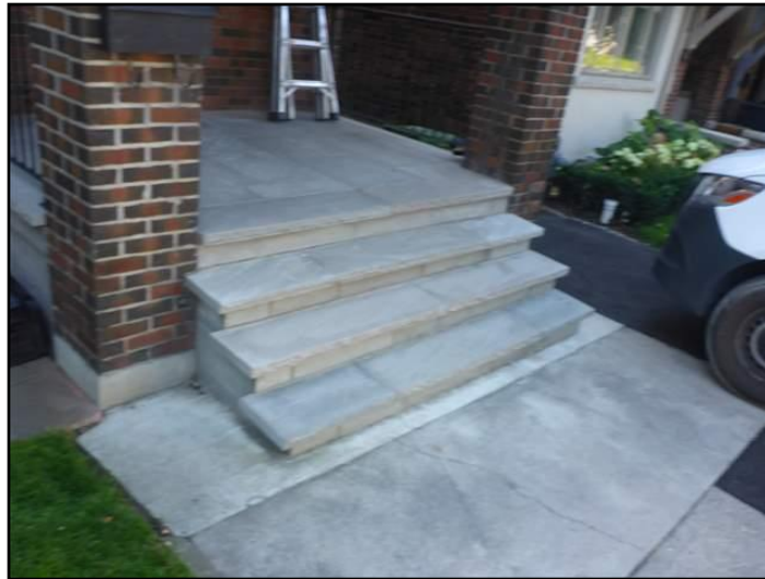
Missing handrail at front steps
