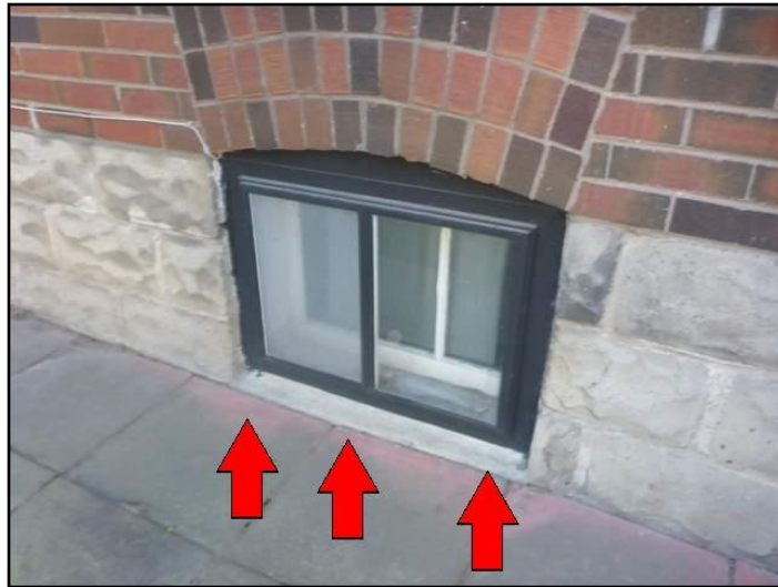
No window well at front basement
