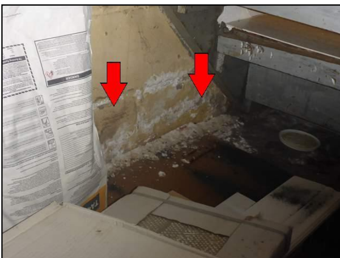
Efflorescence under basement stairs
