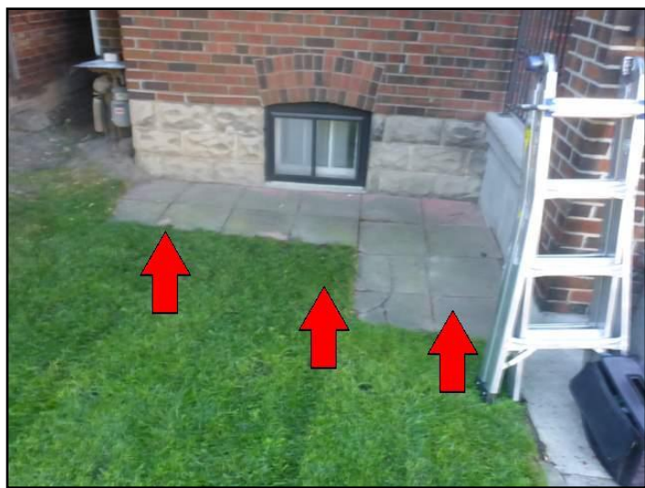
Low area monitor drainage
