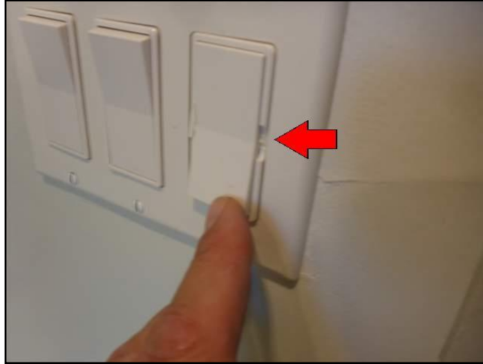
Damaged wall switch (typ.)
