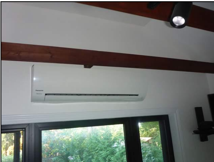
Indoor unit- garage
