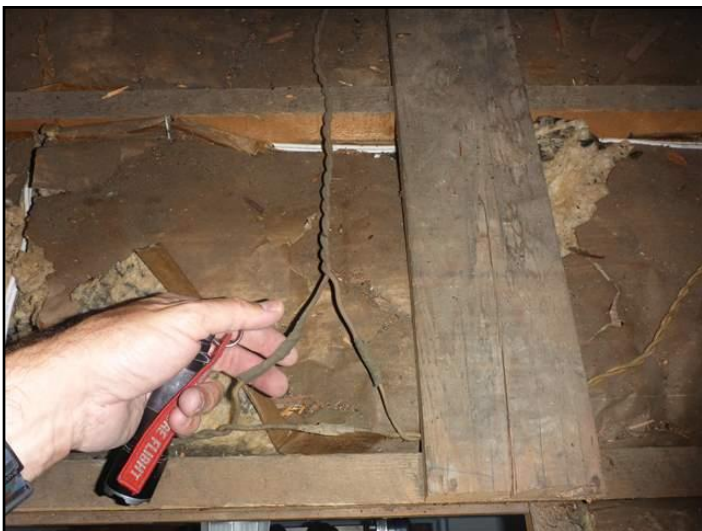
Older abandoned wiring (not K&T)
