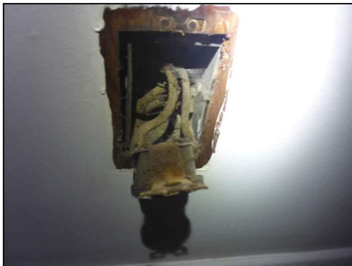
Older abandoned wiring (not K&T)
