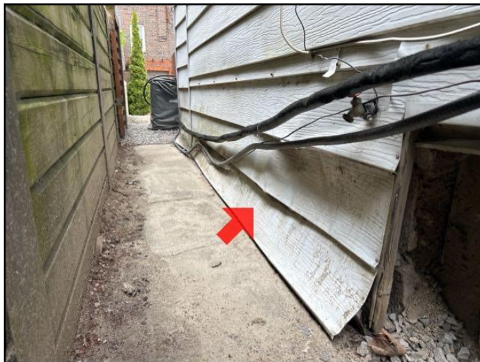
Loose or missing pieces
