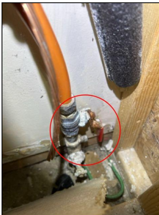
Water shut-off valve
