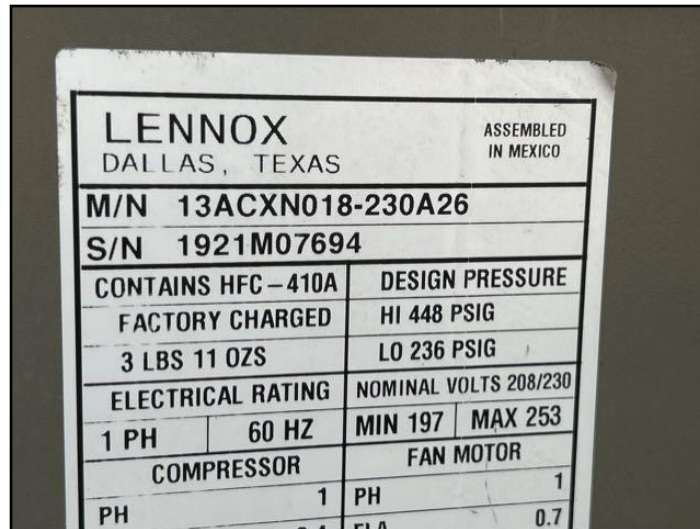
Air conditioner data plate
