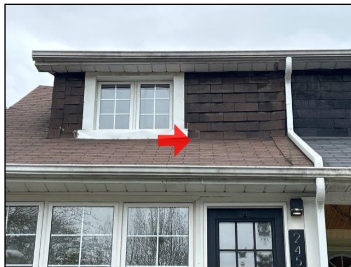
Missing roof-wall flashing
