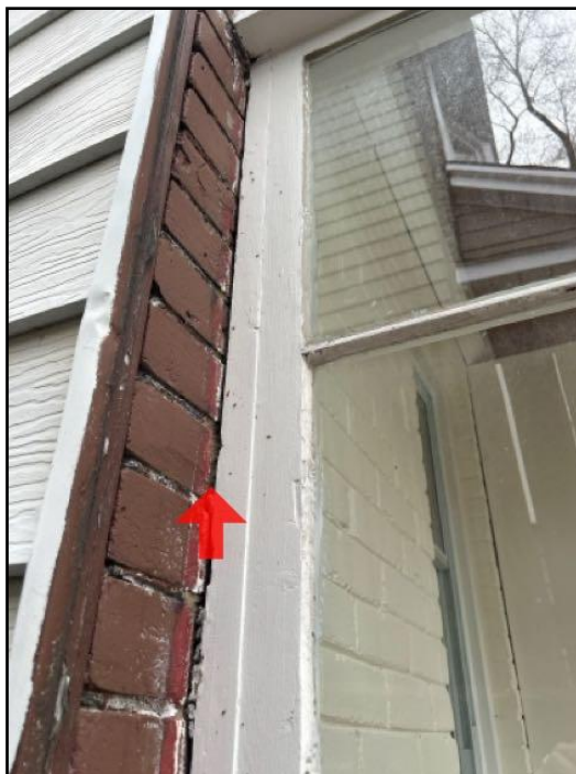
Caulking missing or ineffective
