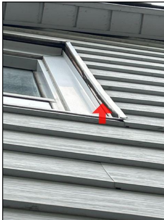
Caulking missing, loose or deteriorated
