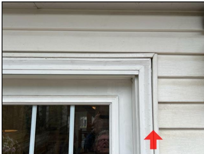
Caulking - deteriorated, loose or missing
