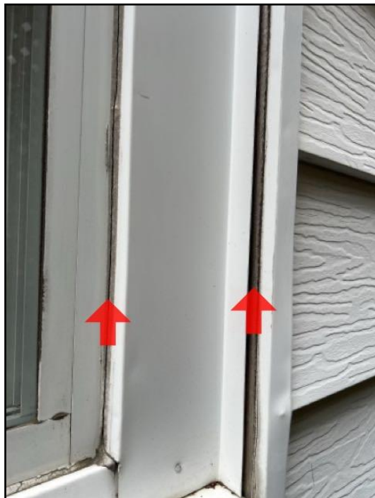
Caulking missing, loose or deteriorated
