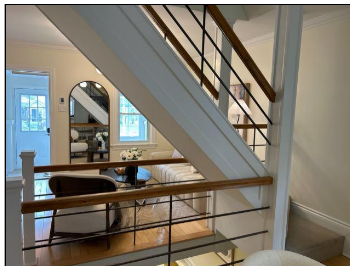
Missing proper spindles
