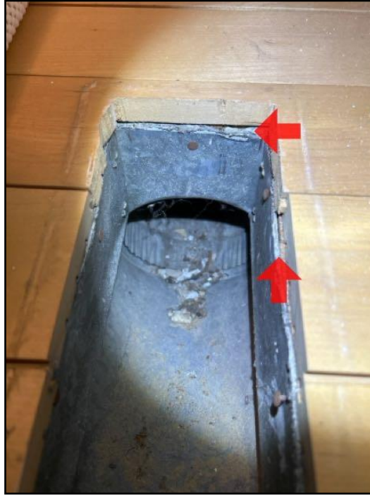
Possible asbestos containing materials
