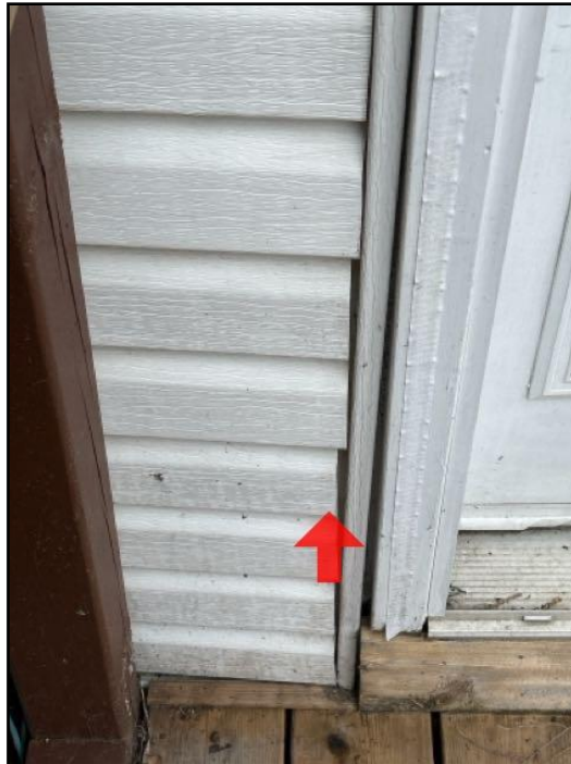
Loose or missing pieces
