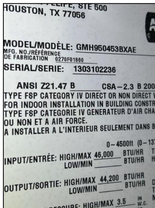
Furnace data plate
